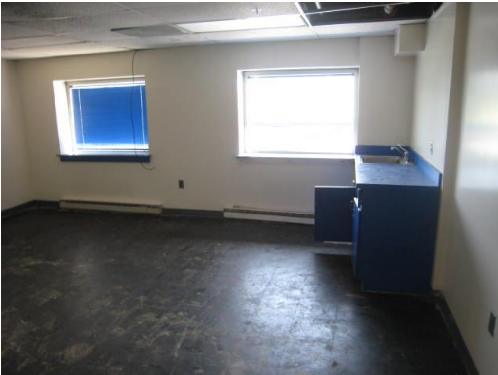
Photo 2: View of Asbestos Remnant Black Floor Tile Mastic Previously Sampled
