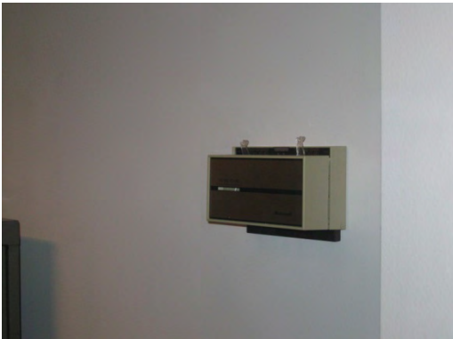
Photograph 6: Thermostat with mercury-containing switches.
