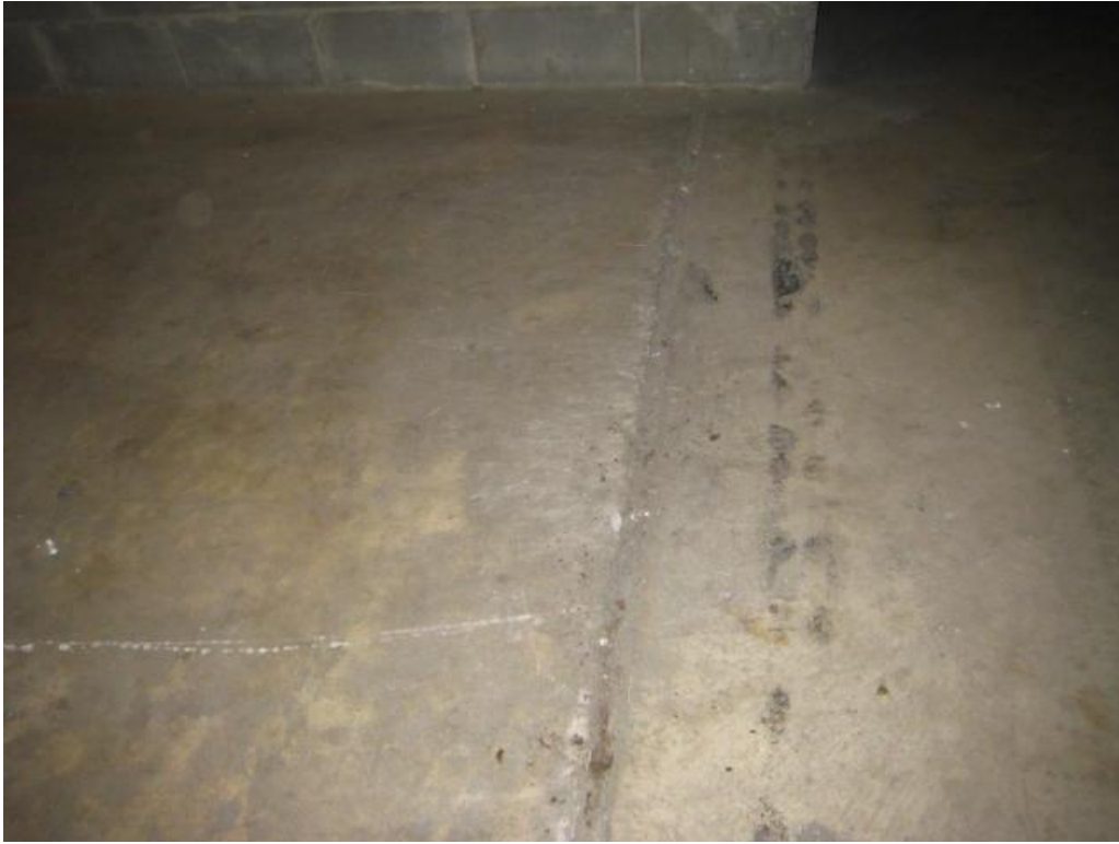
Photo 5 –View of Expansion Joint – Floor Sample 2850-0512-13
