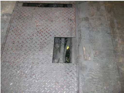
Photograph 8: Piping troughs with standing sludge in main warehouse.
