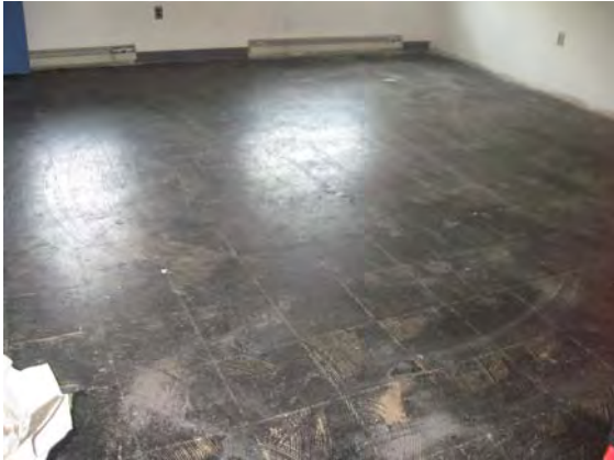
Photograph 1: Asbestos-containing remnant black floor tile mastic
