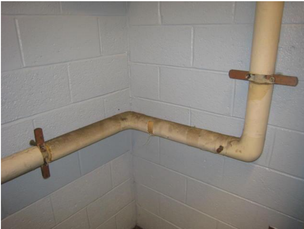
Photo 8 –View of Paper Covering Over Fiberglass Pipe Insulation Sample 2850-0512-22
