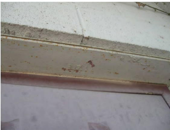
Photograph 3: Metal window lintel with lead-based paint.
