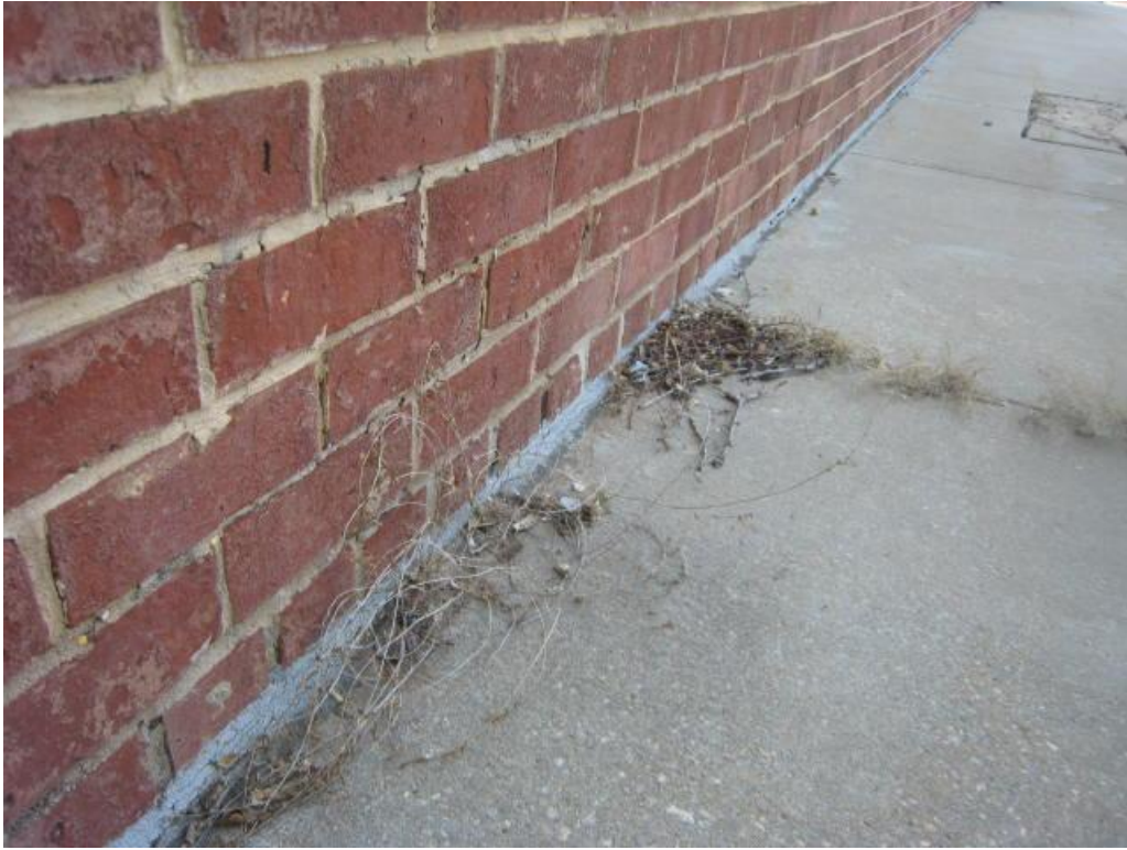
Photo 1 –View of Asbestos Expansion Joint Caulk Previously Sampled
