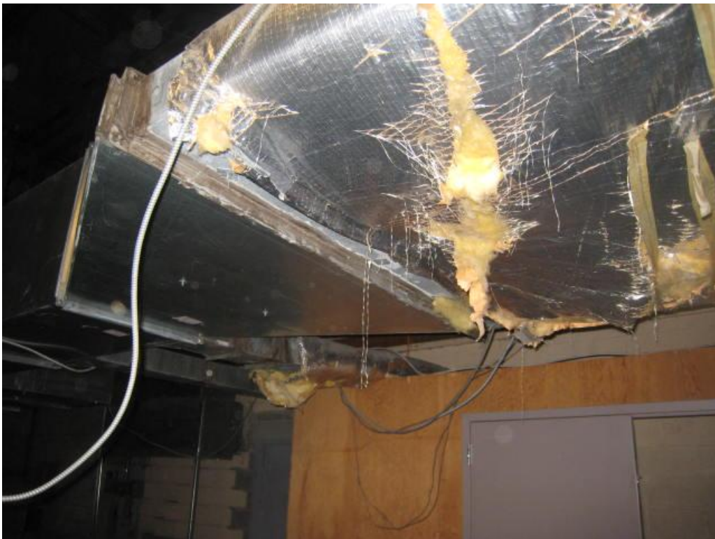
Photo 6 –View of Paper Covering Over Fiberglass Duct Insulation Sample 2850-0512-16
