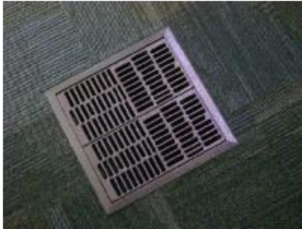
Underfloor air distribution vent
