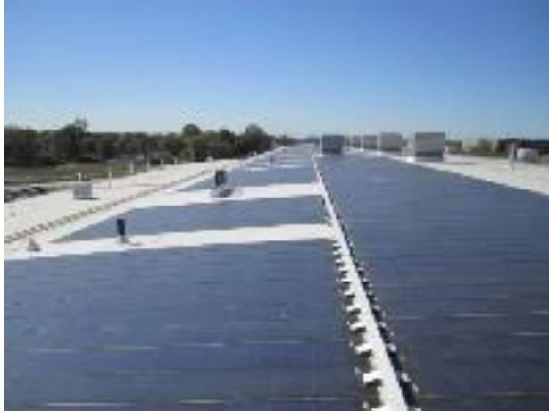
Photovoltaic panels on roof
