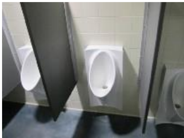
Low-flow and automatic fixtures
