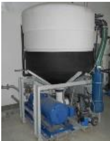
Wash water reclaim system
