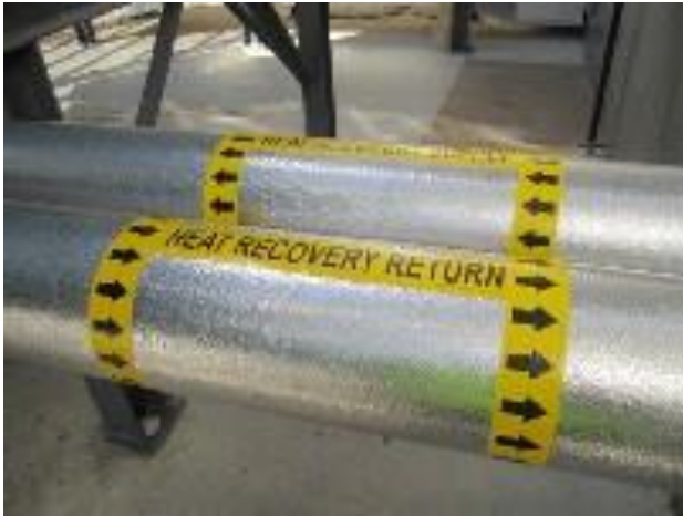
Heat recovery piping
