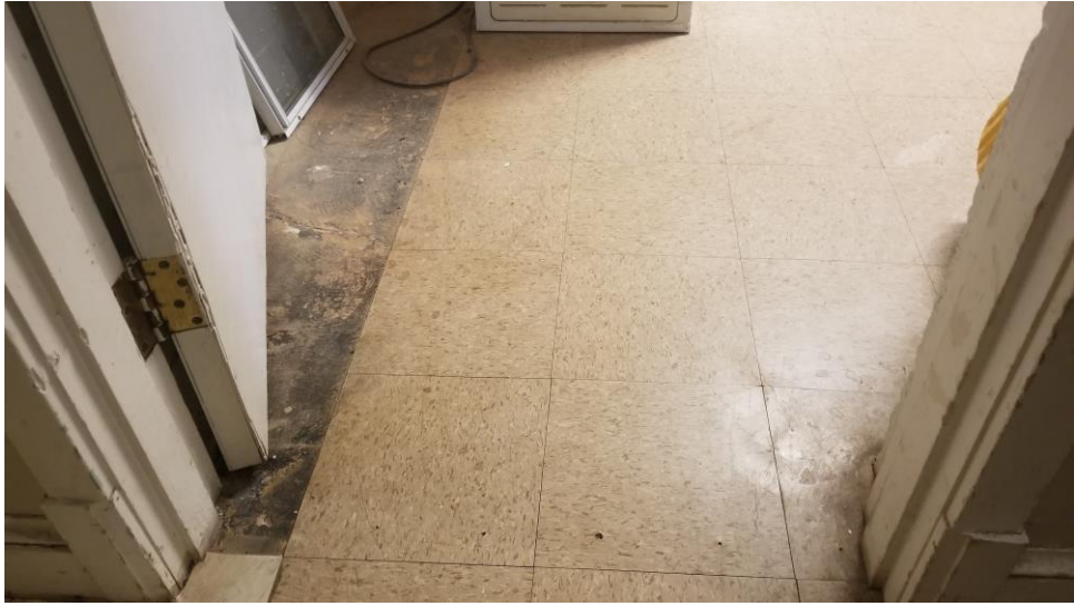
Asbestos below floor tile in basement
