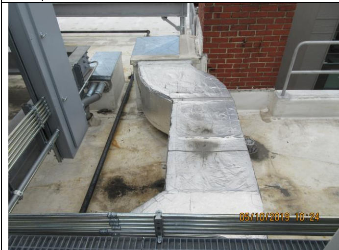
Description: roof level ducts exposed to elements.
