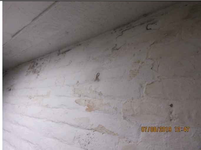
Description: basement exterior walls effervescing.
