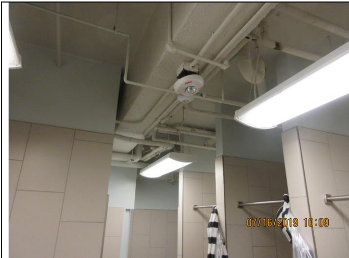
Description: no ceilings in the gang shower rooms.
