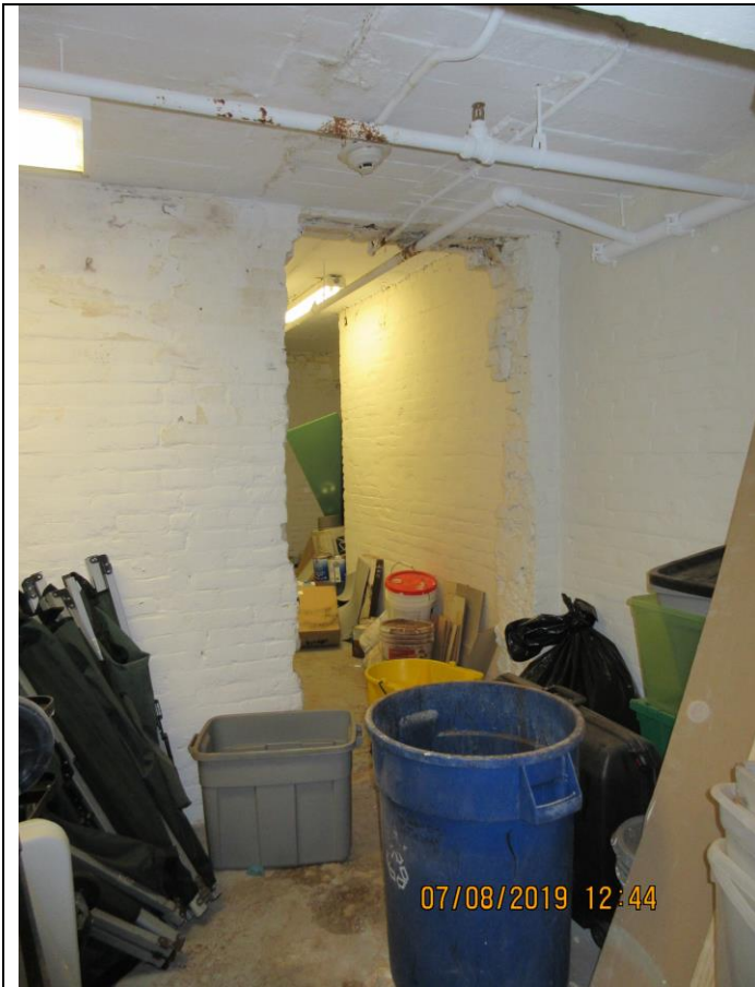
Description: water intrusion at basement ceiling
