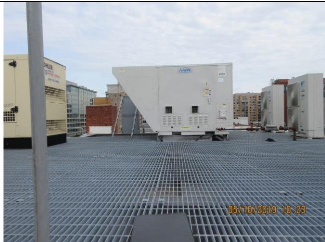
Description: DOAS unit above roof line
