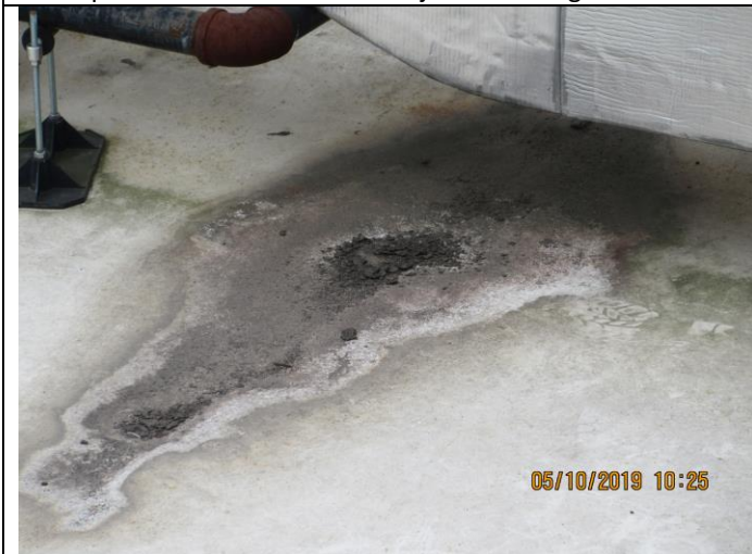
Description: water collected under ducts.
