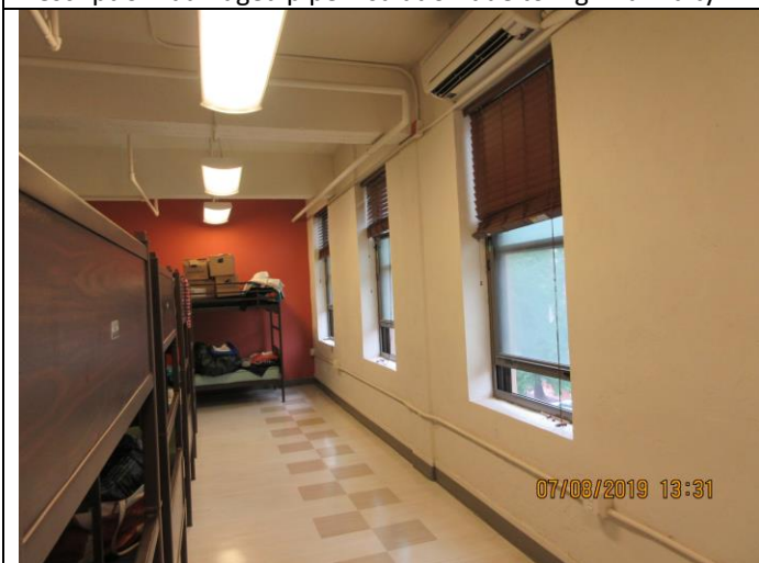
Description: view of a dorm room with a fan coil unit.
