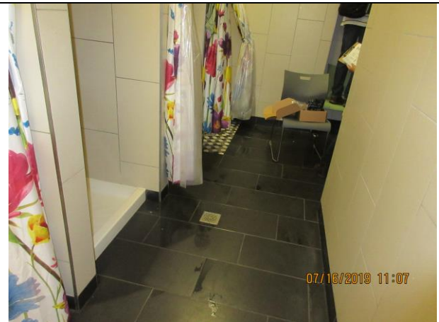
Description: No slope in the floor to allow water to flow to the drains.
