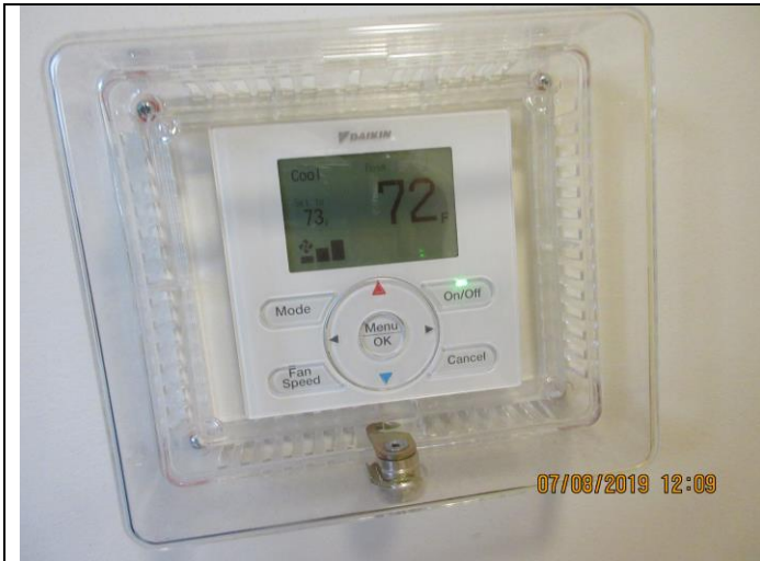
Description: T-Stat set at 73°F with room temp at 72°F.
