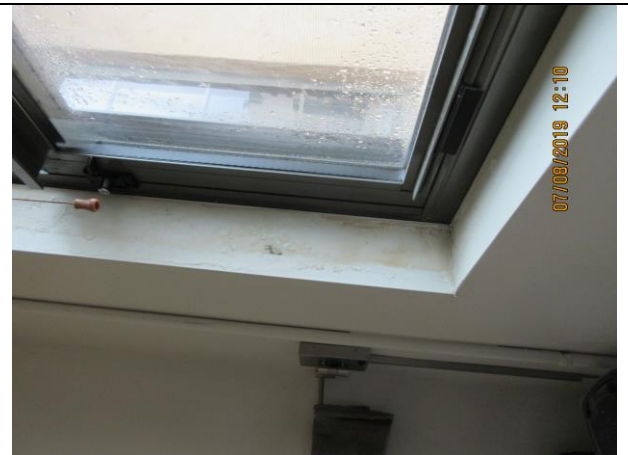
Description: damage to window sill from water intrusion.
