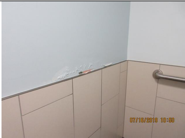
Description: Damaged wall from leaking fan coil above.
