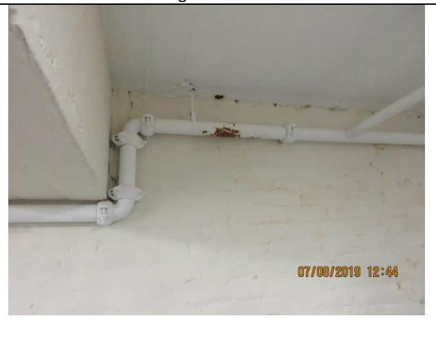
Description: water leak from basement ceiling and damaged pipe.
