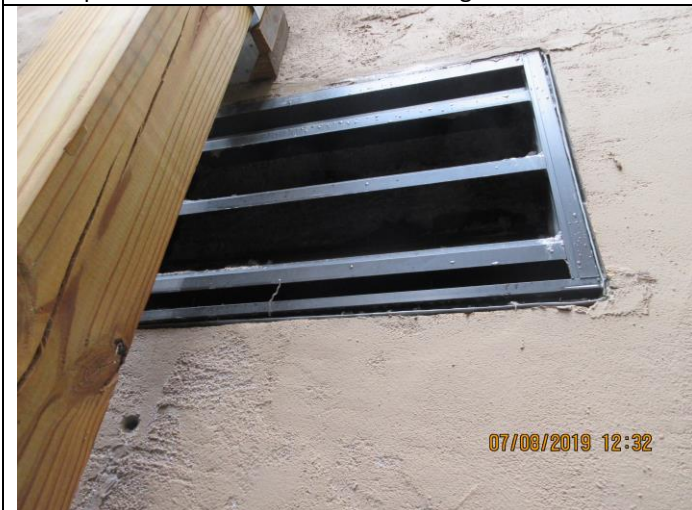
Description: exterior louver frame missing caulk.
