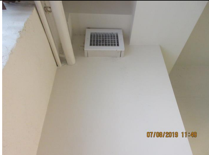
Description: a typical fresh-air supply air outlet
