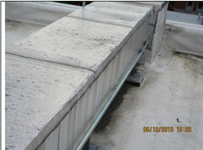
Description: ductwork on roof subject to damage.
