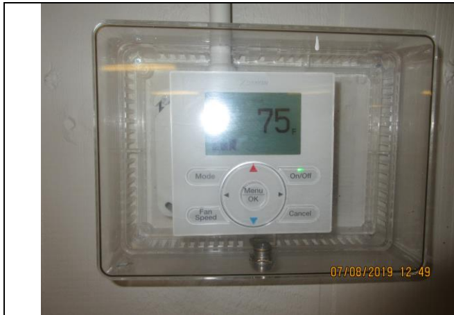
Description: T-Stat is set to 73°F with room temp at 75°F.
