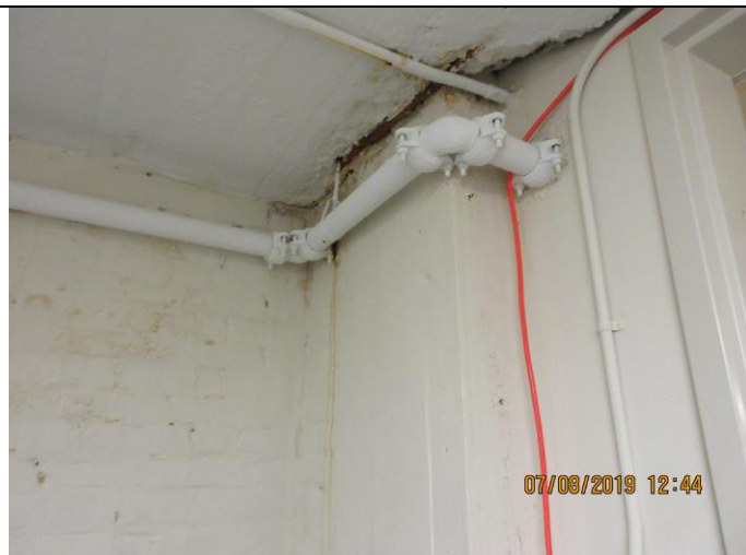
Description: water intrusion in basement.
