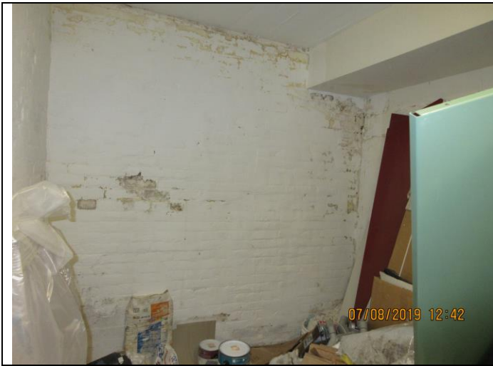
Description: basement exterior walls effervescing.
