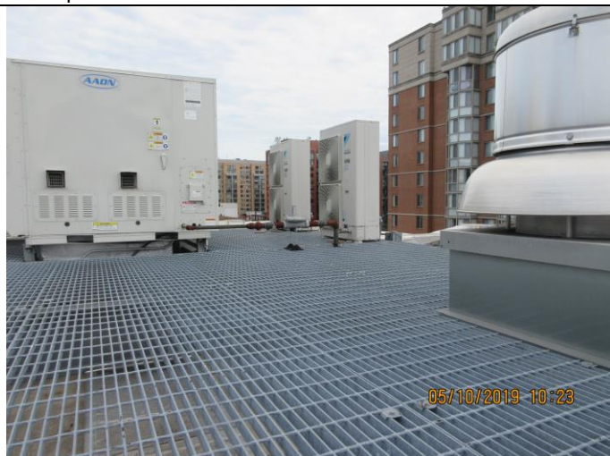
Description: Condensing units above roof line
