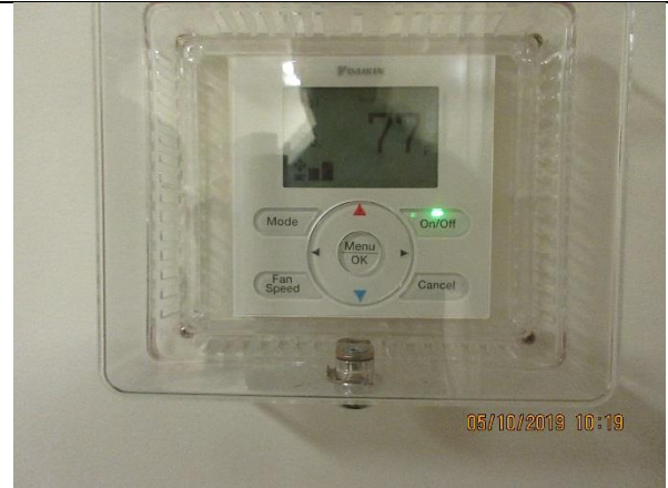
Description: Bathroom thermostat set to 73°F with room temp at 77°F.
