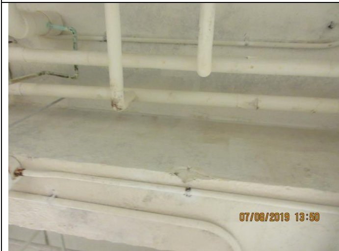
Description: damaged pipe insulation due to high humidity.
