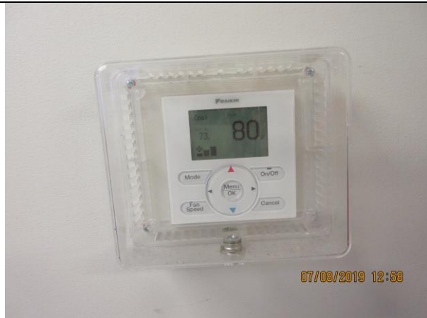
Description: T-Stat is set to 73 with room temp at 80°F.
