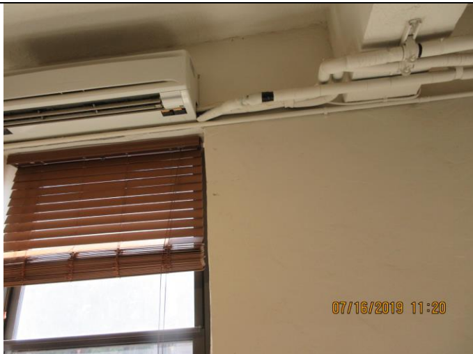
Description: Typical fan coil serving dorm rooms.
