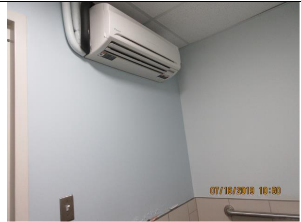
Description: Fan coil's drain pan is clogged and condensate is overflowing.
