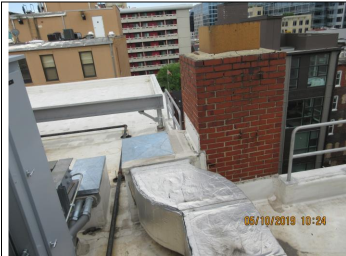
Description: roof level ducts exposed to elements.
