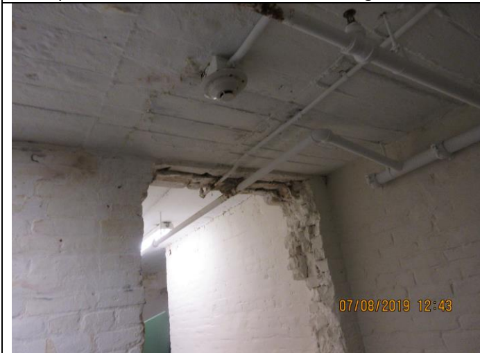
Description: water intrusion at basement ceiling
