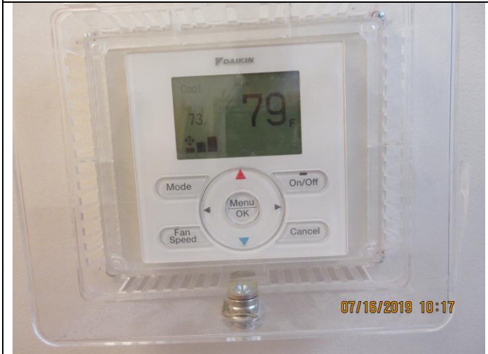
Description: T-Stat set to 73°F with room temp at 79°F.
