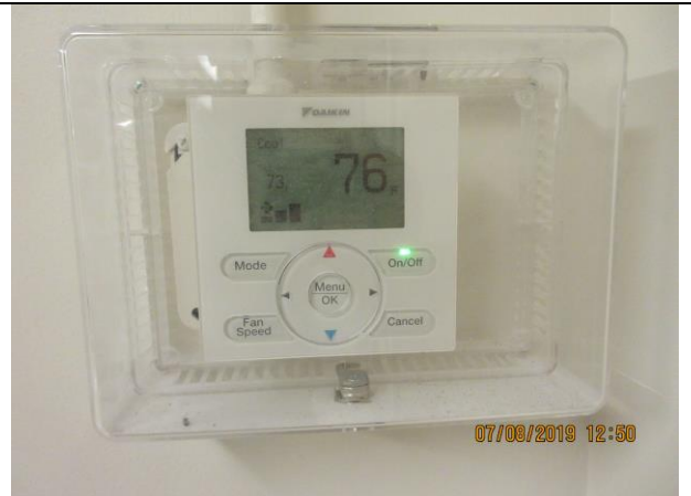
Description: T-Stat is set to 73°F with room temp at 76°F.
