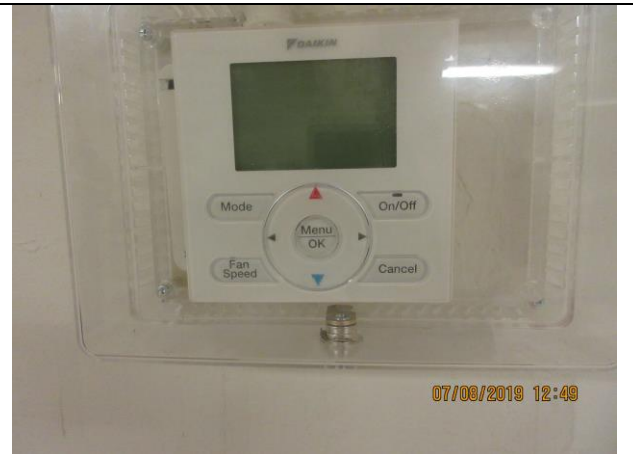
Description: T-Stat is turned off.
