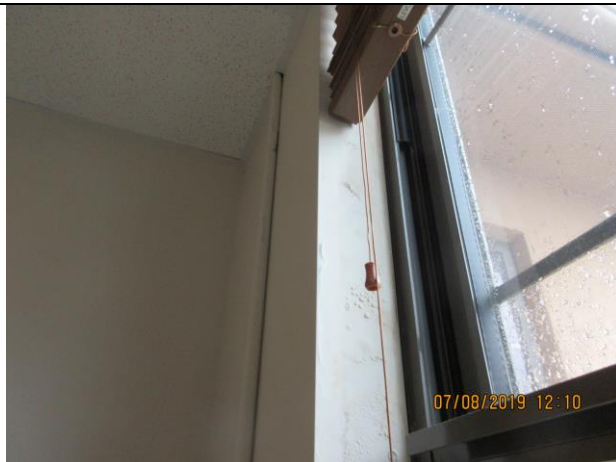
Description: damaged window frame from water intrusion.
