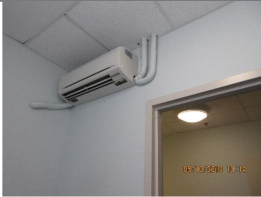
Description: A typical Fan Coil unit serving single bathrooms.
