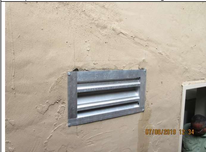
Description: exterior louver frame missing caulk.
