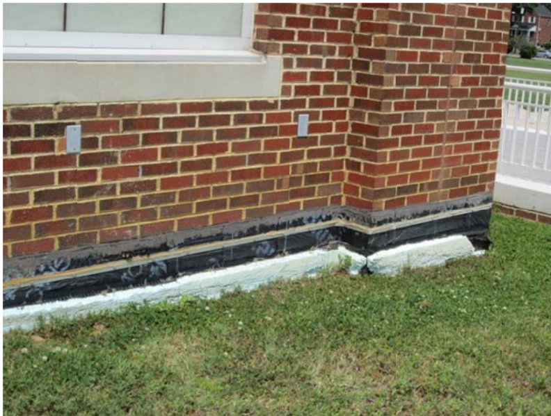
Photograph 4-8.11 (Aquatic Center) Exposed and damaged water barrier and insulation at foundation along exterior of building.
