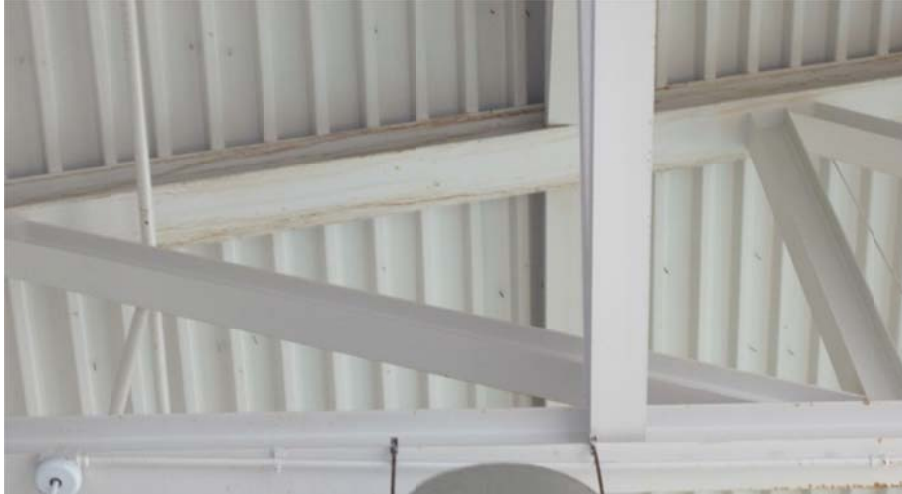
Photograph 4-8.19 (Aquatic Center) Water damage and rust along roof beams and truss over pool.
