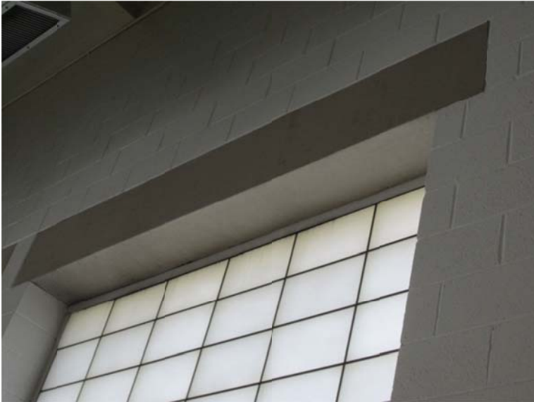
Photograph 4-8.17 (Aquatic Center) Water marks along high windows in pool area.
