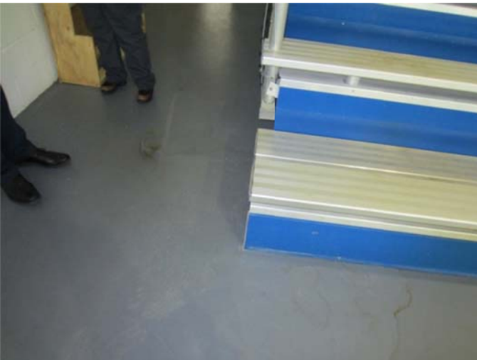
Photograph 4-8.18 (Aquatic Center) Water damage on floor on pool observation deck from apparent roof leak.
