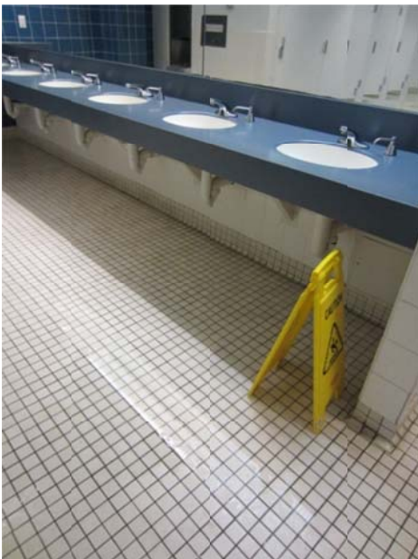
Photograph 4-8.15 (Aquatic Center) Puddle of water in Women's Locker Room from leak into wall near shower area.
