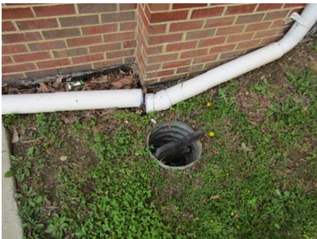
Photograph 4-8.9 (Aquatic Center) Detached rain leader and opened and clogged drain.
