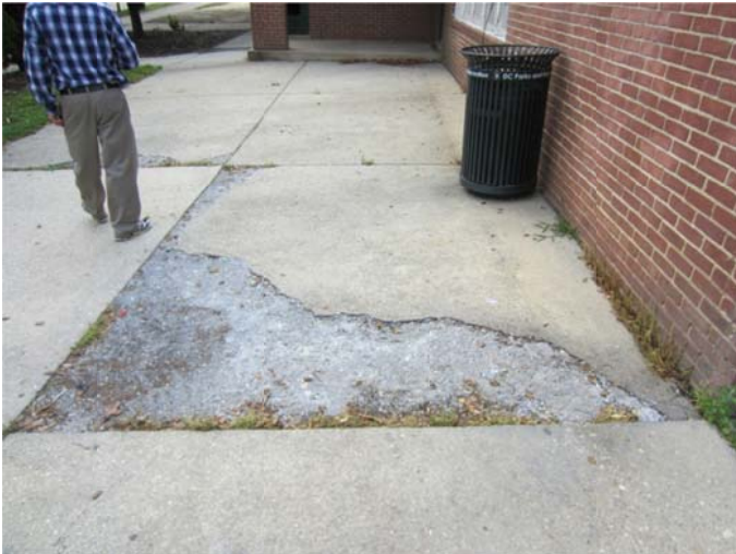
Photograph 4-8.22 (Field House) Damaged exterior paving.
