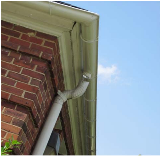
Photograph 4-8.4 (Community Center) Detached roof drain from gutter.
