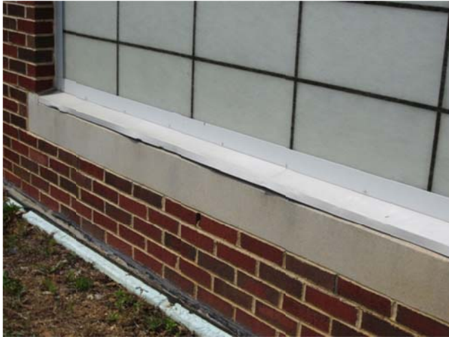
Photograph 4-8.10 (Aquatic Center) Damaged flashing at base of window, exposed insulation at foundation below.
