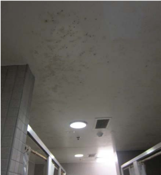
Photograph 4-8.14 (Aquatic Center) Mold growing along ceiling and walls in shower area of Women's Locker Room.
