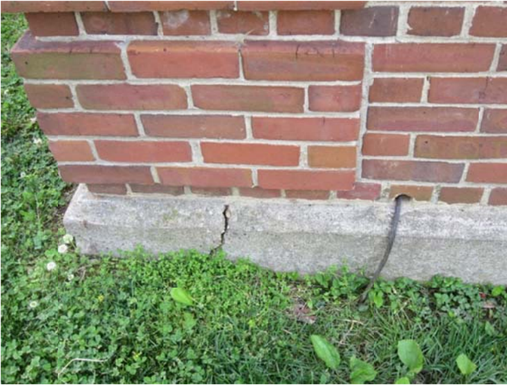
Photograph 4-8.1 (Community Center) Damaged foundation at building corner, anchoring in place.
