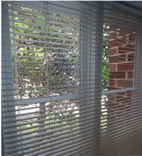
Photograph 4-8.7 (Community Center) Broken Glass.
