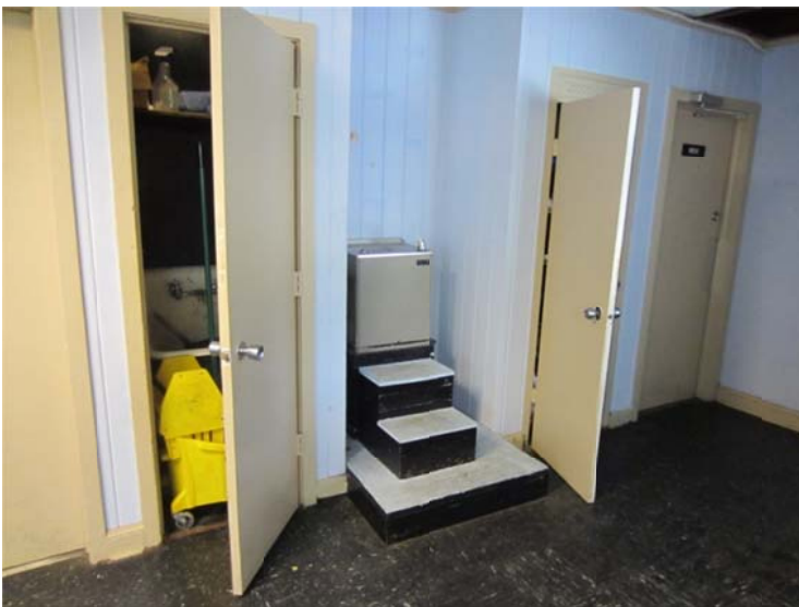
Photograph 4-8.23 (Field House) Non-ADA accessible fixtures.
