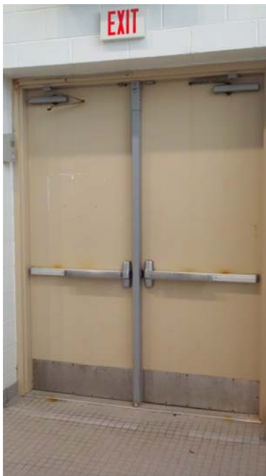
Photograph 4-8.8 (Aquatic Center) Damaged egress door.
