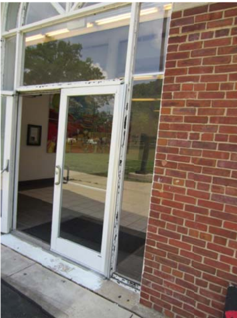
Photograph 4-8.2 (Community Center) Rusted and chipped entry door.
