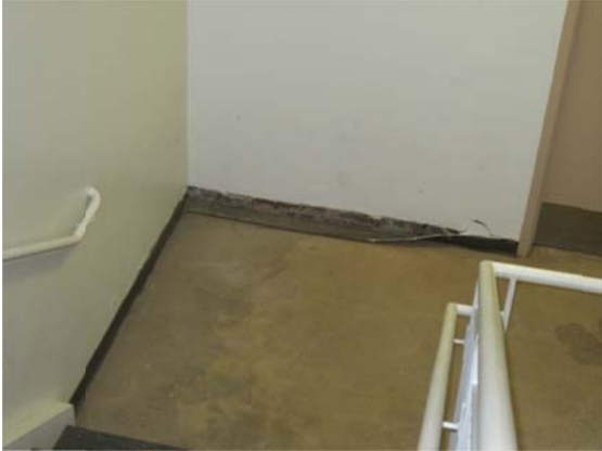
Photograph 4-8.13 (Aquatic Center) Loose base trim in stairwell.
