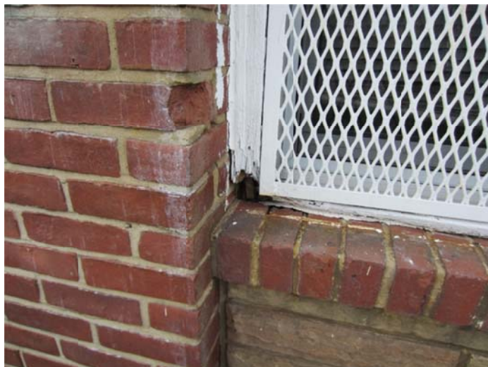
Photograph 4-8.21 (Field House) Damaged wooden exterior window sill.
