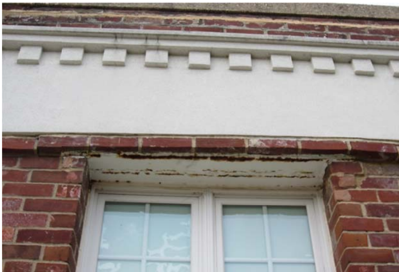
Photograph 4-8.6 (Community Center) Rusted and damaged window head.
