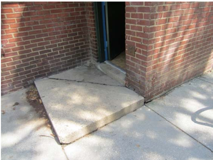
Photograph 4-8.24 (Field House) Damaged exterior landing at restrooms. Not ADA accessible.
