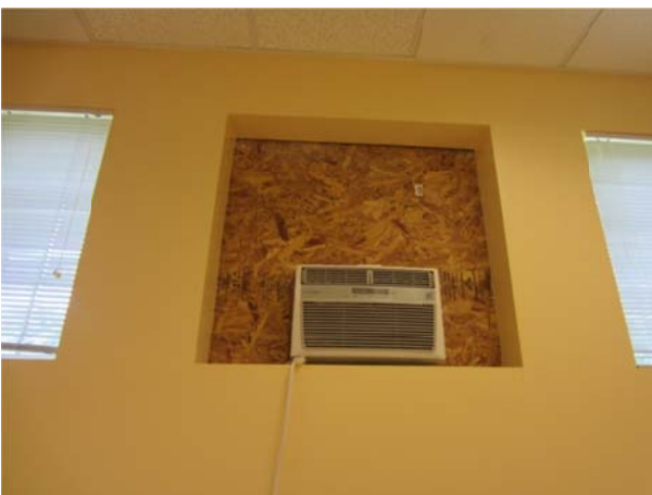
Photograph 4-8.3 (Community Center) Boarded up window with AC unit.
