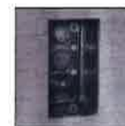
TA-62F Empty Junction Box
