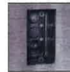
TA-62F Empty Junction Box
