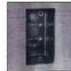
TA-62F Empty Junction Box
