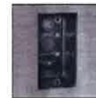
TA-62F Empty Junction Box
