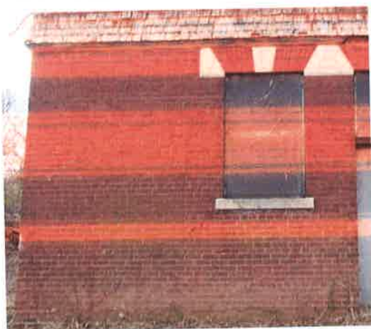
Photo 5 Step crack at north elevation
