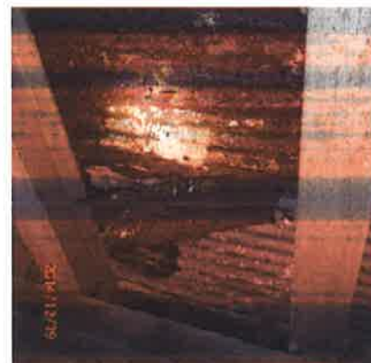
Photo 24 – Deteriorated metal deck and beams at basement slab framing
