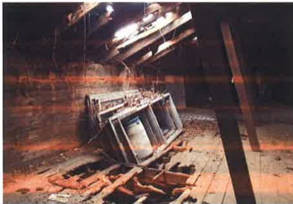
Photo 21 - Typical infiltration of water at the roof, leading to damaged roof framing and second floor framing
