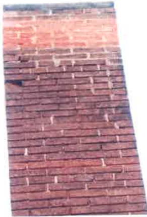
Photo 13 – Past repairs & deterioration at the south chimney
