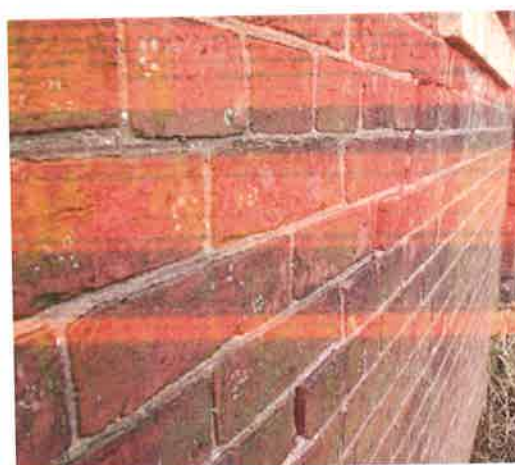
Photo 6 – Out-of-plane displacement at step crack
