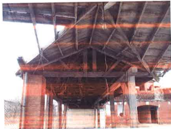
Photo 16 – Failed framing over entry at front storage area
