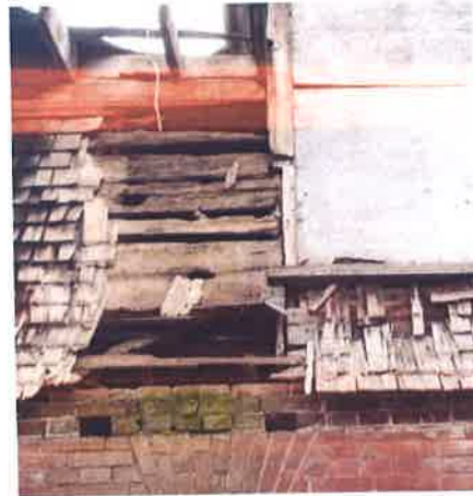
Photo 14 – Loss of roofing and siding leading to deterioration of brick and biological growth
