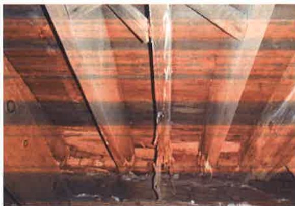
Photo 23 – Failing floor joists at basement slab framing
