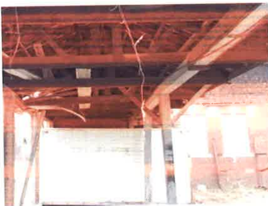
Photo 17 – Missing support posts at front storage area
