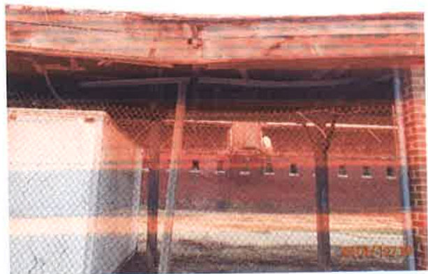
Photo 18 – Failed support beam at front storage area
