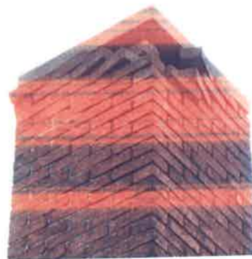
Photo 12 – Displaced bricks at north chimney
