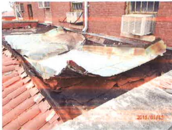
Photo 4. Area 2: Loss of roofing and waterproofing membrane
