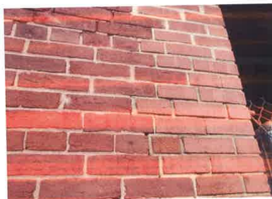
Photo 4 – Past repairs at west elevation (North wing)
