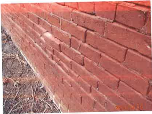
Photo 7 – Typical loose brick courses, east elevation
