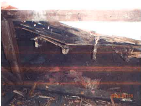
Photo 1. Area 1: Failure of wood frame
