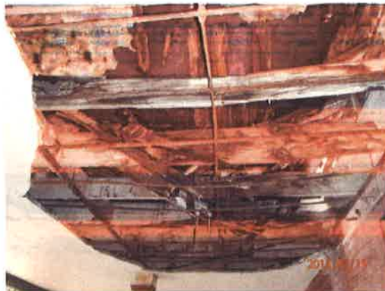
Photo 6. Area 2: Deterioration and failure of rafters
