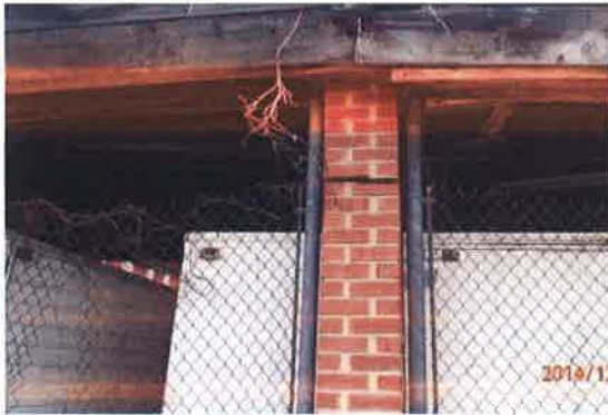
Photo 19 – Damaged brick pier at front storage area
