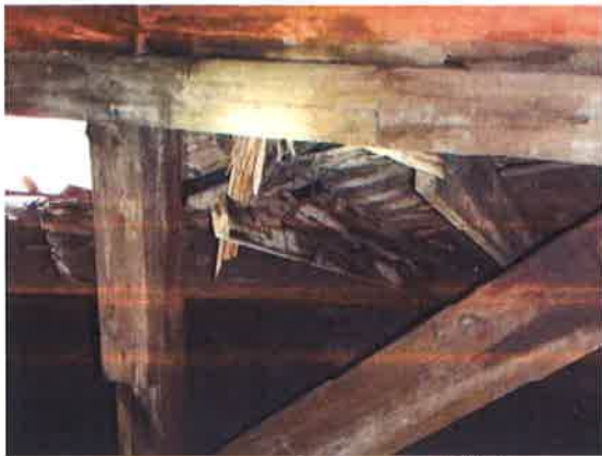
Photo 2. Area 1: Deterioration of rafters and decking
