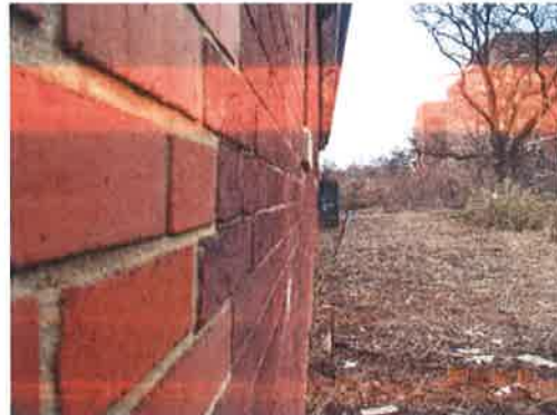
Photo 20 – Leaning brick bearing wall at front storage area
