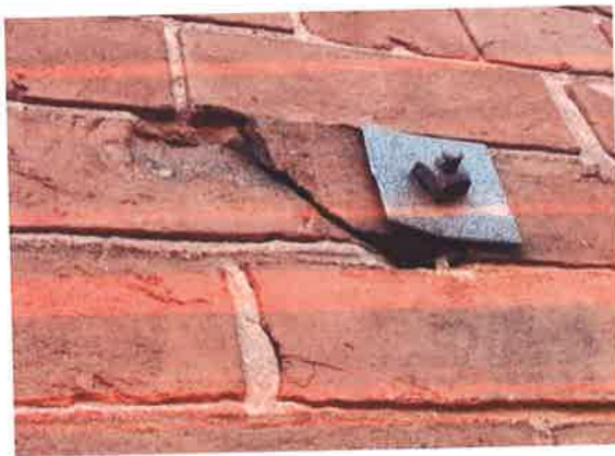
Photo 9 – Brick spalling due to corrosion of embedded steel
