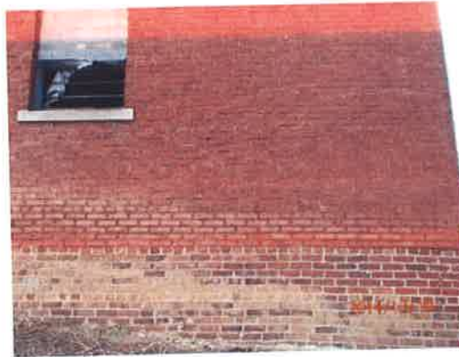
Photo 8 – Past repairs of lower brick courses, south elevation
