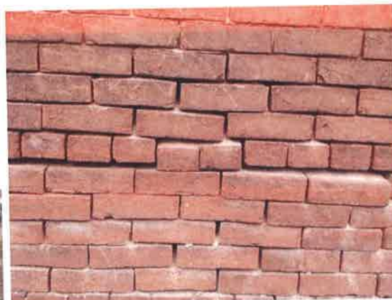
Photo 2 – Typical mortar loss in brick joints
