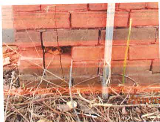
Photo 11 – Missing brick near central entry door
