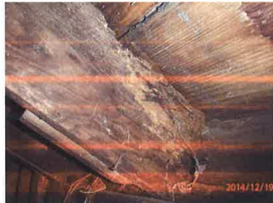
Photo 22 - Typical wood deterioration at roof rafter bearing due to water
