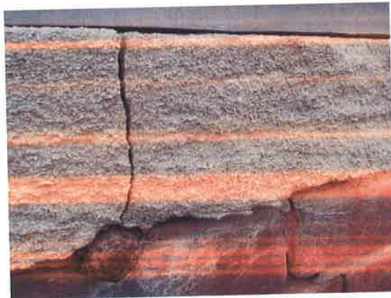
Photo 10 – Cracked limestone sill due to corrosion of embedded steel
