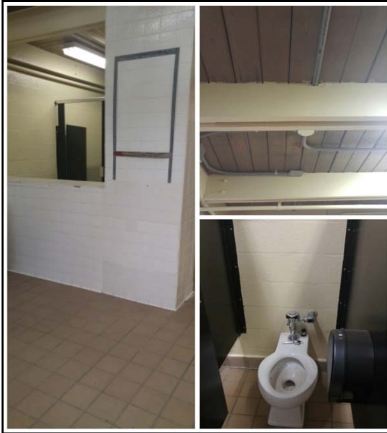
Lead-based paint and surfaces
