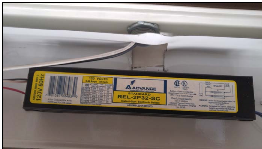
Non-PCB containing ballasts
