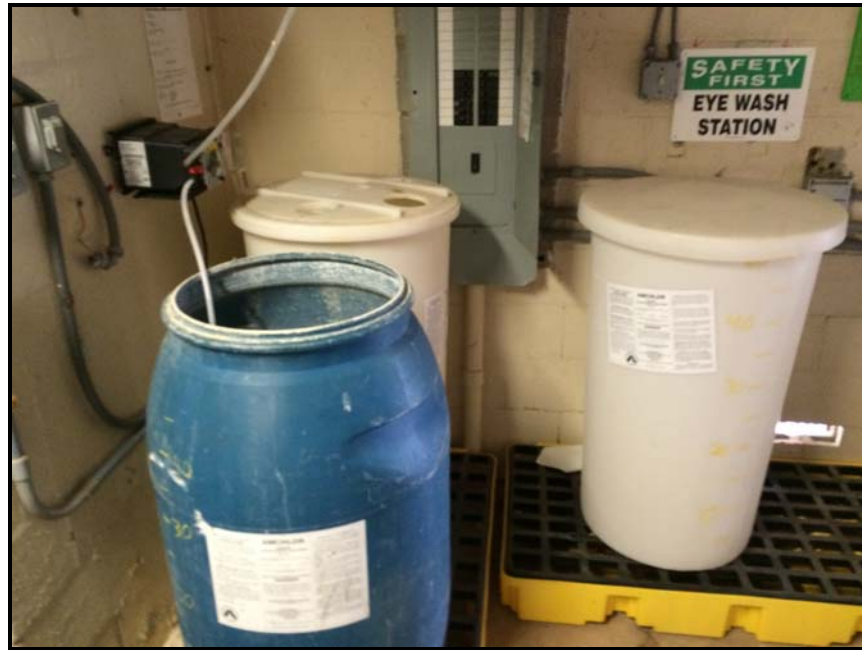
Chemical Storage within secondary containments
