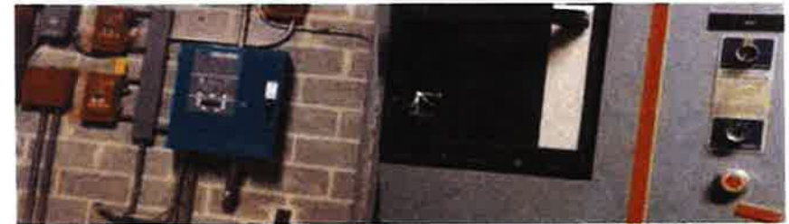
FIRE ALARM & GENERATOR PANEL
