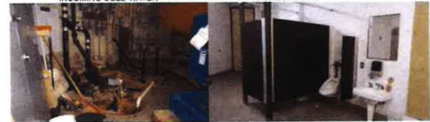
SUMP & SWITCH PUMP
