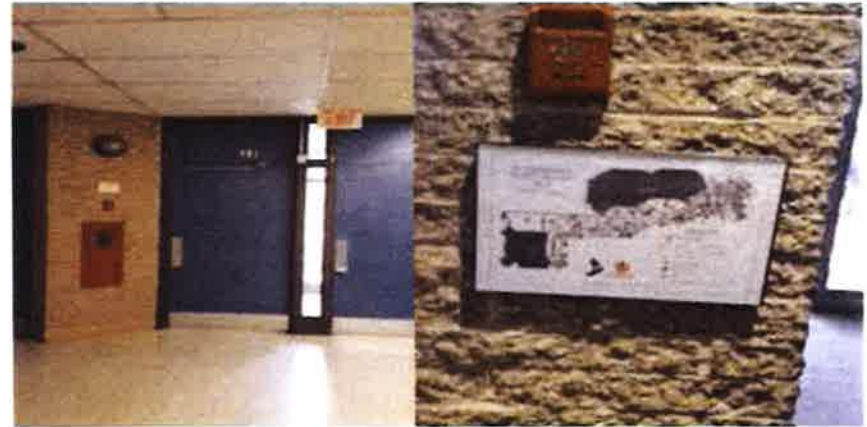
EXIT SIGN (TYPICAL)
