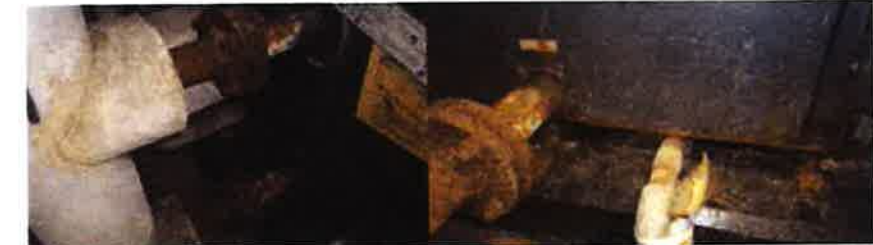
UNINSULATED PIPING AT AHU
