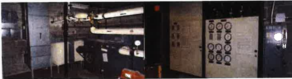
AIR HANDLING UNIT
