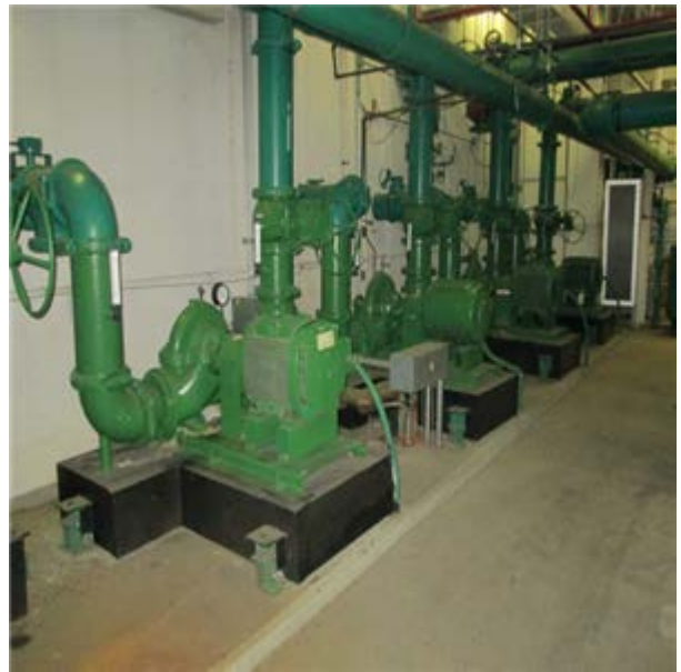
ChW Primary Pump, Base Mt, Var Spd, High Eff 60 HP:- Chiller water pump
