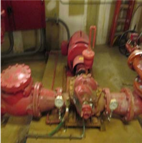
Sprinkler fire pump
