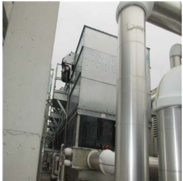
Cooling Tower, 250 Ton:- Cooling tower
