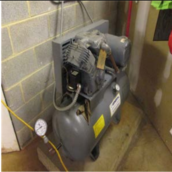
Compressor :- Dry sprinkler system air compressor
