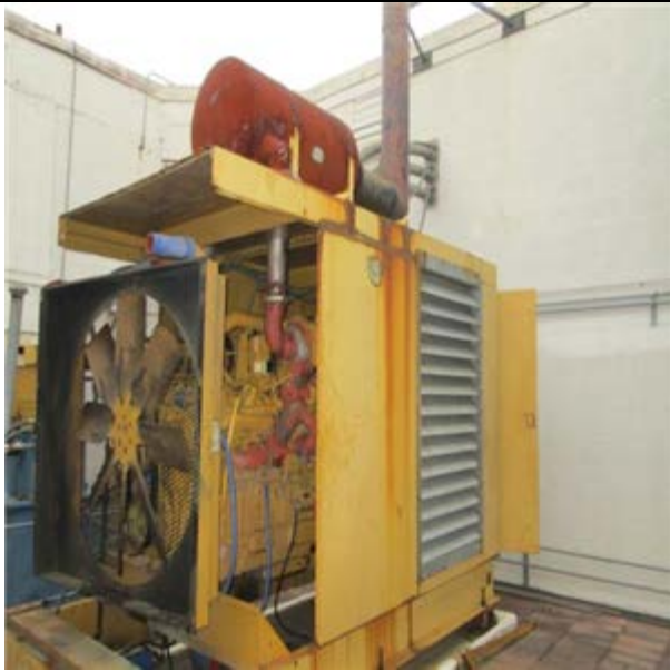
Generator, Diesel, 500 kW :- Emergency generator
