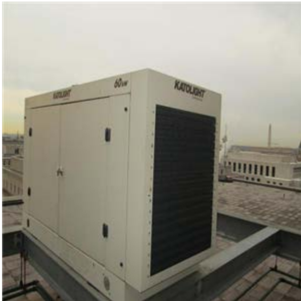
Generator, Diesel, 60 kW :- Emergency generator
