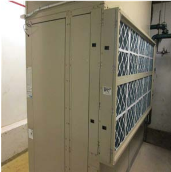
Self contained fan coil
