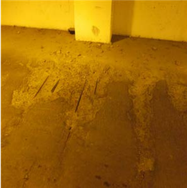
Damaged concrete slab
