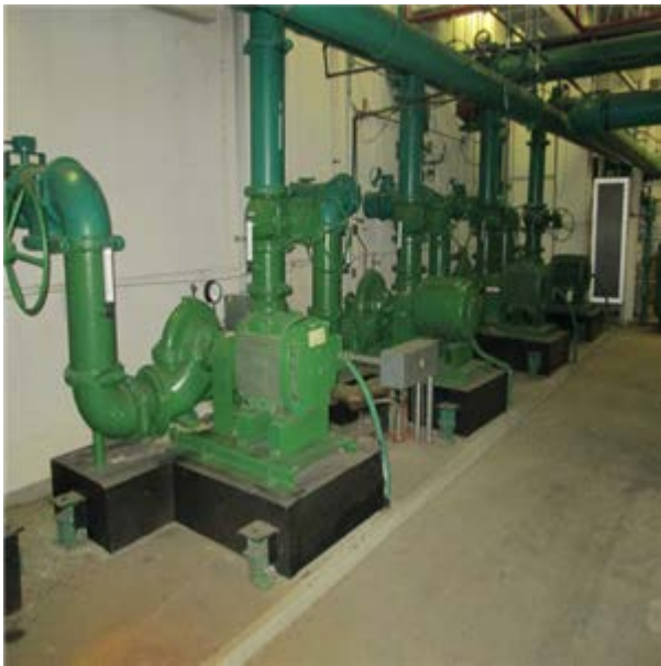
ChW Primary Pump, Base Mt, Var Spd, High Eff 60 HP :- Chilled water pump
