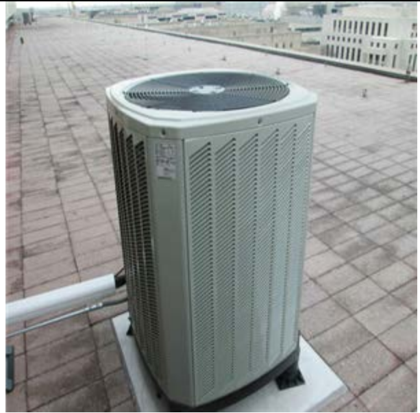
Heat Pump, 5 Ton:- Roof mounted heat pump
