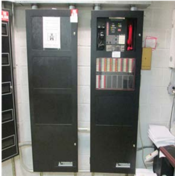
Fire alarm equipment
