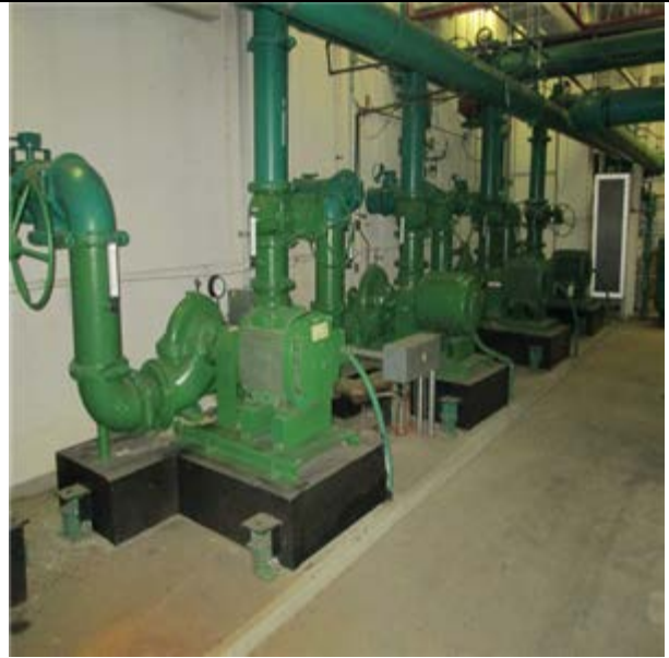
ChW Primary Pump, Base Mt, Var Spd, High Eff 60 HP:- Chilled water pump
