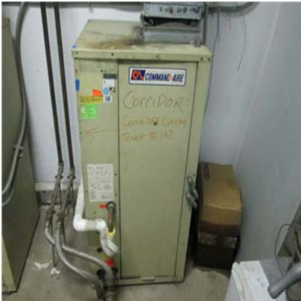
Air Handler, Single Zone, 800 Cfm :- Air handler
