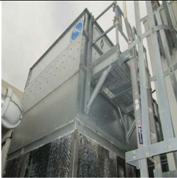
Cooling Tower, 250 Ton :- Rooftop cooling tower
