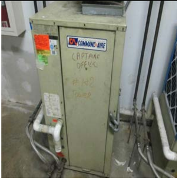
Air Handler, Single Zone, 800 Cfm :- Air handler
