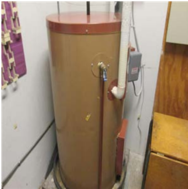
Water Heater, Electric, 65 Gal :- Electric water heater
