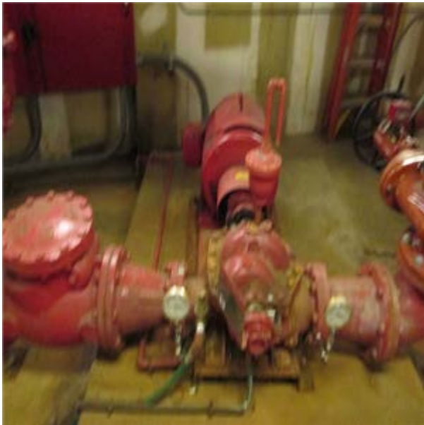
Sprinkler Pumping Equipment :- Sprinkler fire pump
