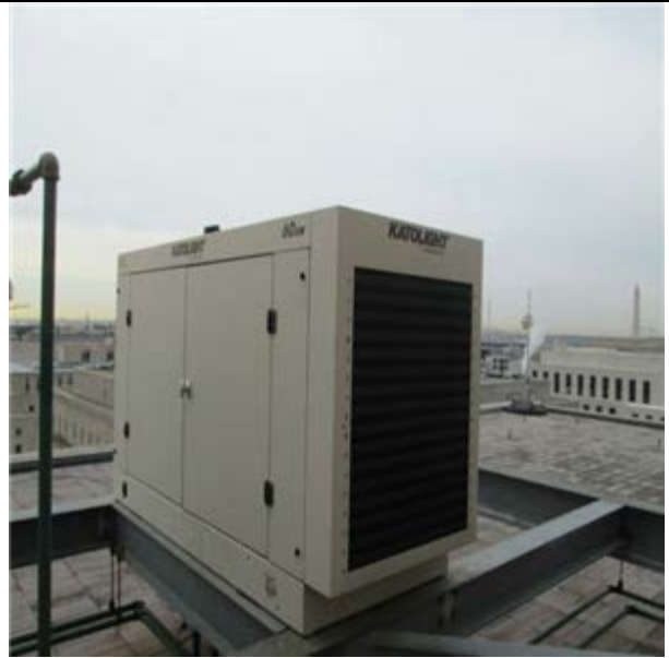
Generator, Diesel, 60 kW:- Diesel generator
