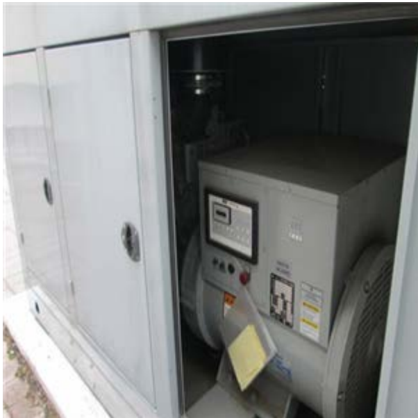
Generator, Diesel, 225 kW :- Emergency generator
