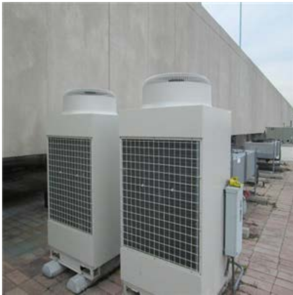
Condenser, Air-Cooled, 10 Ton :- Roof mounted condensers
