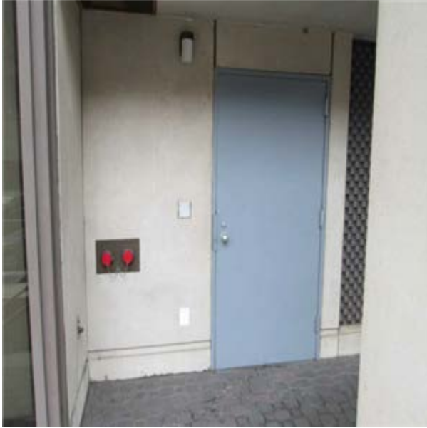
Exterior steel door
