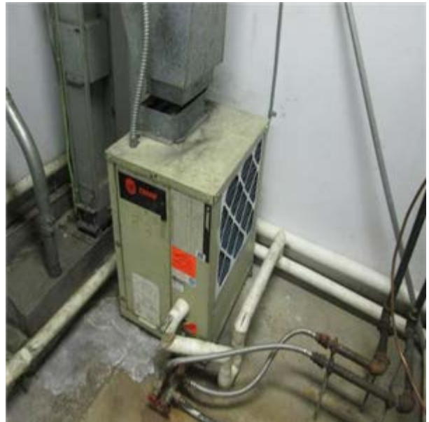
Air Handler, Single Zone, 400 Cfm:- Air handler
