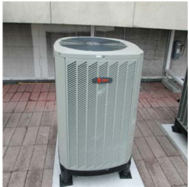
Heat Pump, 5 Ton:- Roof mounted heat pump
