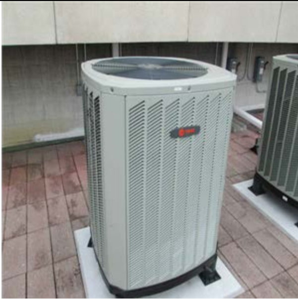
Heat Pump, 5 Ton :- Roof mounted heat pump
