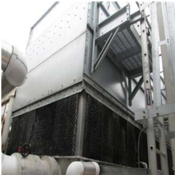
Cooling Tower, 250 Ton :- Cooling tower
