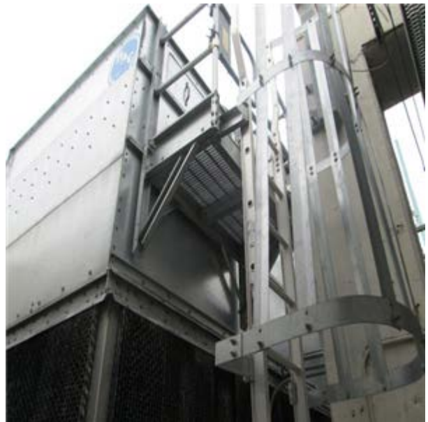
Cooling Tower, 250 Ton:- Cooling tower
