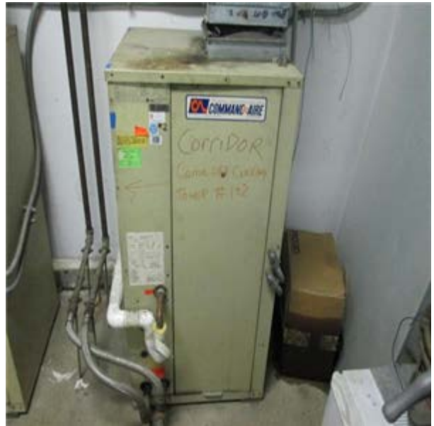
Air Handler, Single Zone, 800 Cfm:- Air handler
