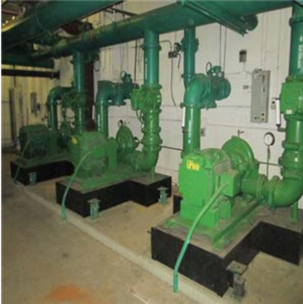
Chilled water pumps
