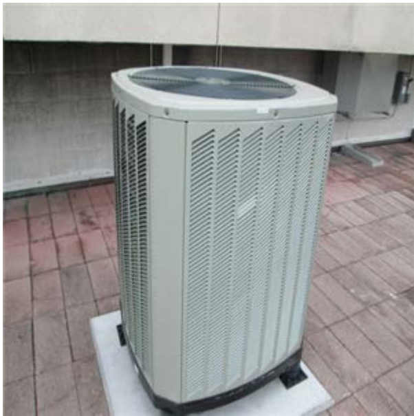
Heat Pump, 5 Ton :- Roof mounted heat pump
