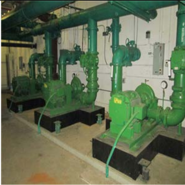
ChW Primary Pump, Base Mt, Var Spd, High Eff 60 HP :- Chilled water pump
