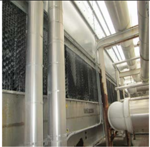
Cooling Tower, 250 Ton:- Rooftop cooling tower
