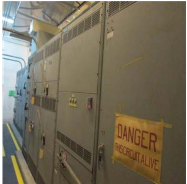
Main Switchgear Double-Ended 480 Y 277 V 4000 Amp:- Electrical switchgear
