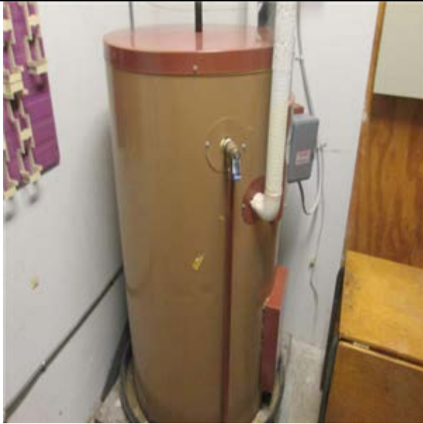
Water Heater, Electric, 65 Gal :- Electric water heater
