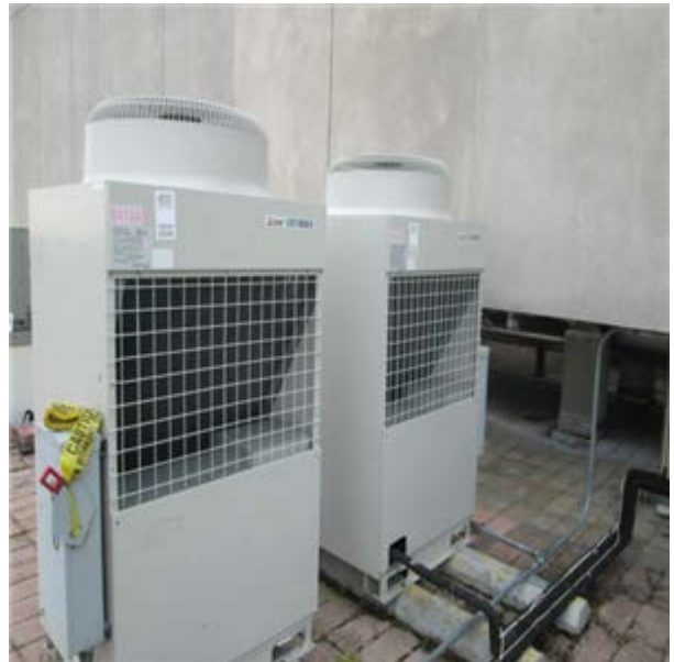
Condenser, Air-Cooled, 10 Ton:- rooftop condenser
