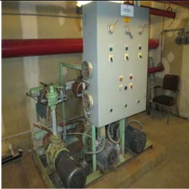
Booster Pump, 7.500 HP :- Booster pumps
