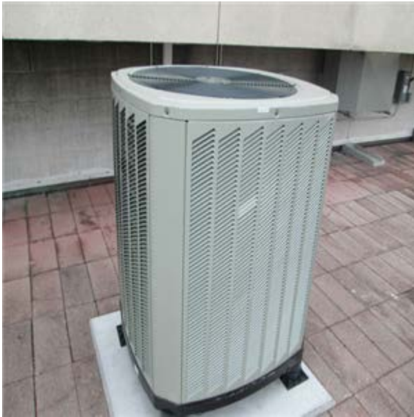
Roof mounted heat pump
