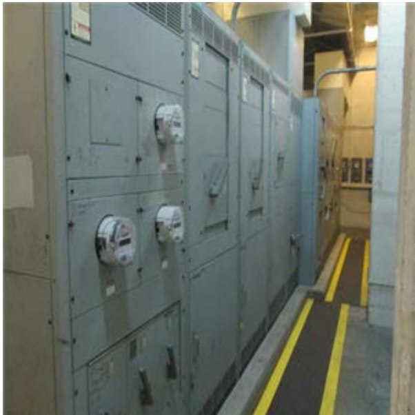
Main Switchgear Double-Ended 480 Y 277 V 4000 Amp :- Main electrical switchgear
