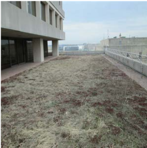
Green Roof w Growing Medium, Rubberized Asphalt :- Green roof
