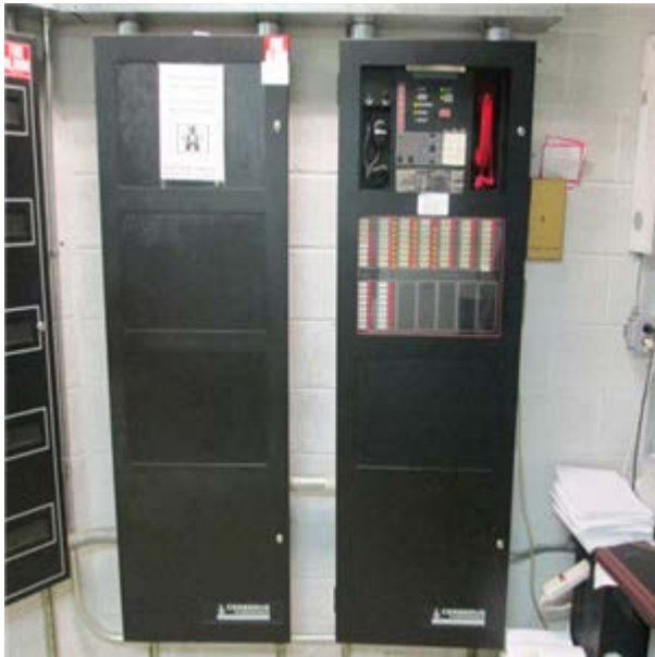
Fire Alarm System Devices :- Fire alarm equipment
