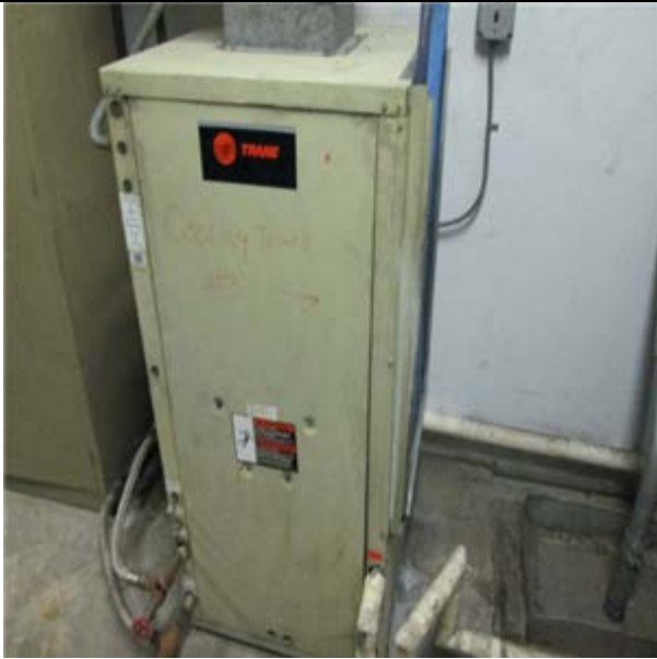
Air Handler, Single Zone, 800 Cfm :- Air handler
