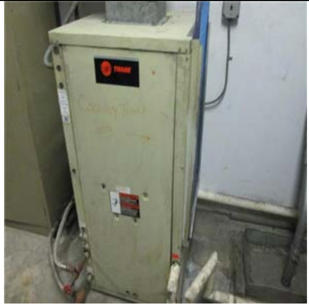
Air Handler, Single Zone, 800 Cfm:- Air handler
