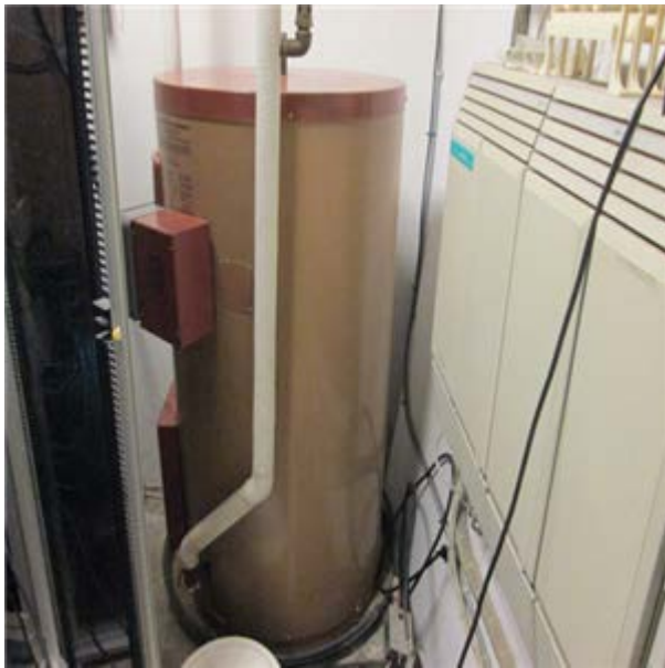
Water Heater, Electric, 65 Gal :- Electric water heater
