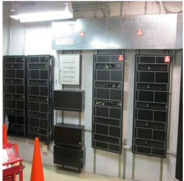
Fire Alarm System Devices :- Fire alarm equipment
