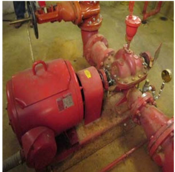
Sprinkler Pumping Equipment:- Sprinkler fire pump
