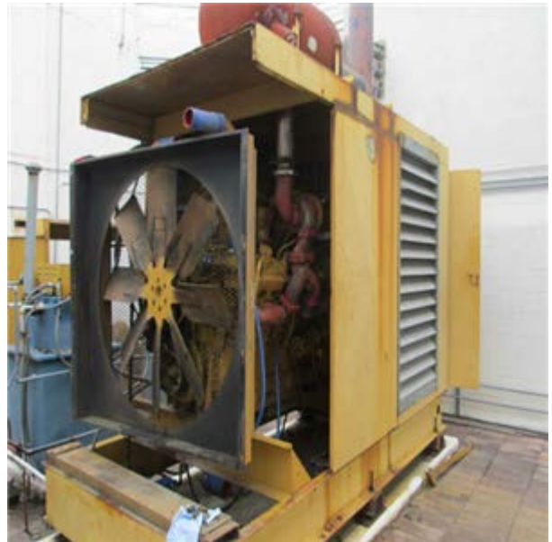
Generator, Diesel, 500 kW:- Diesel generator
