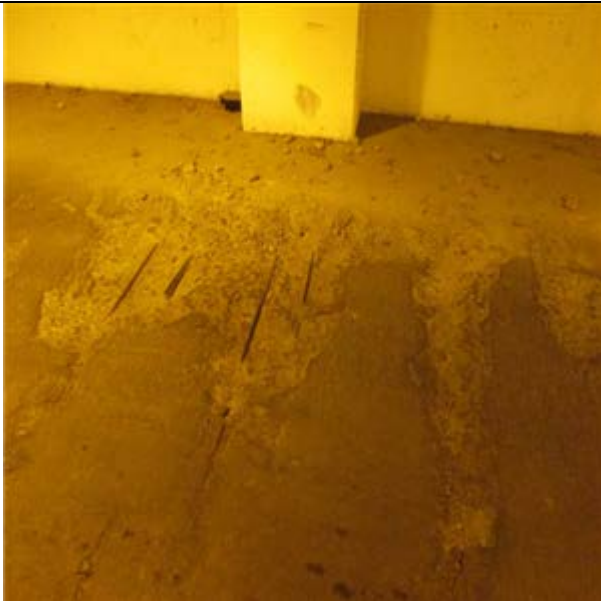
Concrete Slab :- Damaged concrete slab
