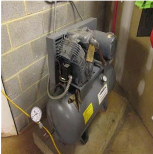
Dry sprinkler air compressor
