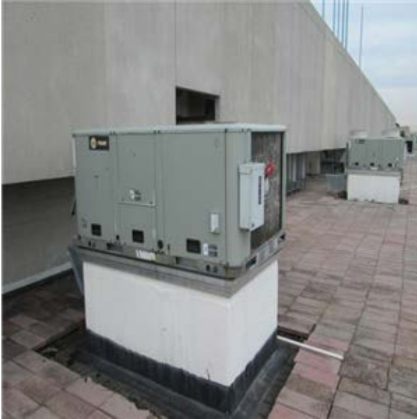
Packaged rooftop unit
