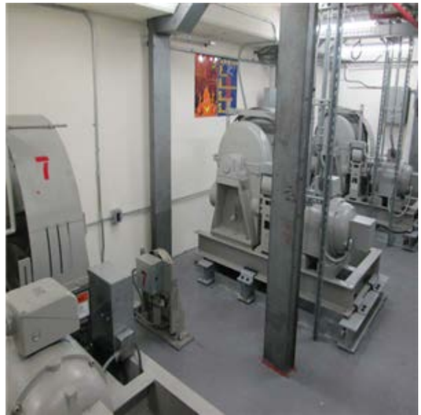
Elevator, Geared, 3-5 Floor, 3,000 Lbs, 300 fpm:- Elevator machinery
