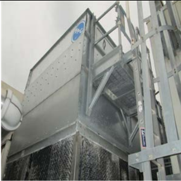
Cooling Tower, 250 Ton :- Cooling tower
