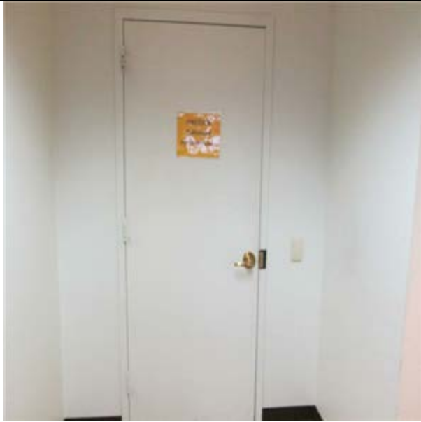
Magnetic Lock :- Door with magnetic lock
