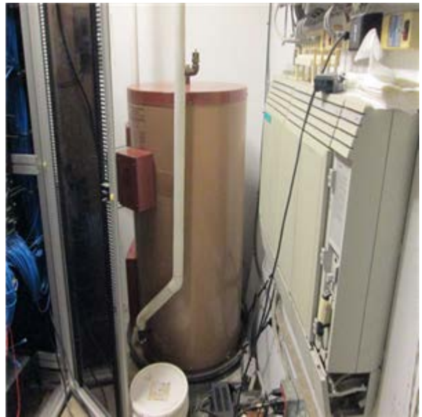
Water Heater, Electric, 65 Gal:- Electric water heater
