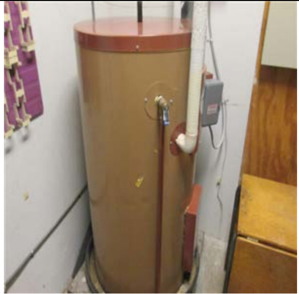
Water Heater, Electric, 65 Gal:- Electric water heater
