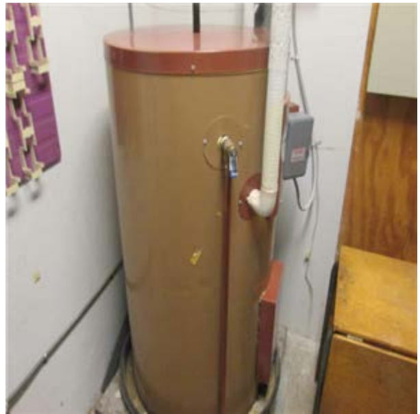
Water Heater, Electric, 65 Gal:- Electric water heater
