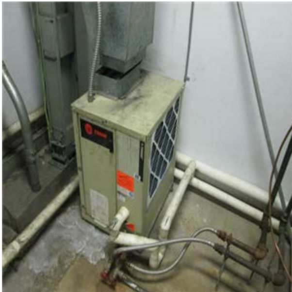
Air Handler, Single Zone, 400 Cfm :- Air handler
