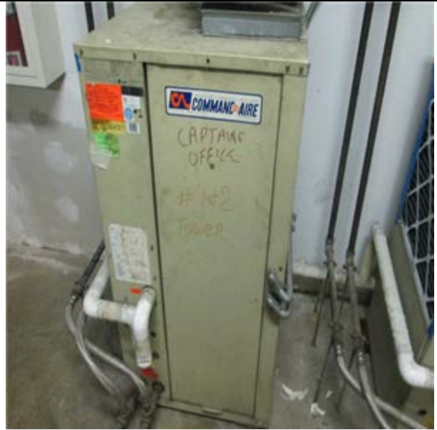
Air Handler, Single Zone, 800 Cfm:- Air handler
