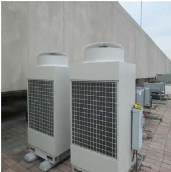
Roof mounted condensers
