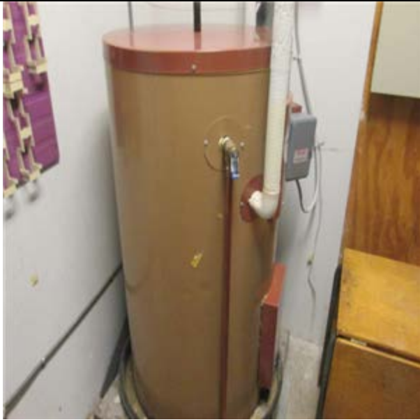
Water Heater, Electric, 65 Gal :- Electric water heater
