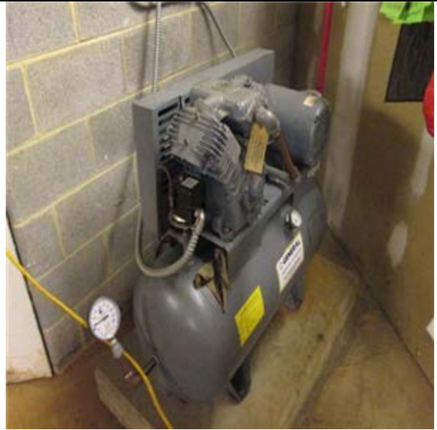
Compressor:- Dry sprinkler air compressor
