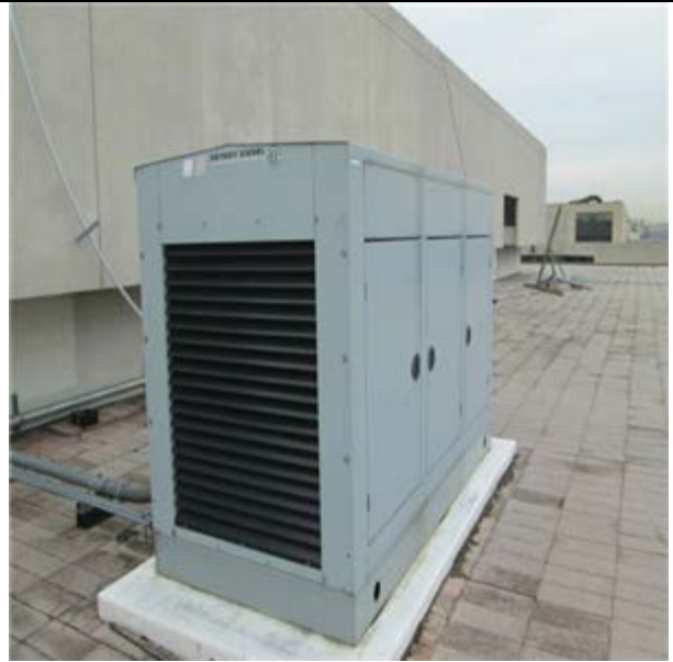
Generator, Diesel, 225 kW:- Diesel generator
