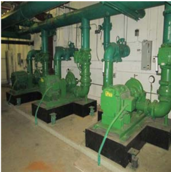
ChW Primary Pump, Base Mt, Var Spd, High Eff 60 HP :- Chilled water pumps
