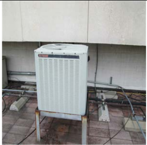
Heat Pump, 3 Ton:- Heat pump
