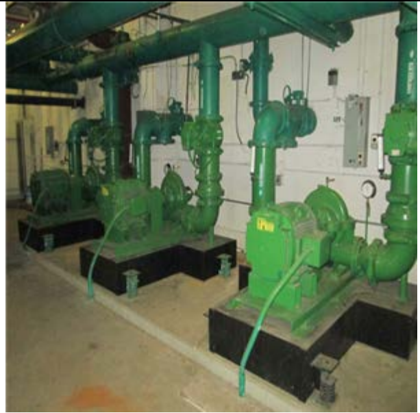
ChW Primary Pump, Base Mt, Var Spd, High Eff 60 HP:- Chilled water pumps
