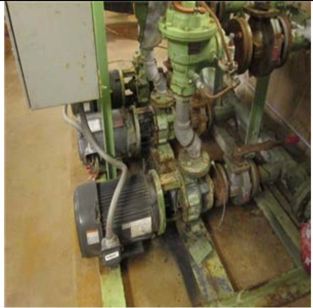
Booster Pump, 7.500 HP:- Corrosion at booster pumps
