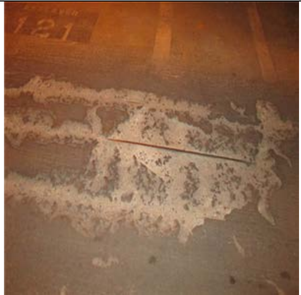
Concrete Slab:- Damaged concrete slab
