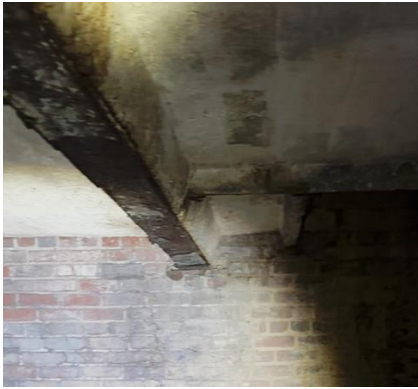
Figure 7: Coal vault roof with exposed steel beam flange
