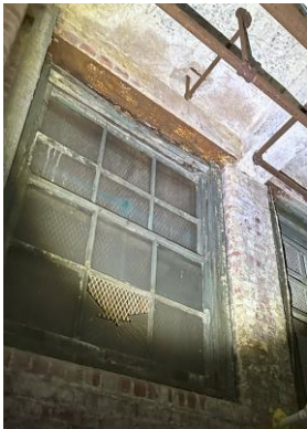
Figure 9: Interview view of lintel over window
