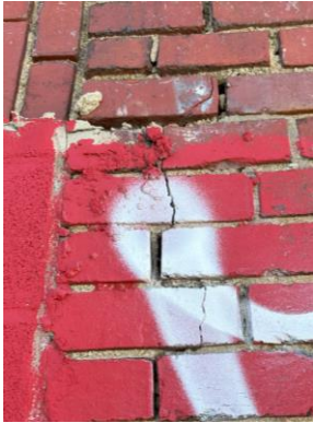
Figure 1: Exterior Wall - Cracked brick
