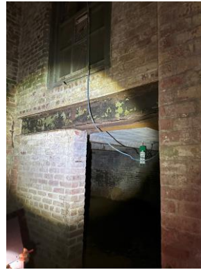
Figure 8: Rusted lintel at entry to Coal Vault
