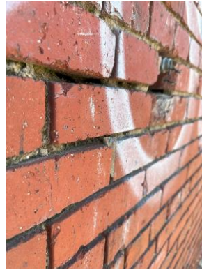
Figure 2: Exterior Wall – Mortar loss
