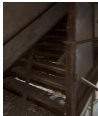
Figure 6: Corroded stair pans
