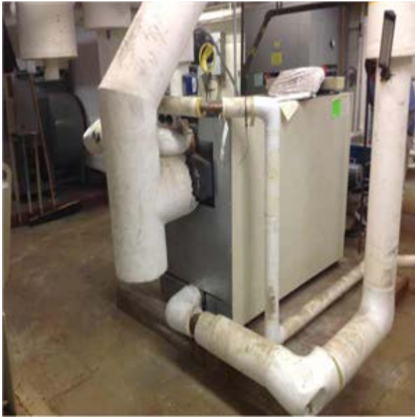
One of two boilers
