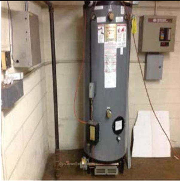
Domestic Hot Water Heater - Gas :- (null)
