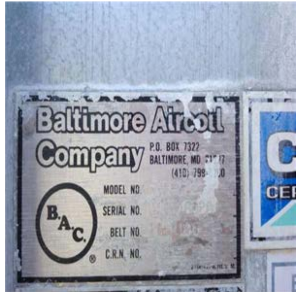
Cooling Tower, 50 Ton
