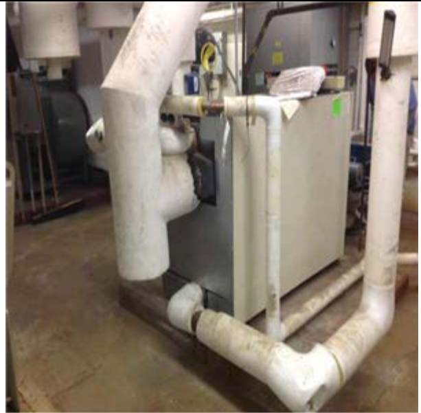
Boiler, Gas, 1,000 Mbh:- one of two boilers
