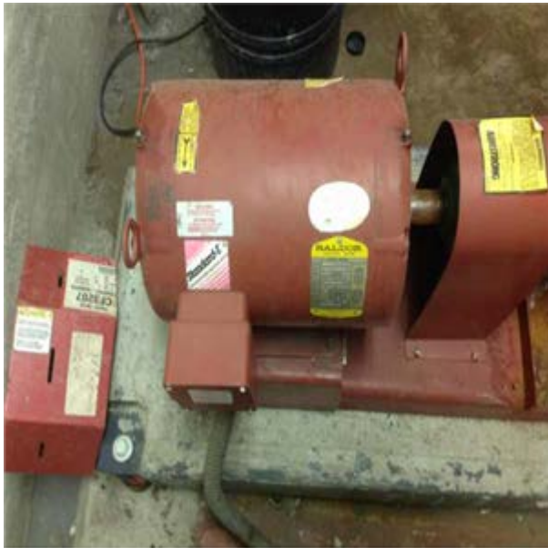
Circulation Pump, Hot Water, 7.500 HP :- (null)
