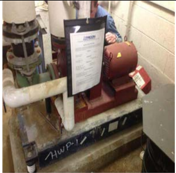
Circulation Pump, Hot Water, 7.500 HP:- (null)
