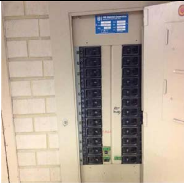
Power Panel Board, 208 Y, 120 V, 225 Amp :- (null)
