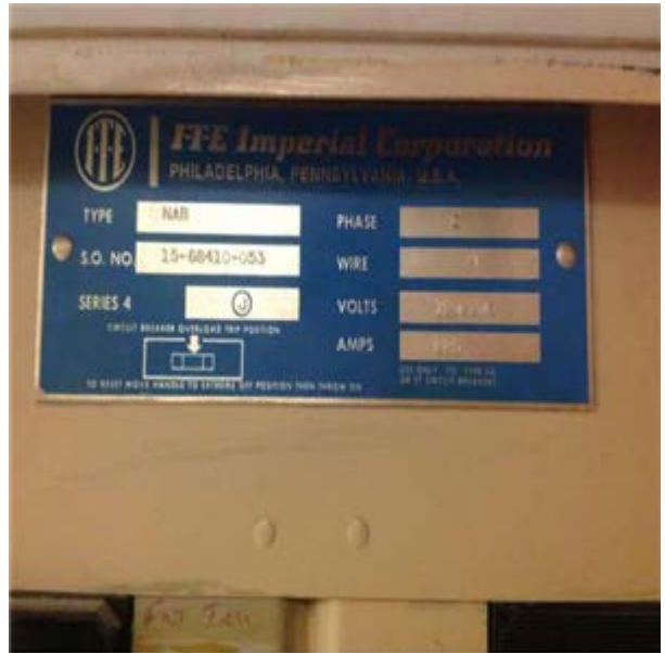
Power Panel Board, 208 Y, 120 V, 225 Amp:- (null)
