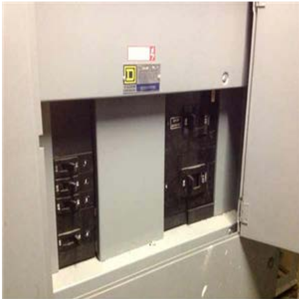
Power Panel Board, 208 Y, 120 V, 400 Amp
