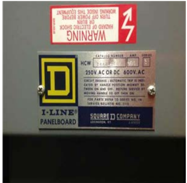
Power Panel Board, 208 Y, 120 V, 400 Amp:- (null)
