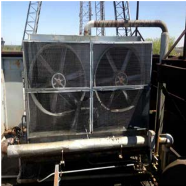
Cooling Tower, 50 Ton :- chiller on rooftop
