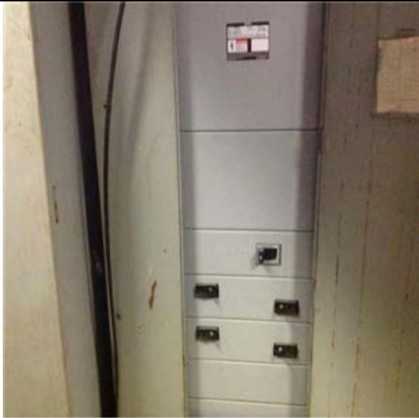
Power Panel Board, 208 Y, 120 V, 600 Amp :- (null)
