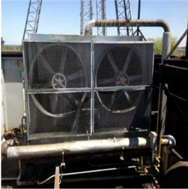
Chiller on rooftop
