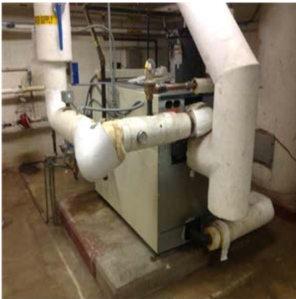
One of two boilers
