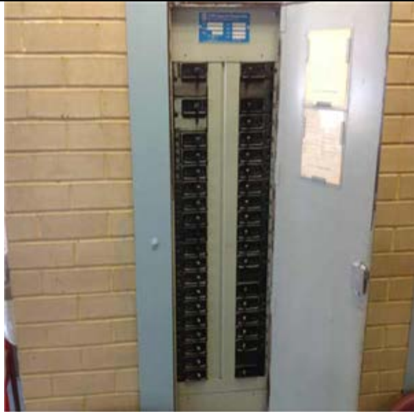
Power Panel Board, 208 Y, 120 V, 225 Amp :- (null)
