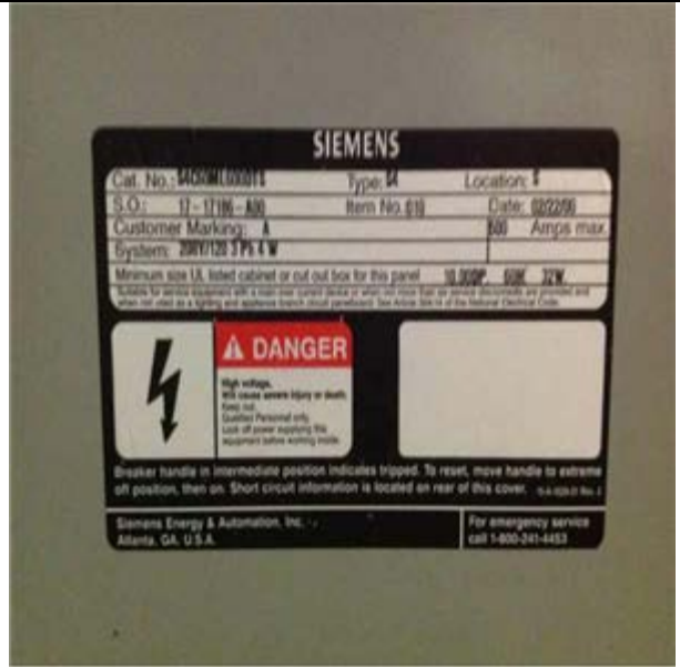
Power Panel Board, 208 Y, 120 V, 600 Amp
