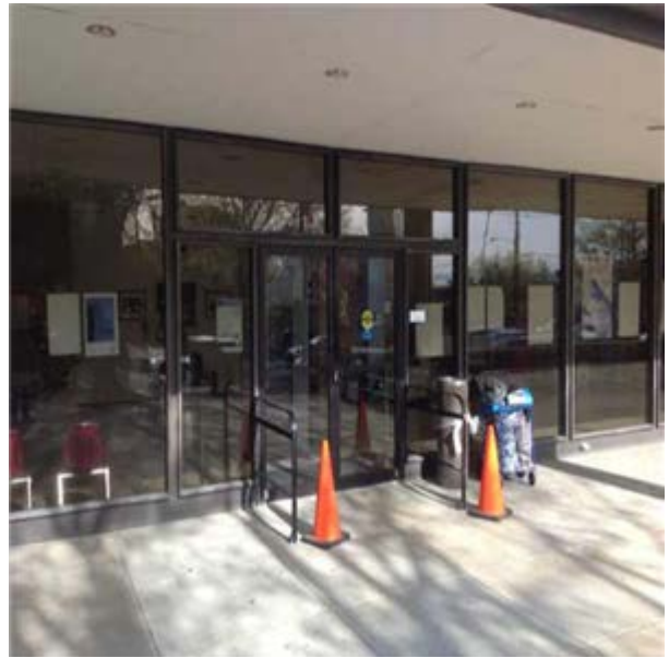
Glazed Aluminum Framed with Swing Doors:- main entrance
