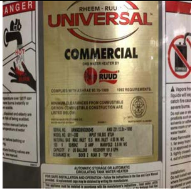
Domestic Hot Water Heater - Gas:- (null)
