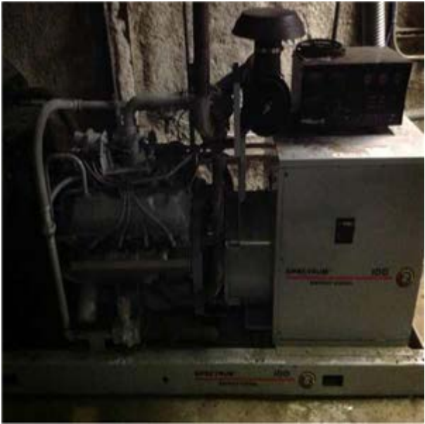
Generator, natural gas, 125 kW
