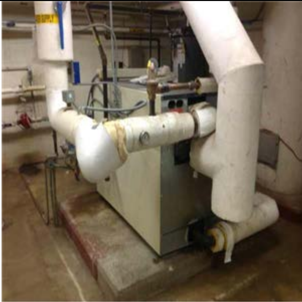
Boiler, Gas, 1,000 Mbh :- one of two boilers
