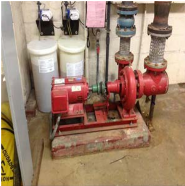
Circulation Pump, Hot Water, 15.000 HP :- (null)
