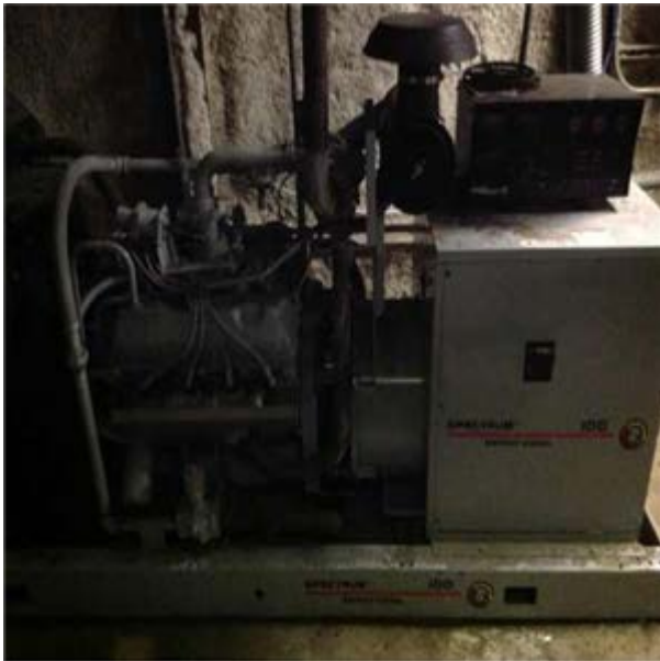
Generator, natural gas, 125 kW :- Generator, natural gas, 125 kW
