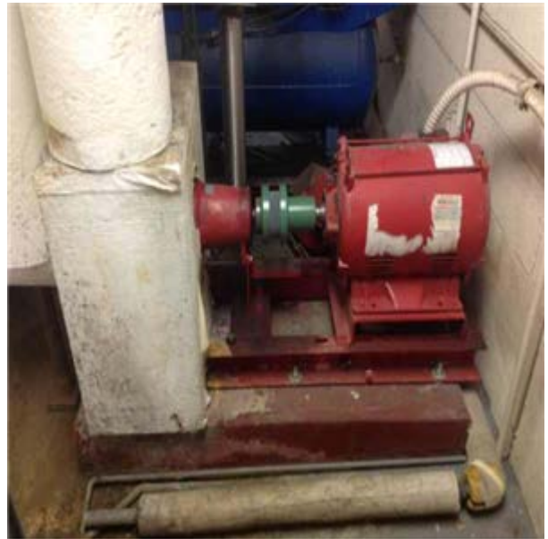
Circulation Pump, Hot Water, 25.000 HP:- (null)
