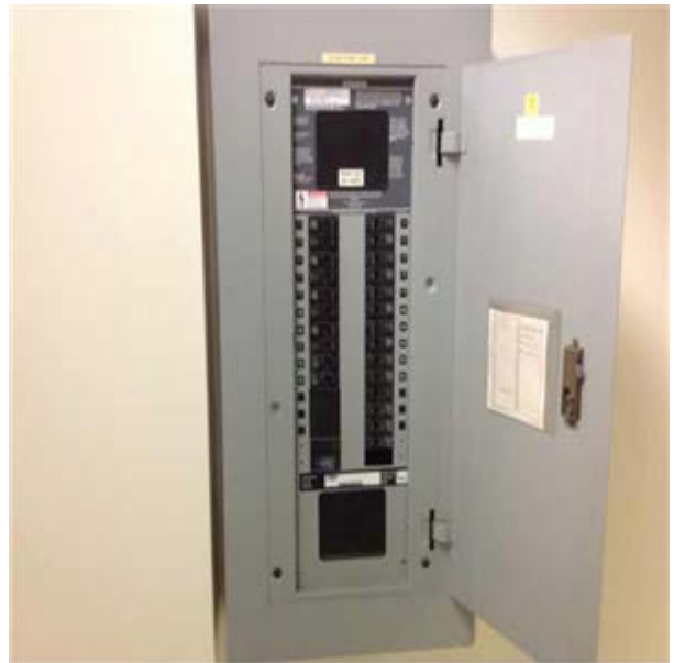
Power Panel Board, 208 Y, 120 V, 125 Amp:- Power Panel Board, 208 Y, 120 V, 125 Amp
