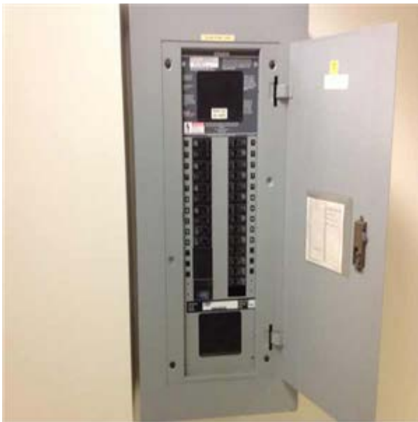
Power Panel Board, 208 Y, 120 V, 125 Amp
