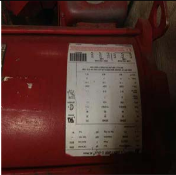
Circulation Pump, Hot Water, 25.000 HP :- (null)
