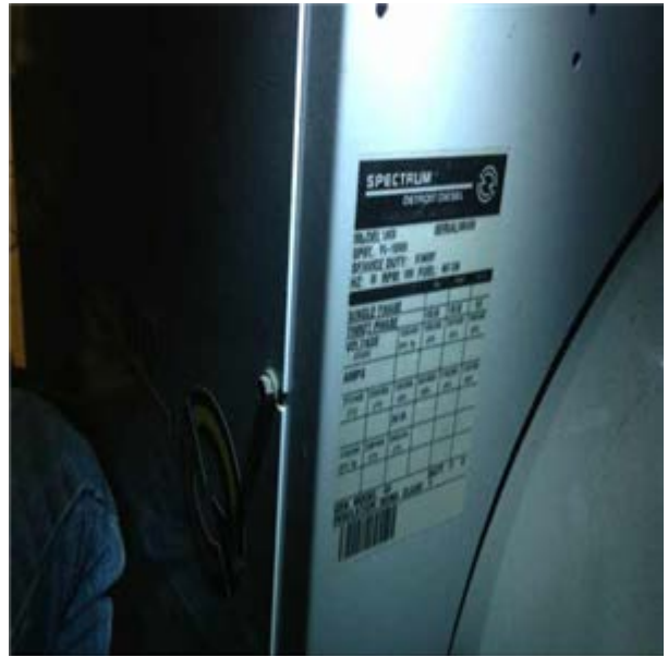
Generator, natural gas, 125 kW:- (null)
