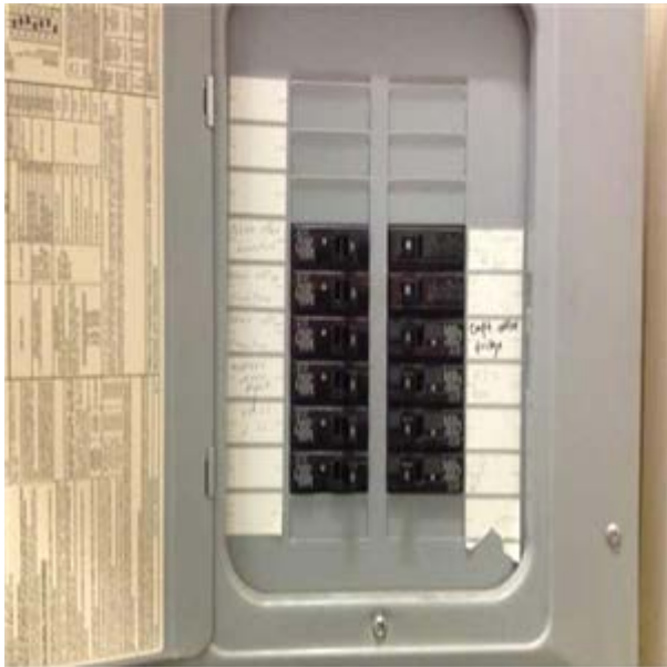
Power Panel Board, 480 Y, 277 V, 100 Amp :- (null)
