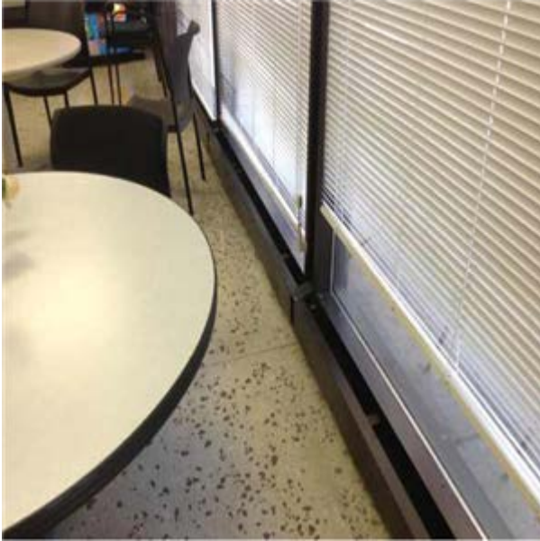
Baseboard hot water fin tube radiators
