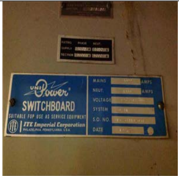
Main Switchgear, 480 Y, 277 V, 4,000 Amp:- (null)
