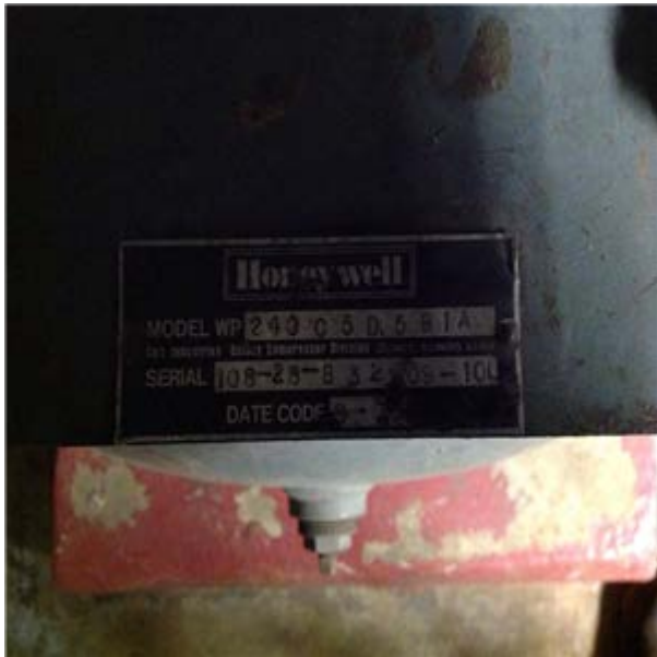
Compressor :- Compressor Nameplate
