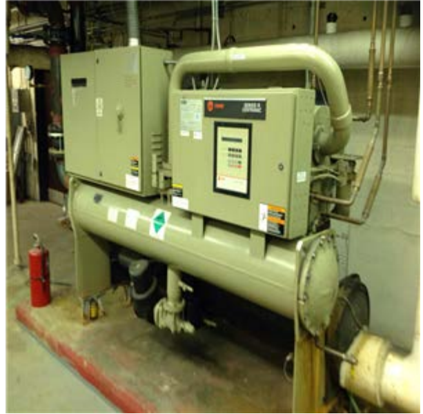
Chiller, Reciprocating Water-Cooled Hermetic, 15 Ton:- Trane Chiller
