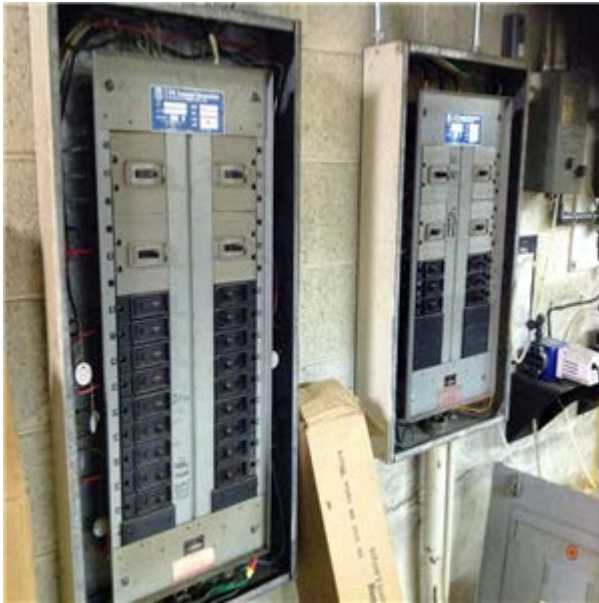
100 Amp Breaker Panels
