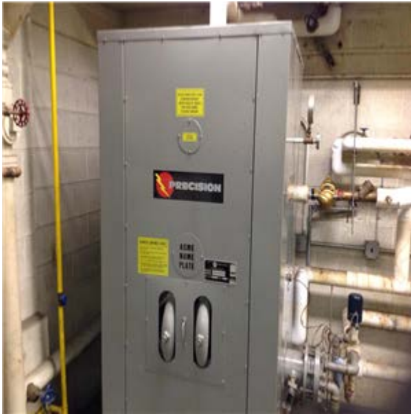
Domestic Hot Water Boiler
