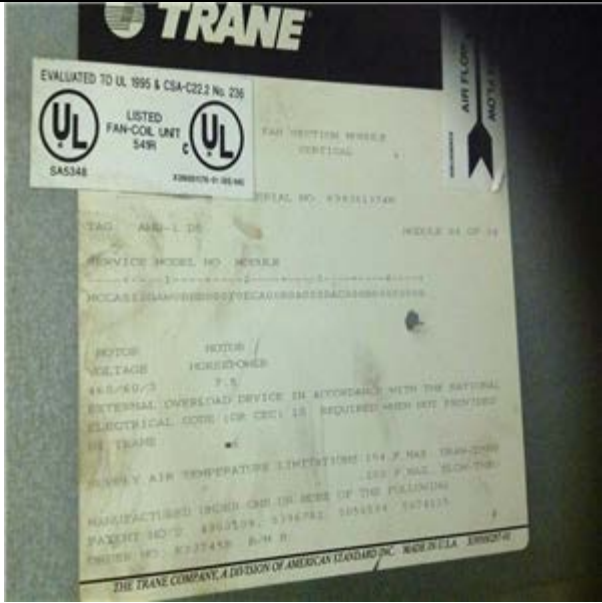
Air Handler, Multizone, 25,000 Cfm :- Air Handler Nameplate
