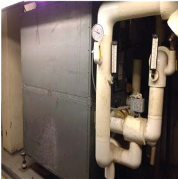
Trane Air Handler
