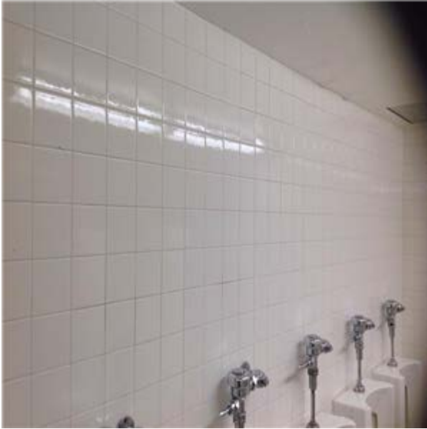
Locker Room Ceramic Tile Wall Finish
