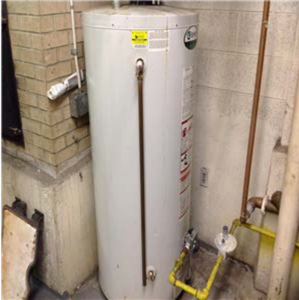
Domestic Water Heater
