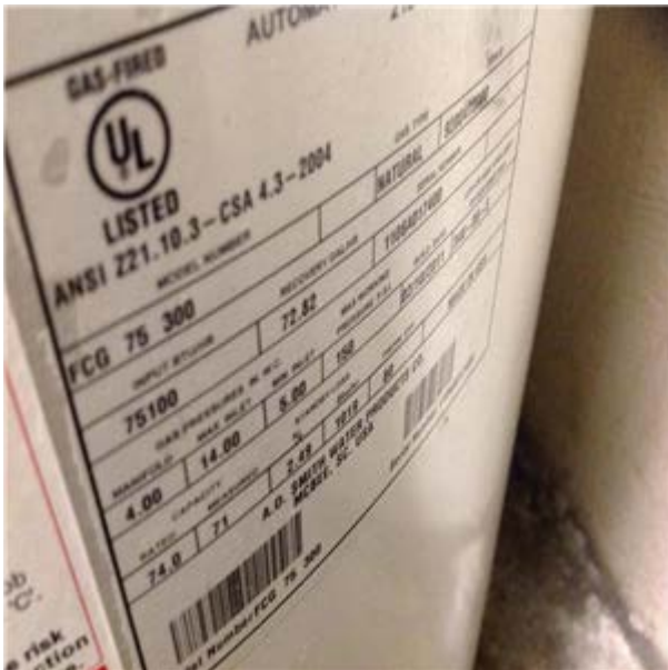
Domestic Hot Water Heater - Gas :- Domestic Water Heater Nameplate
