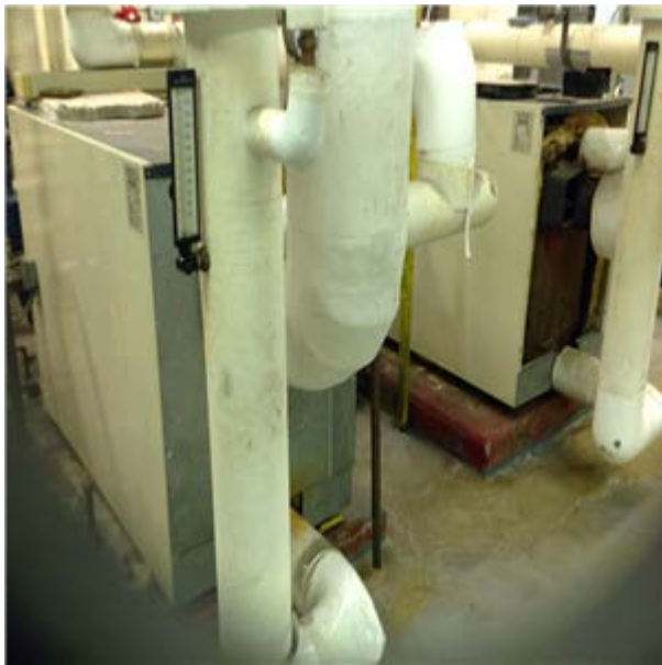
Boiler, Gas, 1,000 Mbh :- Duel Fuel Heating Boilers
