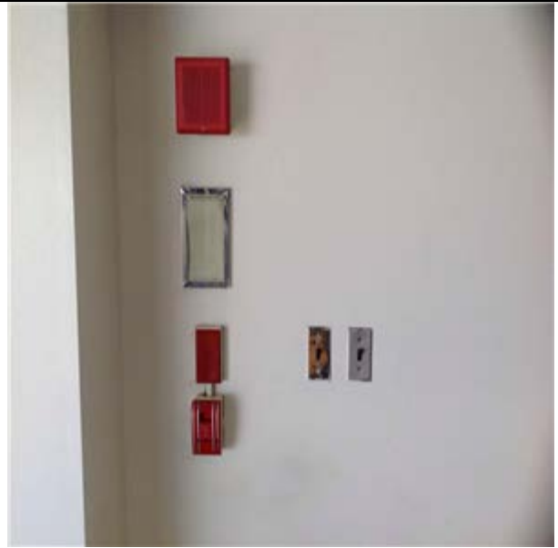
Central Fire Alarm System:- Central Fire Alarm System Components
