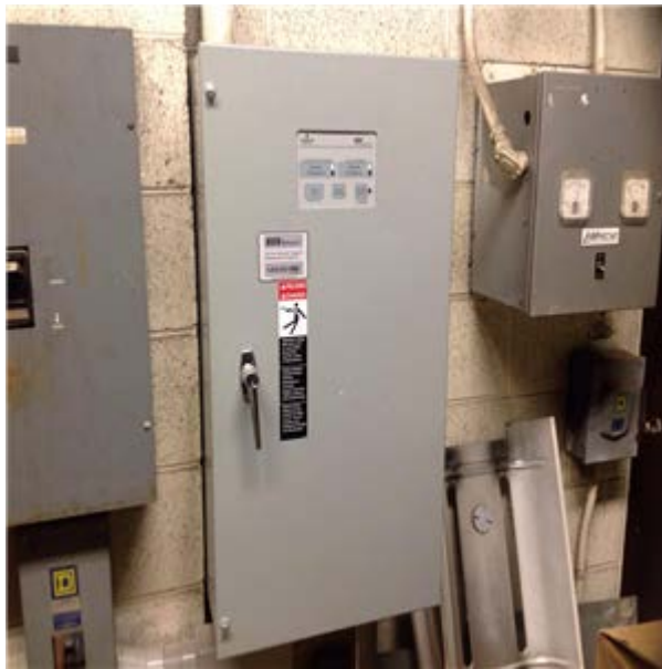
Generator Transfer Switch
