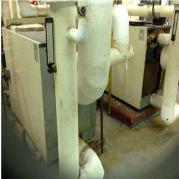
Duel Fuel Heating Boilers
