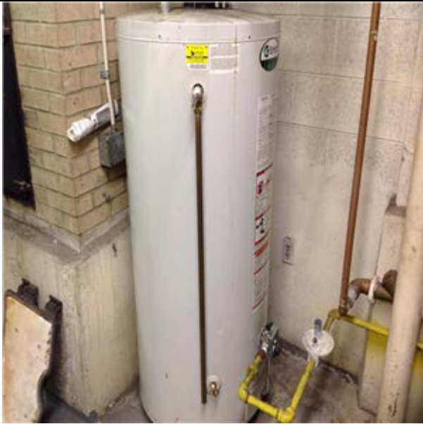
Domestic Hot Water Heater - Gas :- Domestic Water Heater
