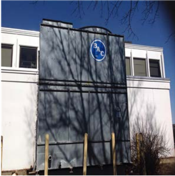
Pad Mounted BAC Cooling Tower
