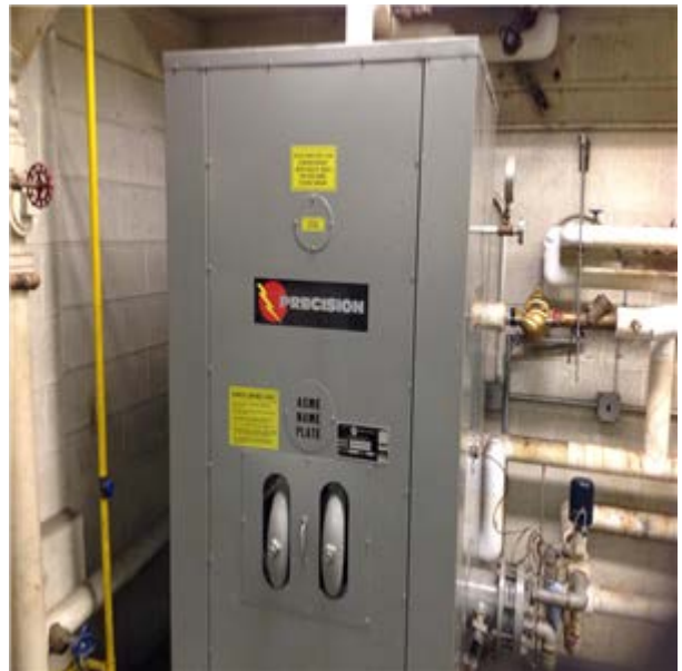
Domestic Hot Water Heater - Gas:- Domestic Hot Water Boiler
