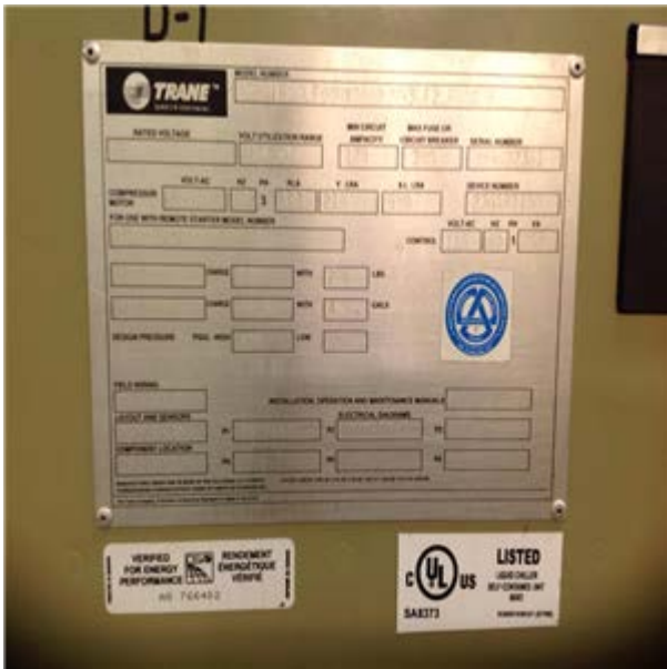
Chiller, Reciprocating Water-Cooled Hermetic, 15 Ton :- Chiller Nameplate
