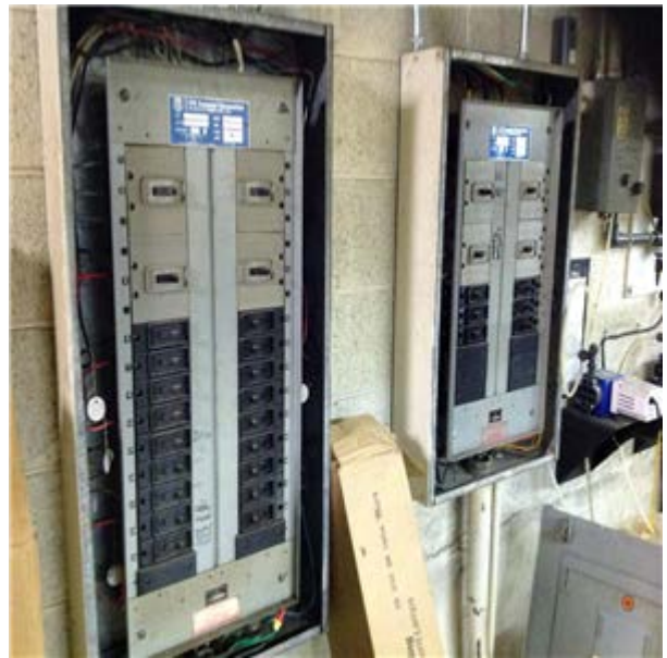
Circuit Breaker, 3 Ph., 600 V, 100 Amp:- 100 Amp Breaker Panels
