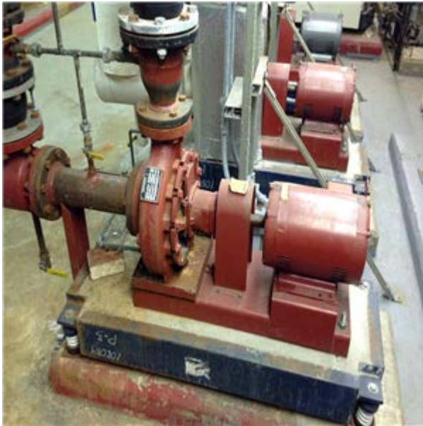
Domestic Hot Water Booster Pump
