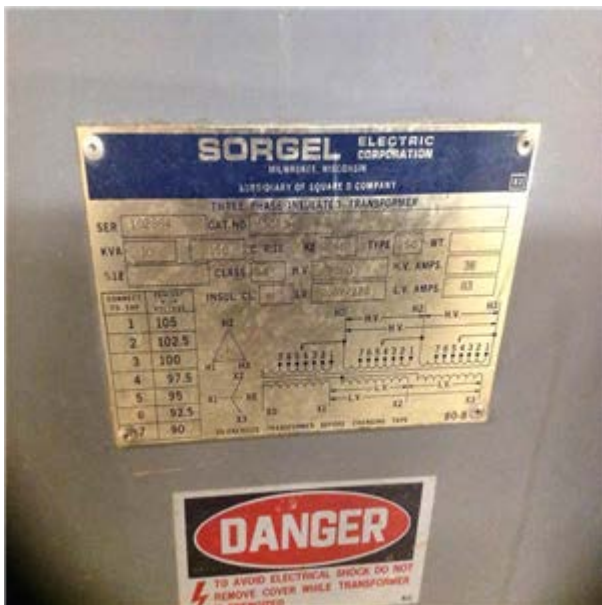
Secondary Transformer, Dry, 30 kVA :- Secondary Transformer Nameplate
