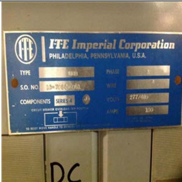
Circuit Breaker, 3 Ph., 600 V, 100 Amp :- Breaker Panel Nameplate
