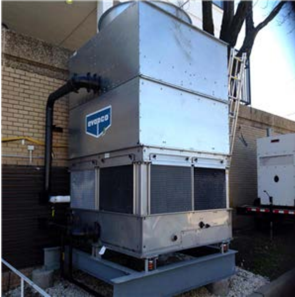
Evapco Cooling Tower
