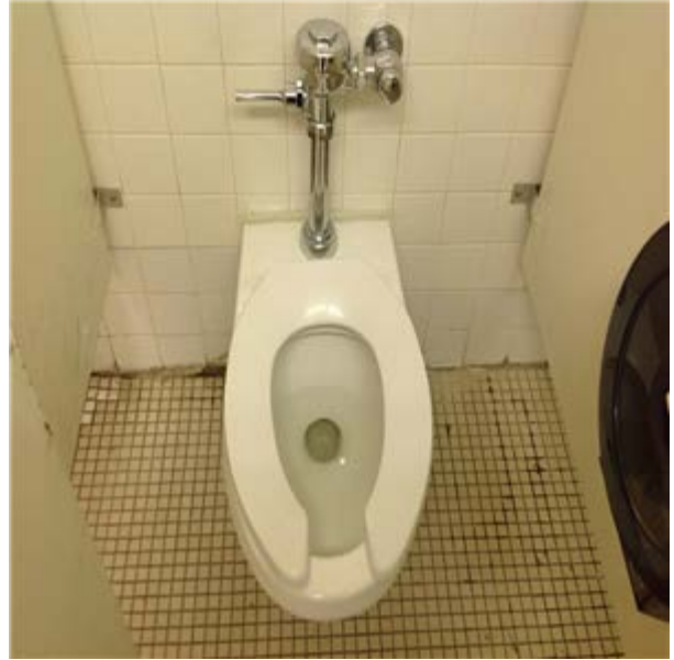
Flush Tank Water Closet, One Piece:- Locker Room Water Closet
