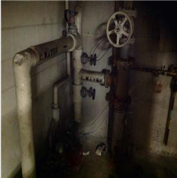
Water Main Piping
