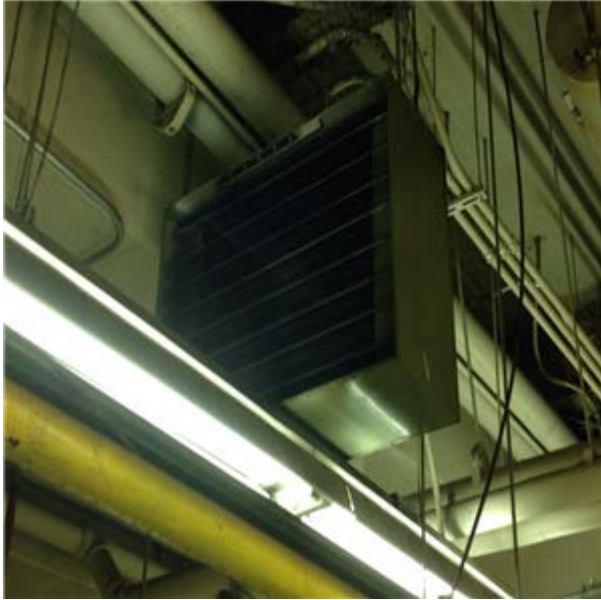
Electric Unit Heater :- Boiler Room Unit Heater
