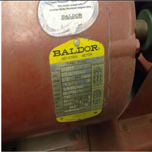
Booster Pump, 7.500 HP :- Domestic Hot Water Booster Pump Nameplate
