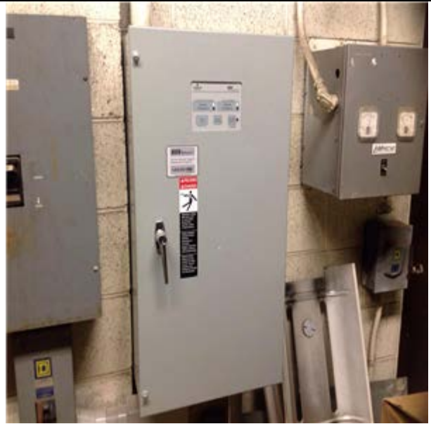
Generator Switchgear:- Generator Transfer Switch
