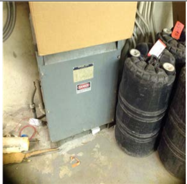
Secondary Transformer, Dry, 30 kVA:- Secondary Transformer
