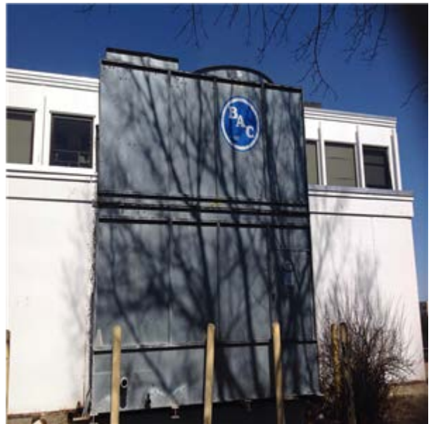
Cooling Tower, 50 Ton:- Pad Mounted BAC Cooling Tower
