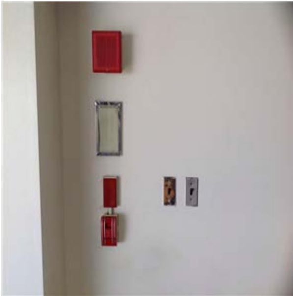
Central Fire Alarm System Components
