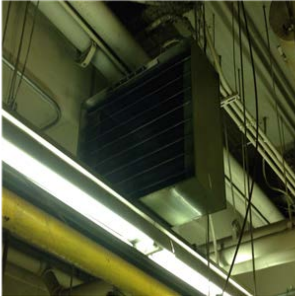
Boiler Room Unit Heater
