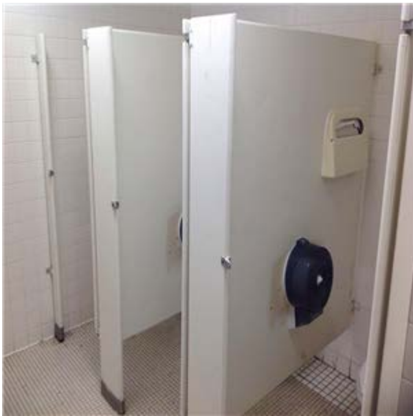
Toilet Partitions, Painted Metal, Overhead Braced :- Locker Room Metal Toilet Partitions
