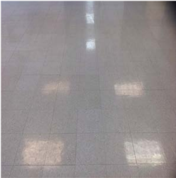
Vinyl Tile Flooring
