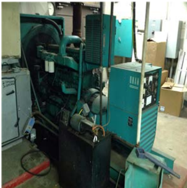
Generator, Diesel, 125 kW :- Diesel Generator
