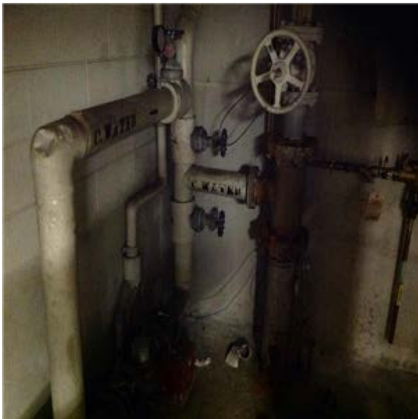
Domestic Water Main :- Water Main Piping
