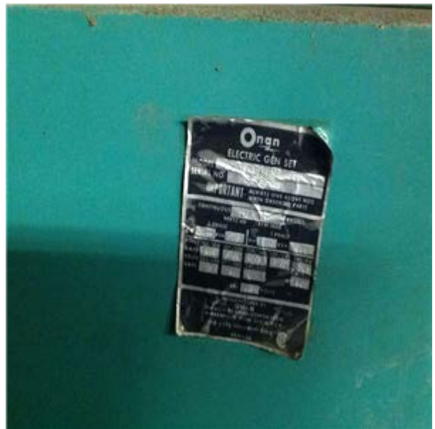
Generator, Diesel, 125 kW:- Diesel Generator Nameplate
