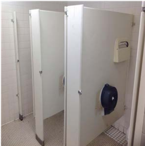
Locker Room Metal Toilet Partitions
