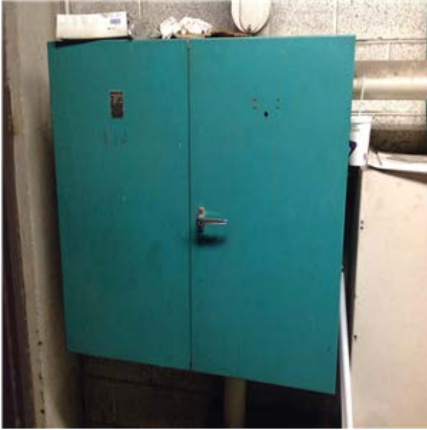
400 Amp Electric Disconnect
