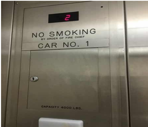
D1011 Passenger Elevators:- View of Elevators (x2)
