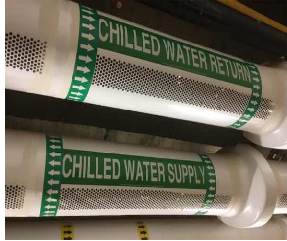
D3045 Chilled Water Distribution:- Chilled Water Piping
