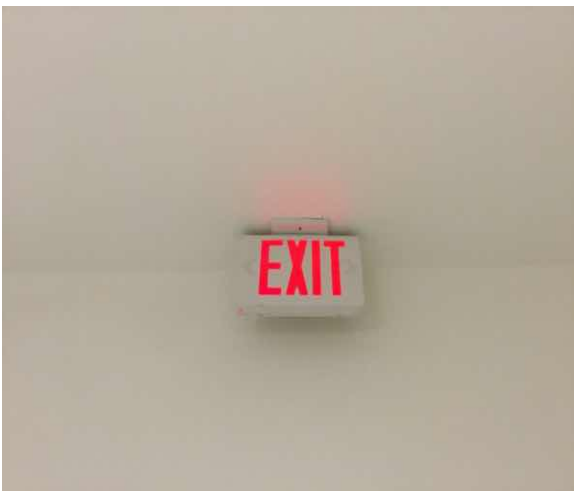
D5092 Emergency Light & Power Systems:- Exit Sign
