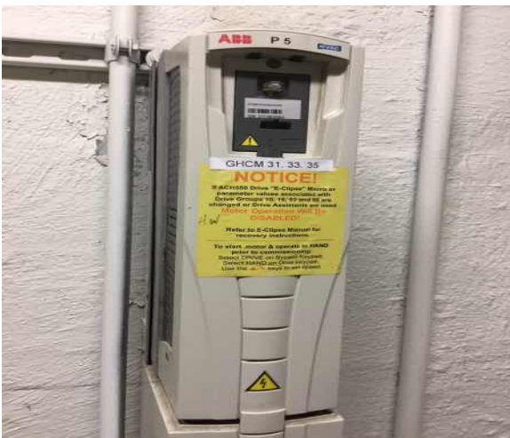
D3068 Building Automation Systems:- Broken VFD Controller of Hot Water Pump 5
