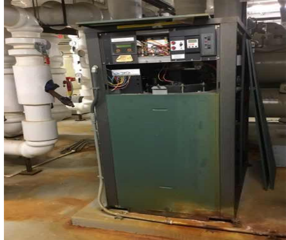
D3021 Boilers:- Boiler 3...not Working
