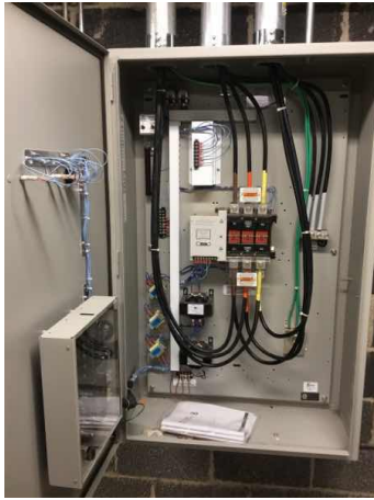
Automatic Transfer Switch
