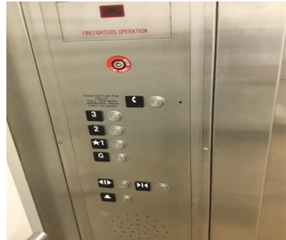
D1011 Passenger Elevators:- View of Elevators (x2)
