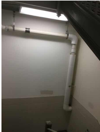
Rain Drainage Piping
