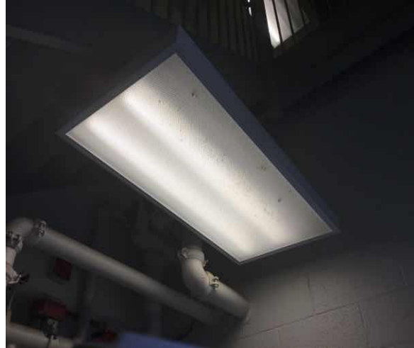
D5092 Emergency Light & Power Systems:- Emergency Light
