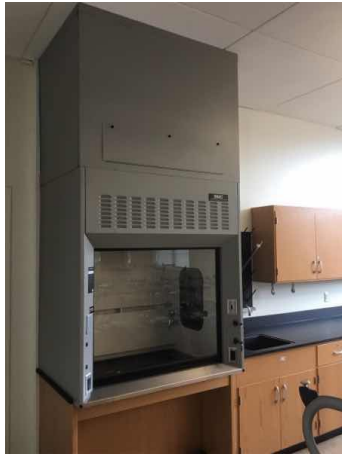
Laboratory Exhaust Hood
