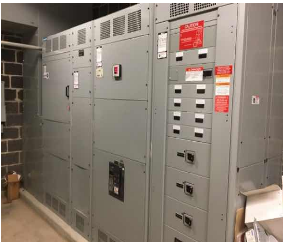
D5012 Low Tension Service & Dist.:- Switchboard
