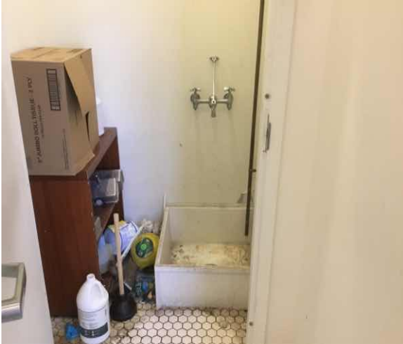
D2010.0 Water_Fixtures:- Mopping Sink
