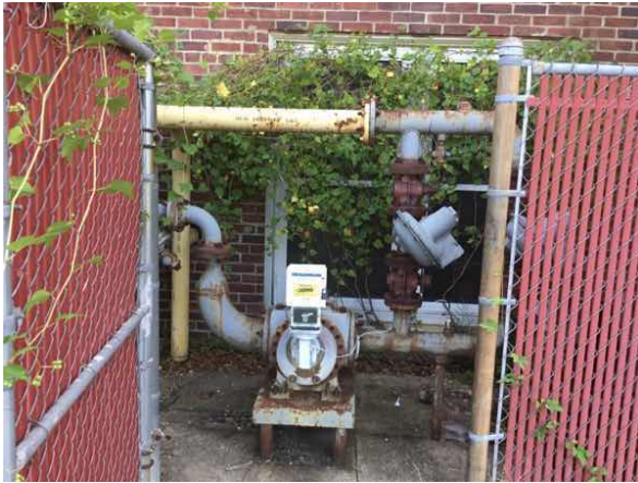
Fuel Gas Piping
