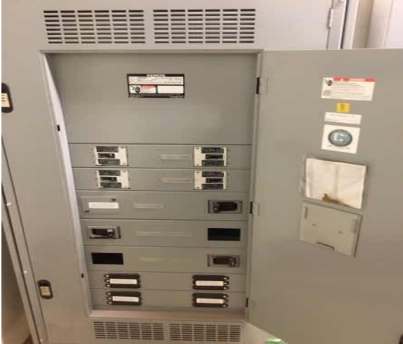
D5012 Low Tension Service & Dist.: - Panel Board
