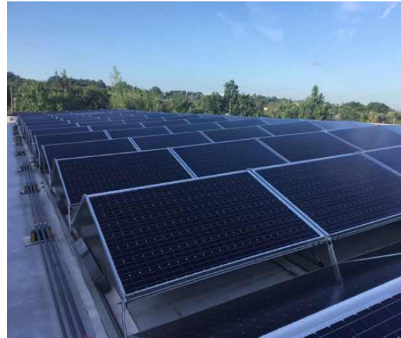
D3016 Solar Energy System:- Solar Panel
