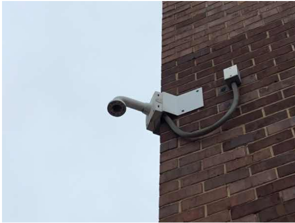
Damaged Surveillance Camera
