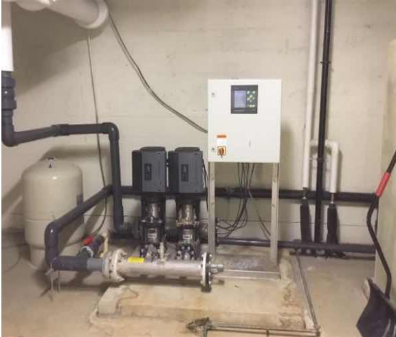
D2023 Domestic Water Supply Equipment:- Booster Pump
