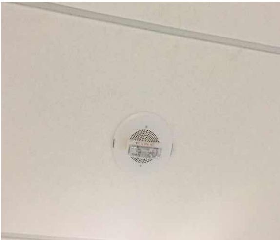
D5037 Fire Alarm Systems:- Speaker Strobe
