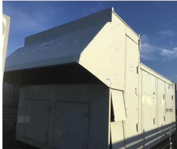
D3052 Package Units:- Rooftop Unit
