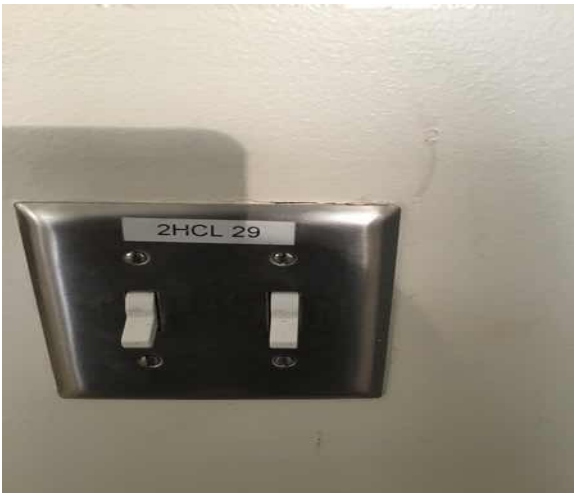
D5021 Branch Wiring Devices:- Switch
