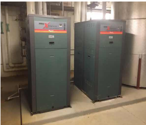
D2022 Hot Water Service:- Water Heaters
