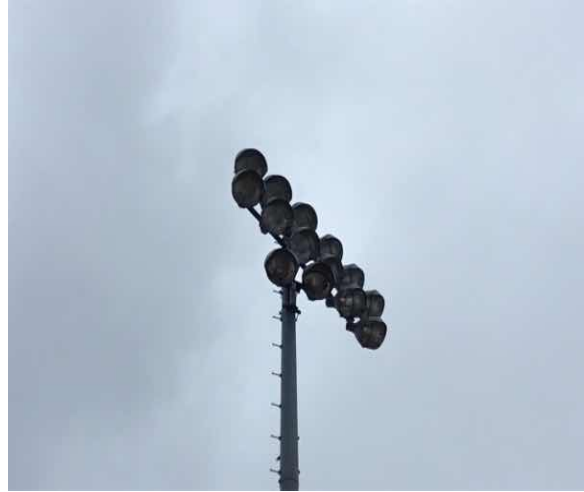
G4021 Fixtures & Transformers:- Stadium Lighting
