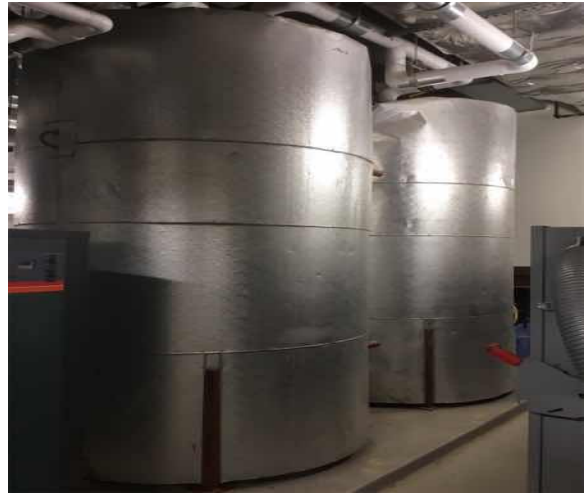
D2022 Hot Water Service:- Domestic Hot Water Storage Tanks
