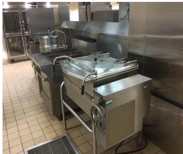
E1093 Food Service Equipment:- Kitchen Equipment
