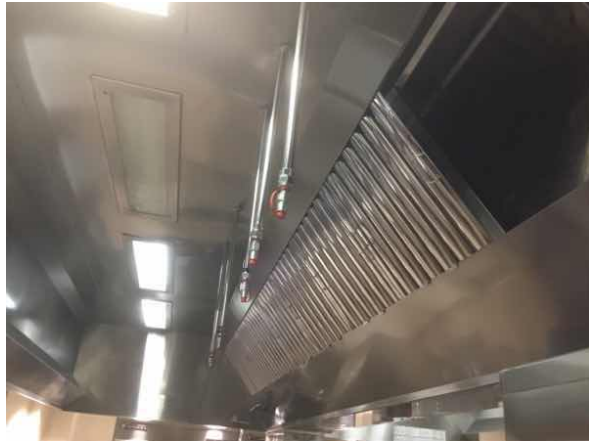
Kitchen Hood Sprinkler Nozzles
