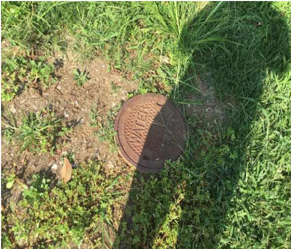
D2023 Domestic Water Supply Equipment:- Water Meter
