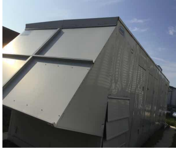
D3041 Air Distribution Systems:- Rooftop Unit
