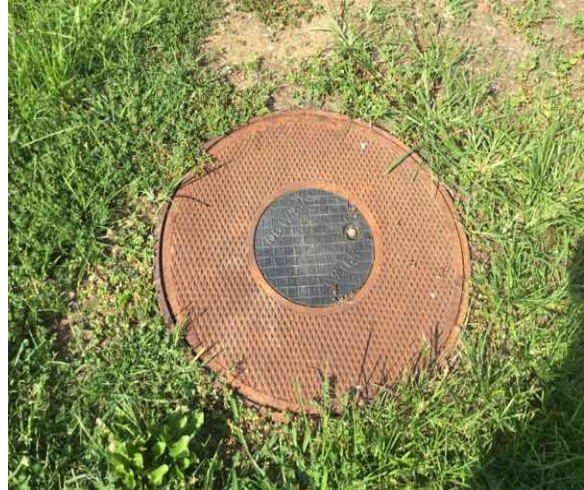
D2023 Domestic Water Supply Equipment:- Water Meter
