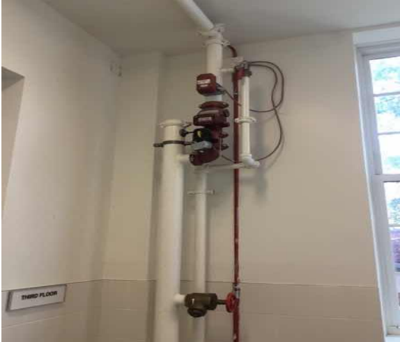
D4012 Sprinkler Pumping Equipment:- Fire Standpiping
