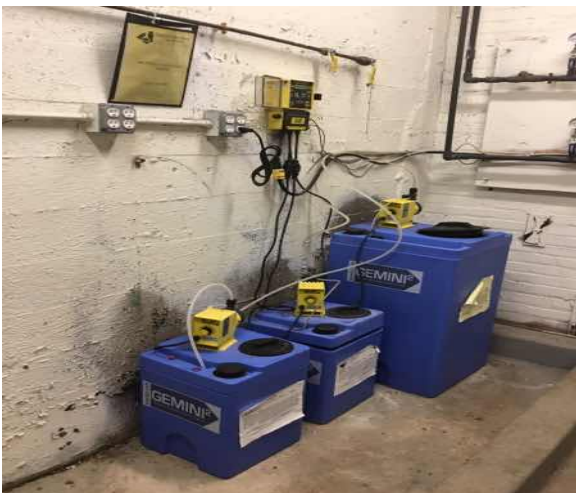
D2023 Domestic Water Supply Equipment:- Water Filtration System
