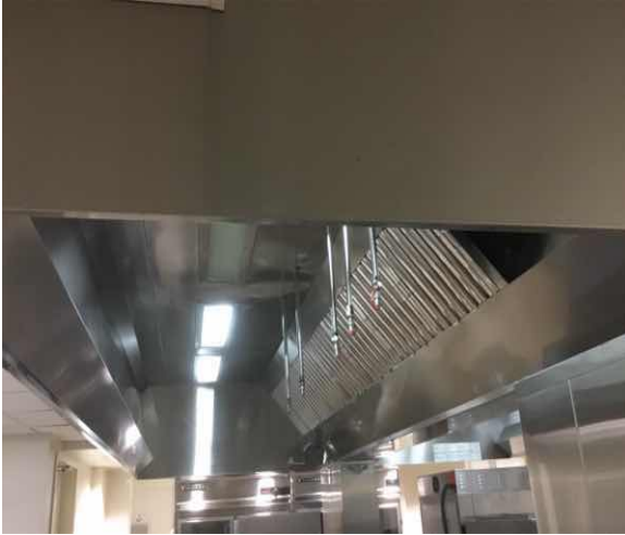
D3042 Exhaust Ventilation Systems:- View of Kitchen Exhaust Hood
