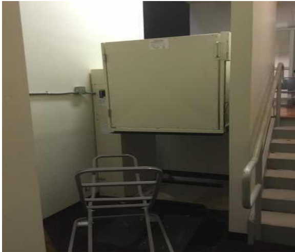
D1013 Lifts:- Wheel Chair Lift
