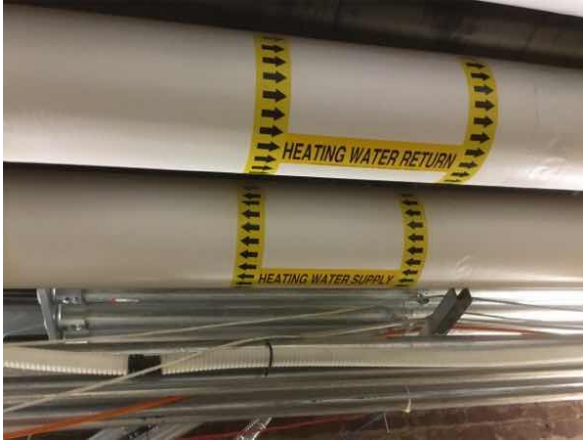
Heating Water Piping
