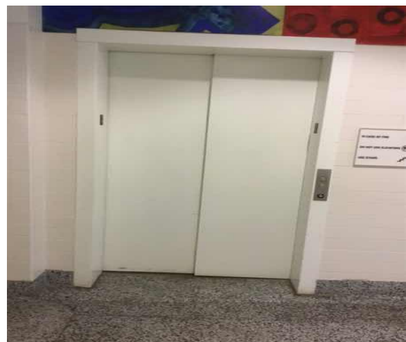
D1011 Passenger Elevators:- View of Elevators (x2)
