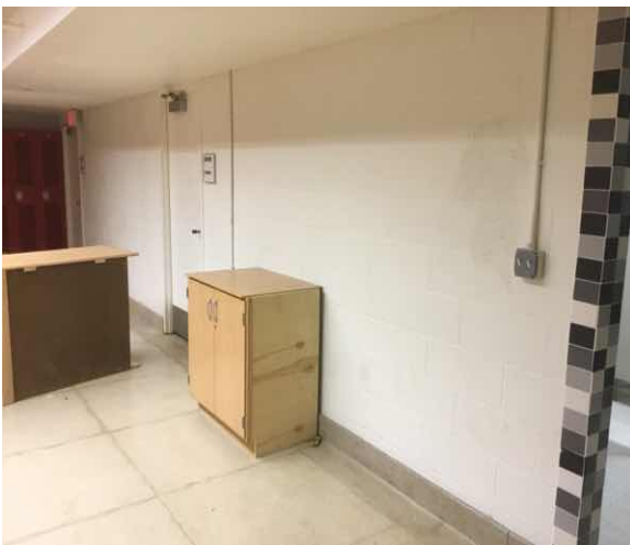
C3012 Wall Finishes to Interior Walls:- View of Concrete Block Interior Wall Finish
