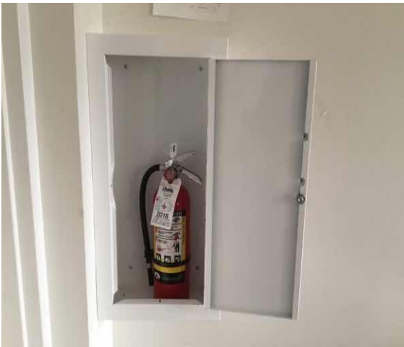
D4031 Fire Extinguishers:- Fire Extinguisher
