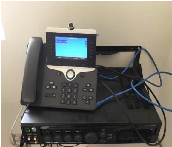
D5033 Telephone Systems:- Telephone
