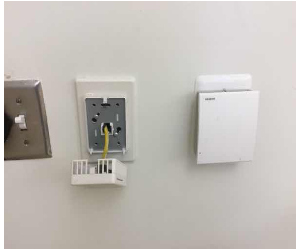
D3068 Building Automation Systems:- Detached Thermostat in Room 321
