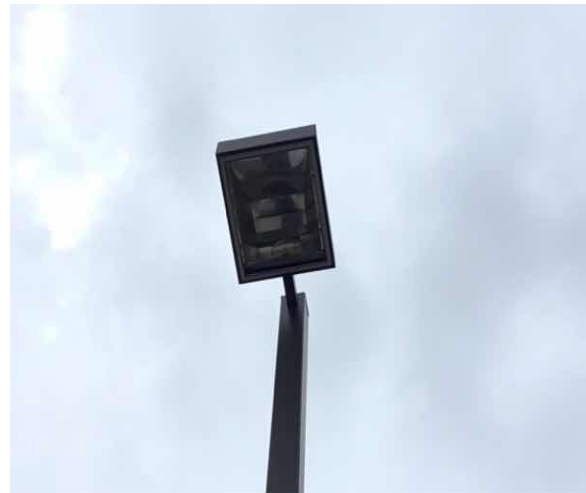
G4021 Fixtures & Transformers:- Site Lights
