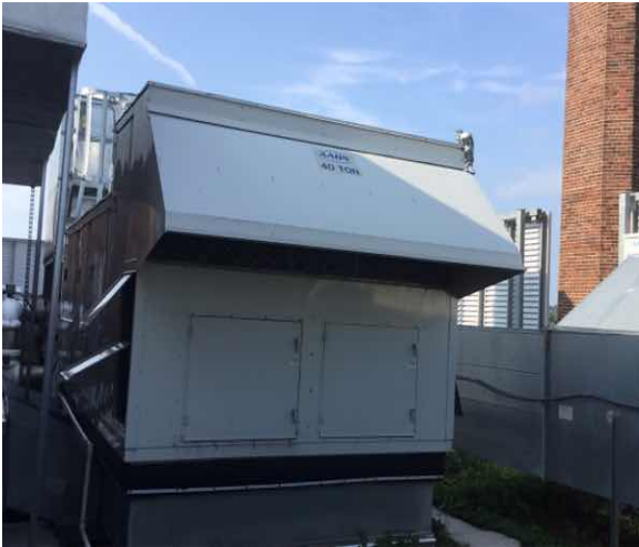
D3052 Package Units:- Rooftop Unit
