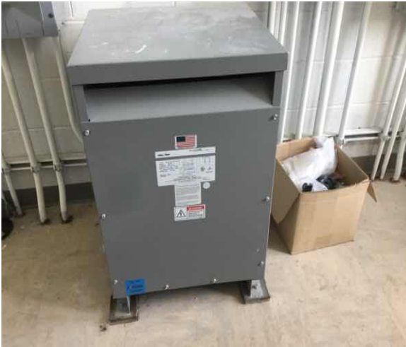
D5012 Low Tension Service & Dist.: - Transformer
