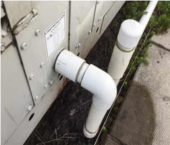
D3041 Air Distribution Systems:- Condensate piping leaking
