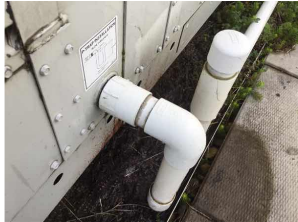
Condensate piping leaking
