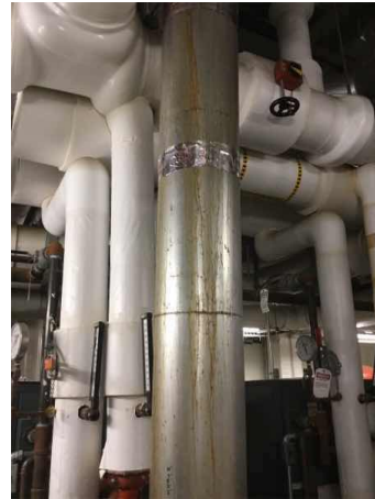
Flue Piping Leaking...Boiler 1
