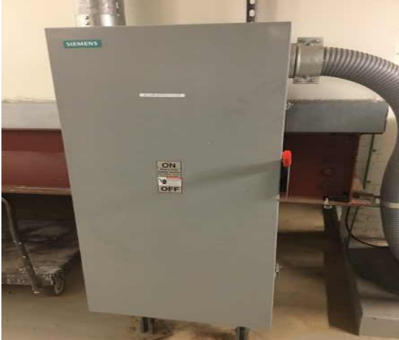
D5012 Low Tension Service & Dist.:- Disconnect
