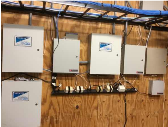
Access Control Panel
