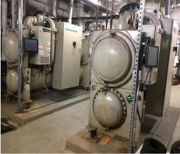
D3031 Chilled Water Systems:- Chillers
