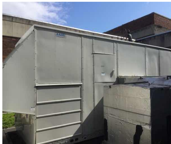
D3052 Package Units:- Rooftop Unit
