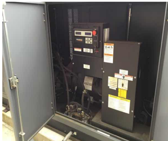
D5092 Emergency Light & Power Systems:- Generator
