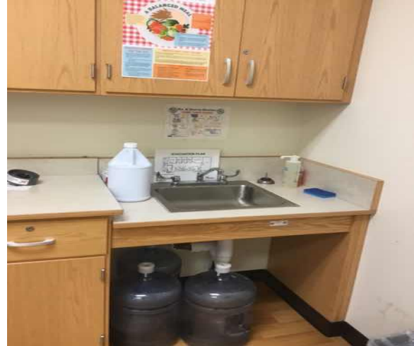
D2014 Sinks:- Classroom Sink
