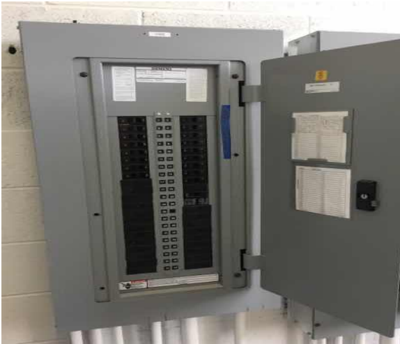
D5012 Low Tension Service & Dist.:- Panel Board
