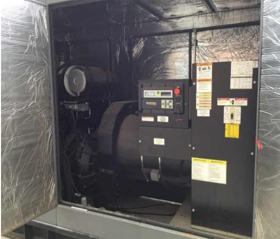
D5092 Emergency Light & Power Systems:- Generator
