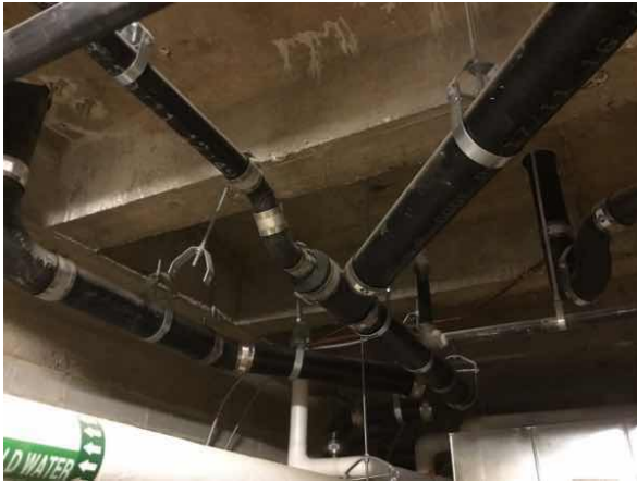
Sanitary Waste Piping
