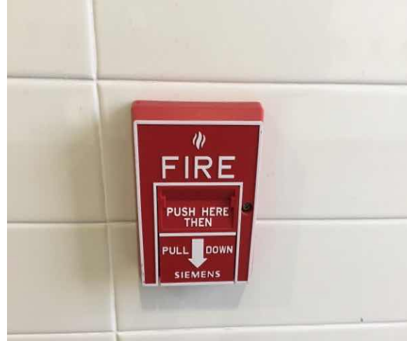
D5037 Fire Alarm Systems:- Pull Station
