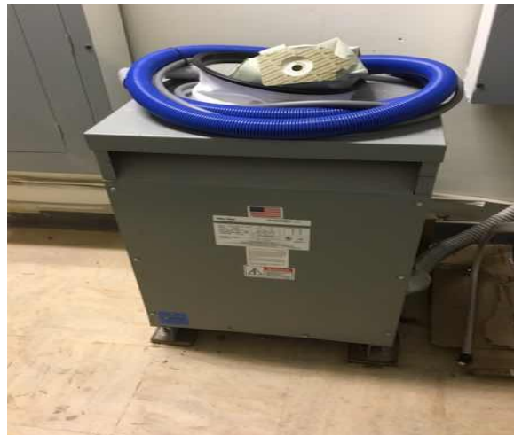
D5012 Low Tension Service & Dist.: - View of Secondary Transformer, Dry, 30 kVA
