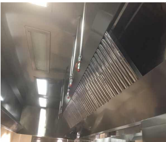
D4095 Hood & Duct Fire Protection:- Kitchen Hood Sprinkler Nozzles
