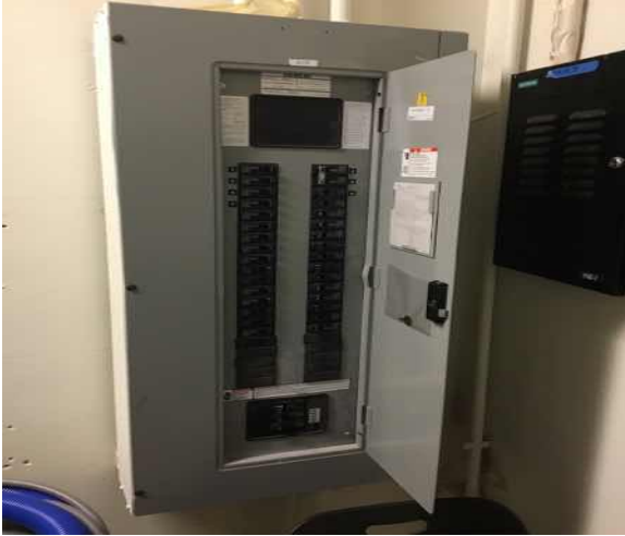
D5012 Low Tension Service & Dist.:- Panel Board
