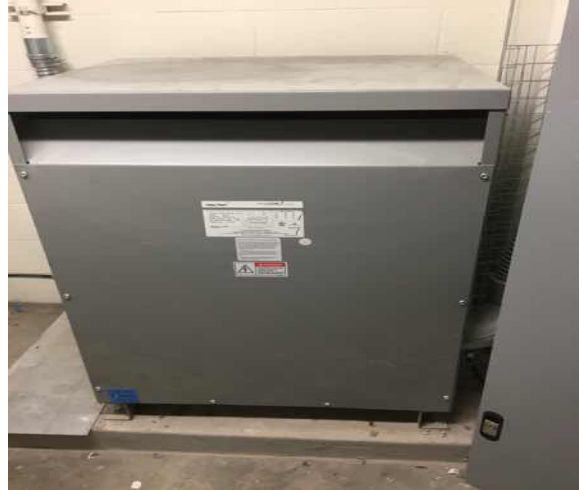
D5012 Low Tension Service & Dist.: - Transformer
