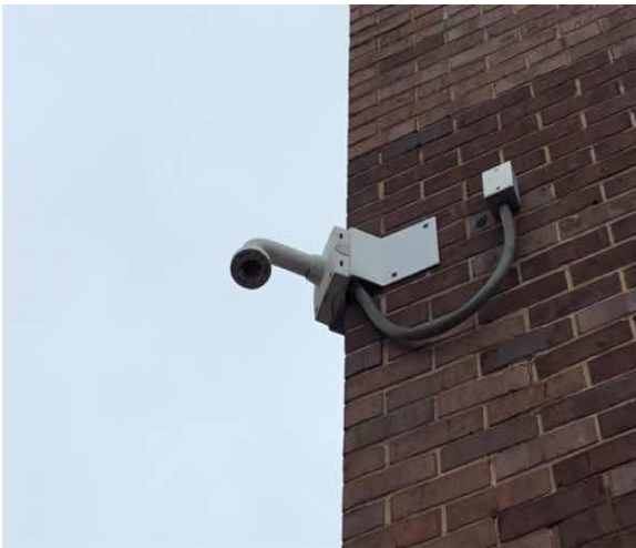
D5038 Security and Detection Systems:- Damaged Surveillance Camera
