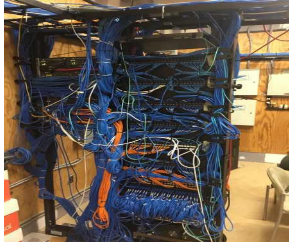
D5039 Local Area Networks:- LAN Rack
