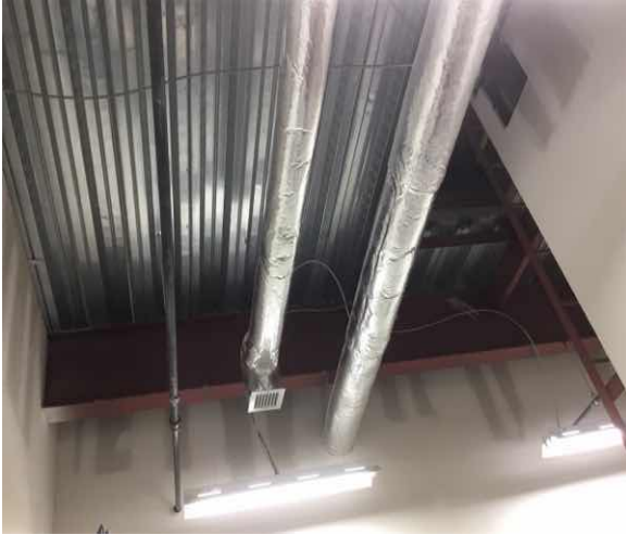
D3041 Air Distribution Systems:- Ductwork
