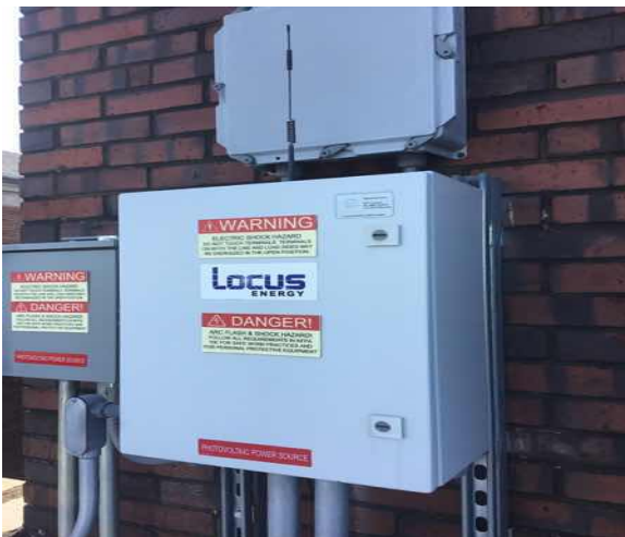
D3016 Solar Energy System:- Inverter Box
