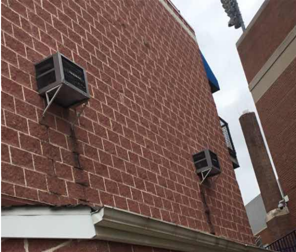
D3051 Terminal Self-Contained Units:- Window A/C Unit
