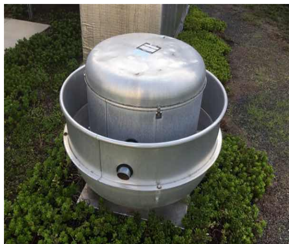
D3042 Exhaust Ventilation Systems:- Exhaust Fan
