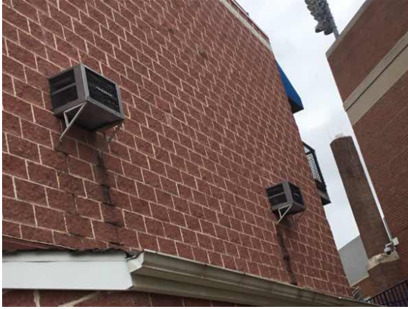
Window A/C Unit
