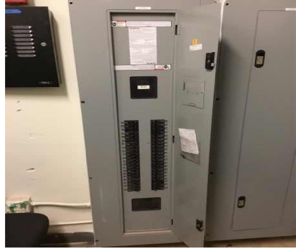
D5012 Low Tension Service & Dist.:- Panel Board
