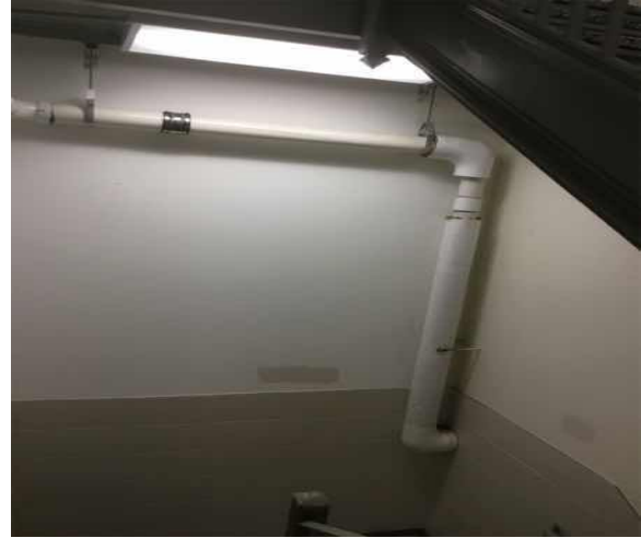
D2041 Pipe & Fittings:- Rain Drainage Piping
