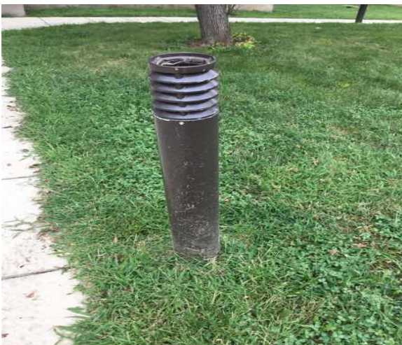
G4021 Fixtures & Transformers:- Bollard Light
