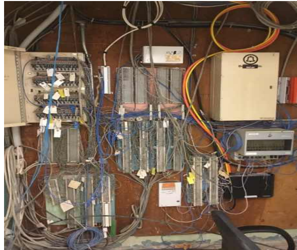
D5033 Telephone Systems:- Telephone
