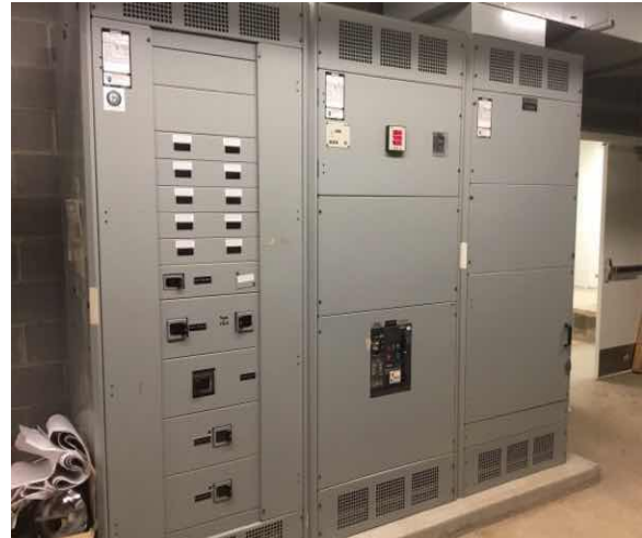
D5012 Low Tension Service & Dist.:- Main Switchgear
