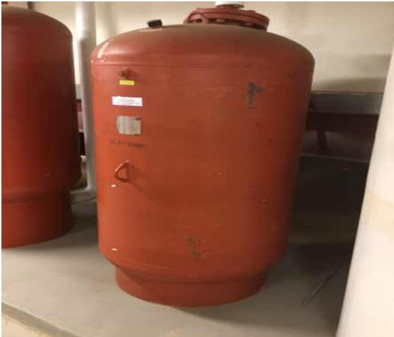
D3022 Boiler Room Piping & Specialties:- Expansion Tank
