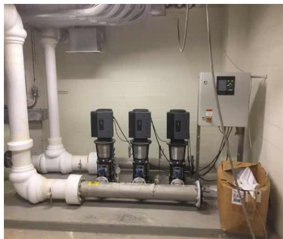
D2023 Domestic Water Supply Equipment:- Booster Pump
