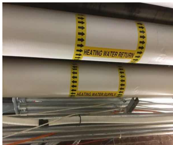
D3022 Boiler Room Piping & Specialties:- Heating Water Piping
