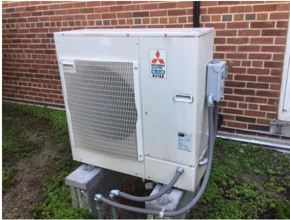
Air Cooled Condenser
