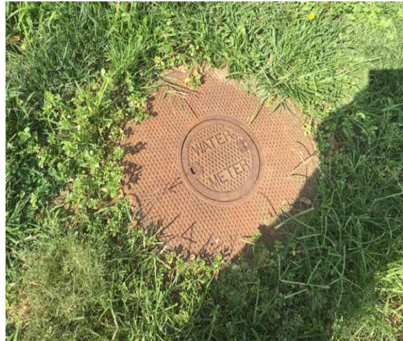
D2023 Domestic Water Supply Equipment:- Water Meter
