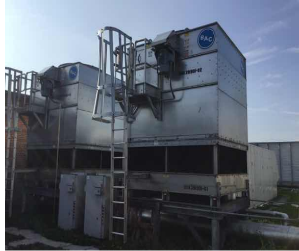
D3031 Chilled Water Systems:- Cooling Towers
