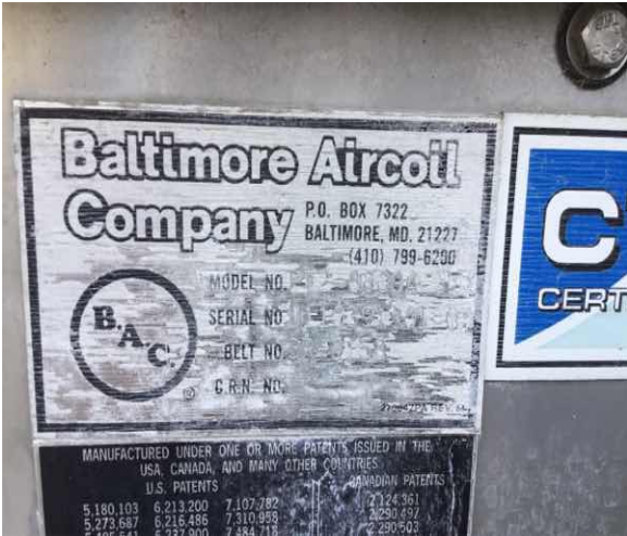
D3031 Chilled Water Systems:- View of Cooling Tower, 250 Ton (x2)
