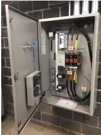
Automatic Transfer Switch
