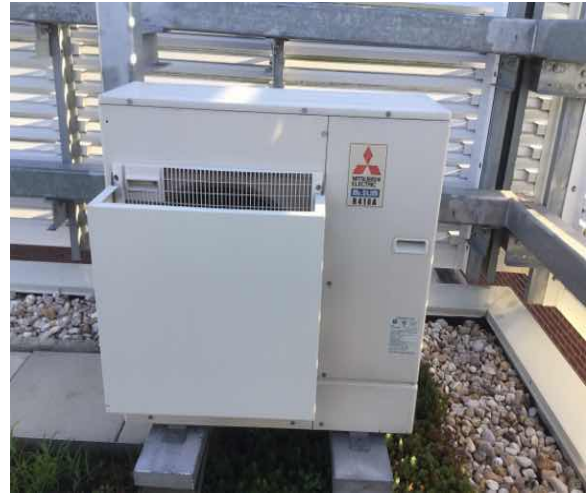
D3032 Direct Expansion Systems:- Air-Cooled Condenser
