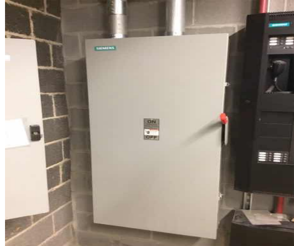
D5012 Low Tension Service & Dist.:- Disconnect
