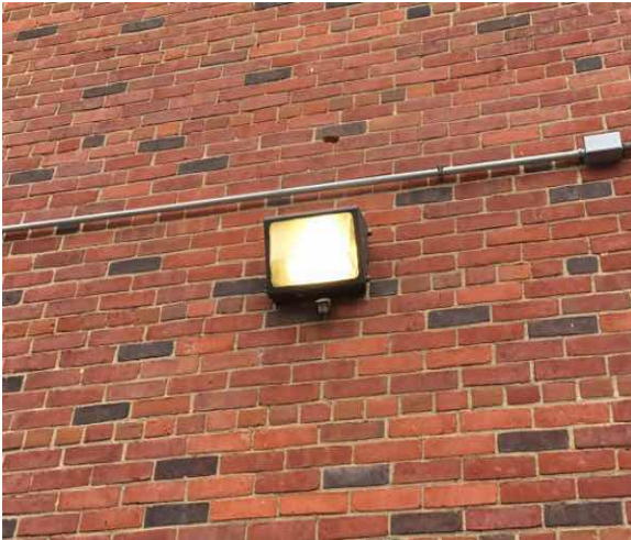
D5022 Lighting Equipment:- Flood Lights
