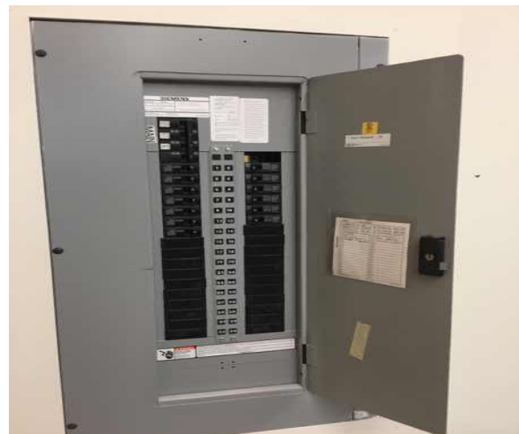
D5012 Low Tension Service & Dist.:- Panel Board
