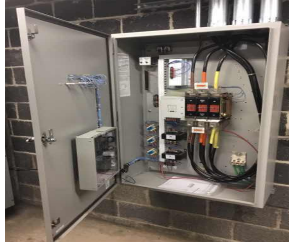
D5012 Low Tension Service & Dist.:- Automatic Transfer Switch
