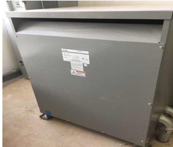
D5012 Low Tension Service & Dist.: - Transformer
