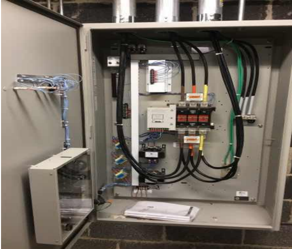
D5012 Low Tension Service & Dist.:- Automatic Transfer Switch
