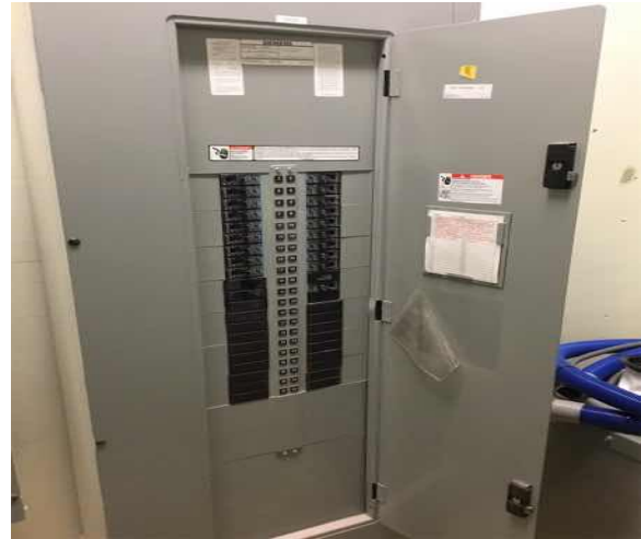
D5012 Low Tension Service & Dist.:- Panel Board
