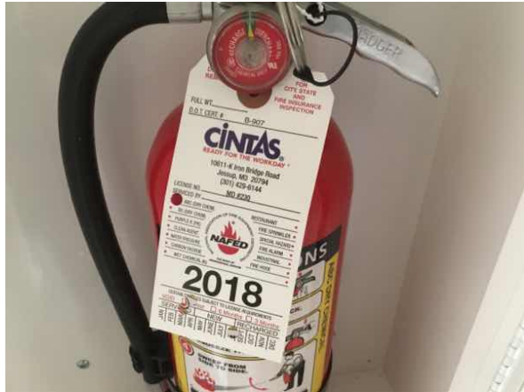
Fire Extinguisher Certification Tag
