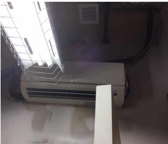
D3041 Air Distribution Systems:- Split A/C System Indoor Unit
