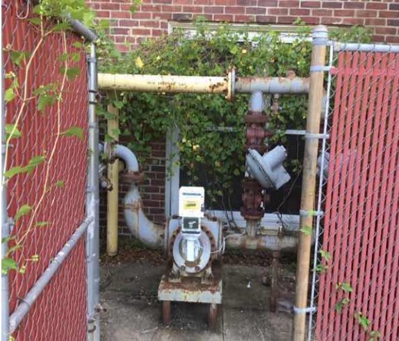
D3067 Energy Monitoring & Control:- Gas Meter
