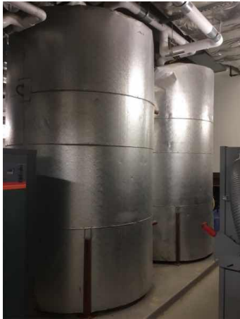
Domestic Hot Water Storage Tanks
