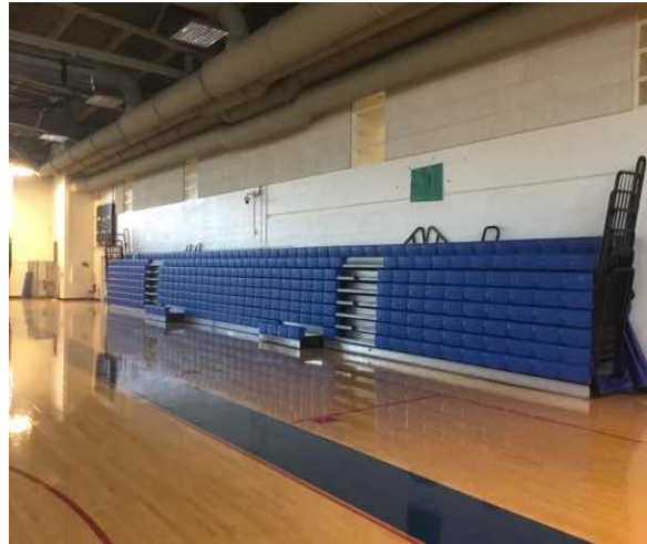
E2015 Fixed Multiple Seating:- View of Gymnasium Seatings
