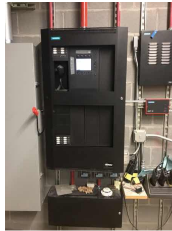
Fire Alarm Panel
