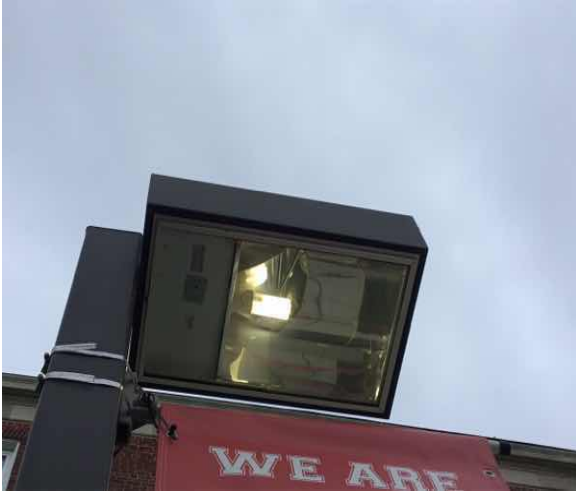
G4021 Fixtures & Transformers:- Site Lights
