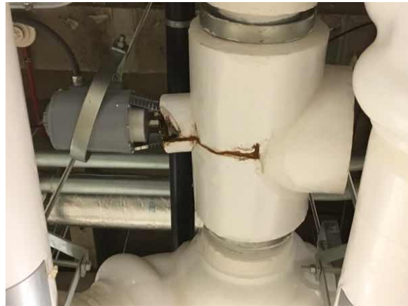
Cracked Chilled Water Piping at a Valve Controller- Leaking
