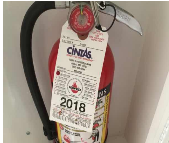
D4031 Fire Extinguishers:- Fire Extinguisher Certification Tag
