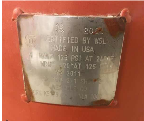
D3022 Boiler Room Piping & Specialties:- View of Expansion Tank, 400 Gal
