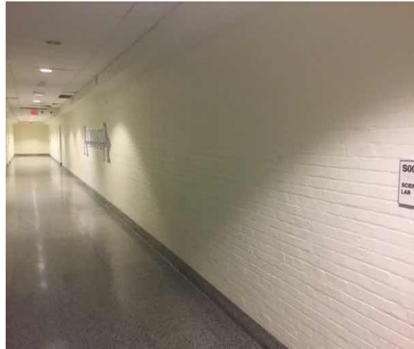
C3012 Wall Finishes to Interior Walls:- View of Clay Brick Interior Wall Finish
