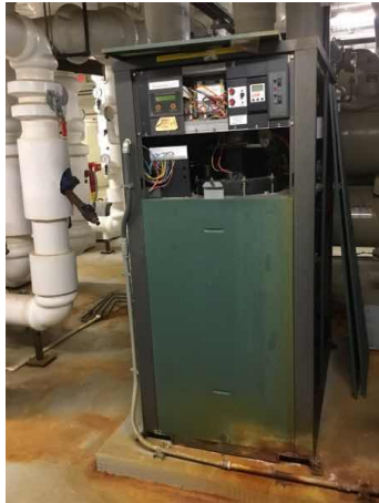
Boiler 3...not Working
