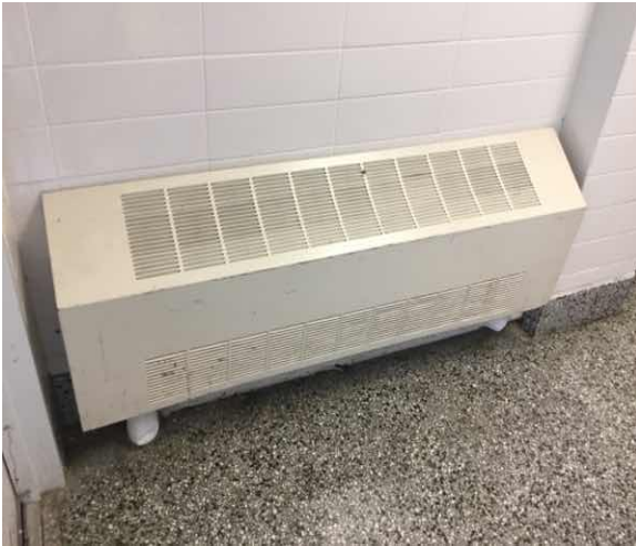
D3044 Hot Water Distribution:- Hydronic Heater
