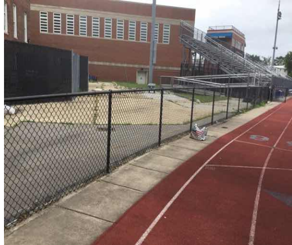
G2041 Fences & Gates:- View of 4' Chain Link Fence
