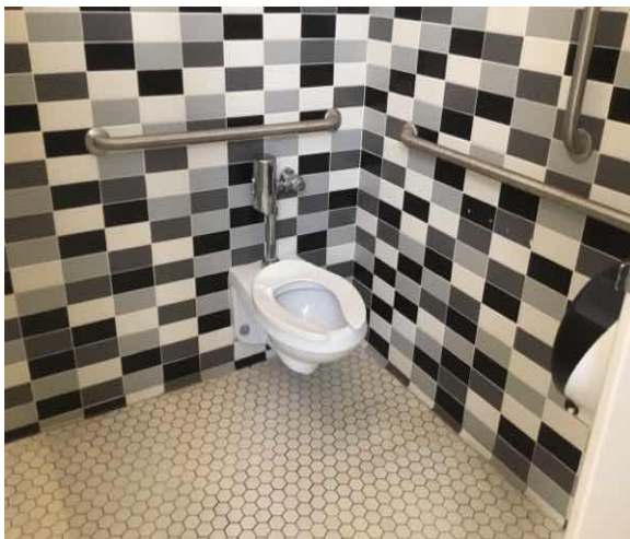
D2010.0 Water_Fixtures:- Toilet Seat
