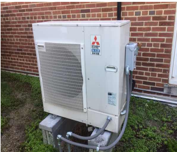
D3032 Direct Expansion Systems:- Air Cooled Condenser
