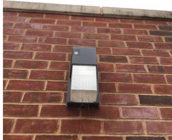
D5022 Lighting Equipment:- Exterior Lights
