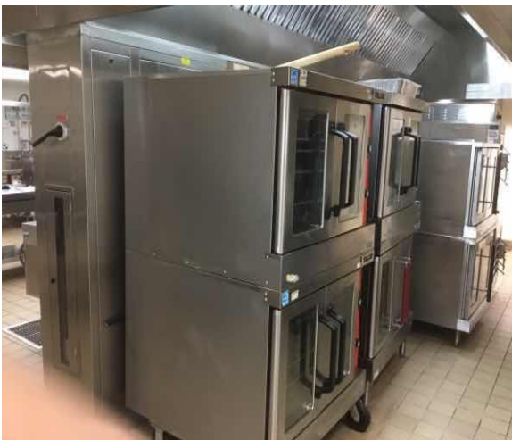
E1093 Food Service Equipment:- Kitchen Equipment
