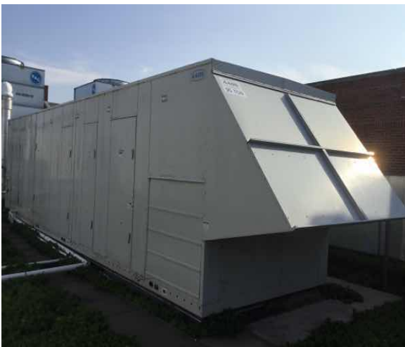
D3052 Package Units:- Rooftop Unit
