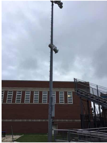
Football Site Light Pole
