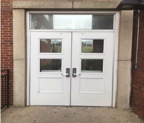
B2031 Glazed Doors & Entrances:- View of Steel w/ Safety Glass Exterior Door
