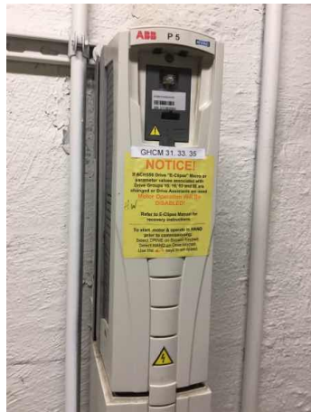
Broken VFD Controller of Hot Water Pump 5
