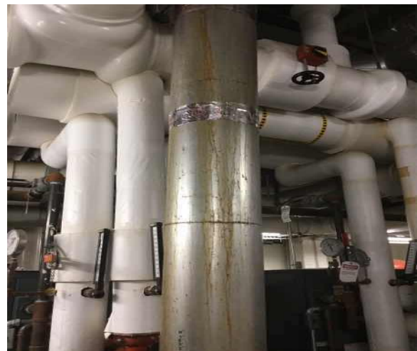
D3021 Boilers:- Flue Piping Leaking...Boiler 1
