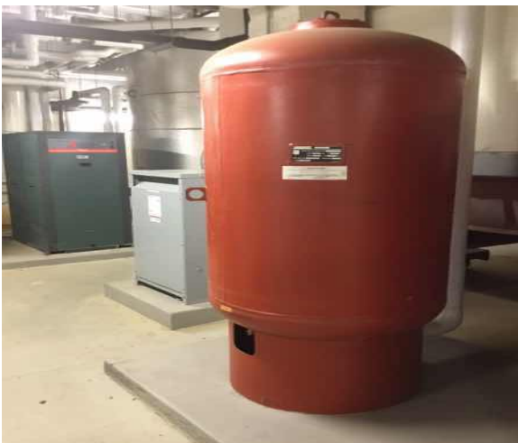
D3022 Boiler Room Piping & Specialties:- Expansion Tank
