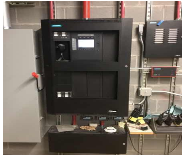
D5037 Fire Alarm Systems:- Fire Alarm Panel
