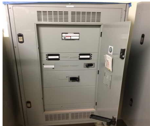
D5012 Low Tension Service & Dist.:- Panel Board
