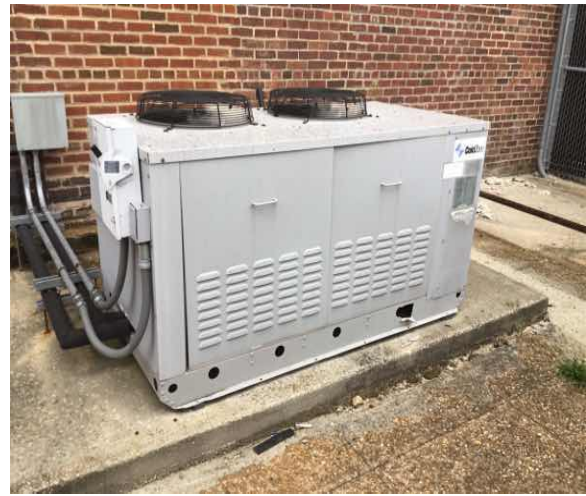
D3032 Direct Expansion Systems:- Condensing Unit
