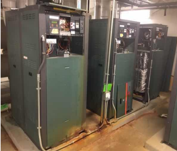
D3021 Boilers:- Boilers
