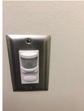
Occupancy Sensor Receptacle
