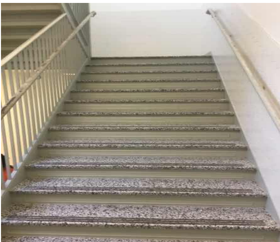
C2011 Regular Stairs:- View of Concrete Filled Metal Pan Type Interior Stair
