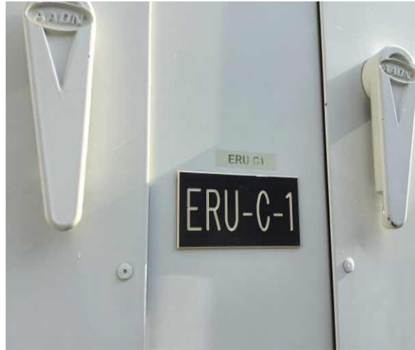
D3041 Air Distribution Systems:- View of Energy Recovery Unit, 27,500 CFM
