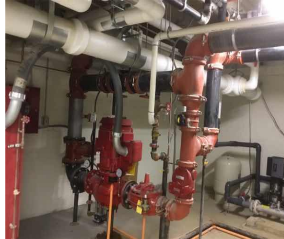
D4012 Sprinkler Pumping Equipment:- Sprinkler System
