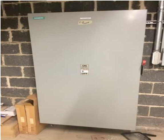
D5012 Low Tension Service & Dist.:- Disconnect
