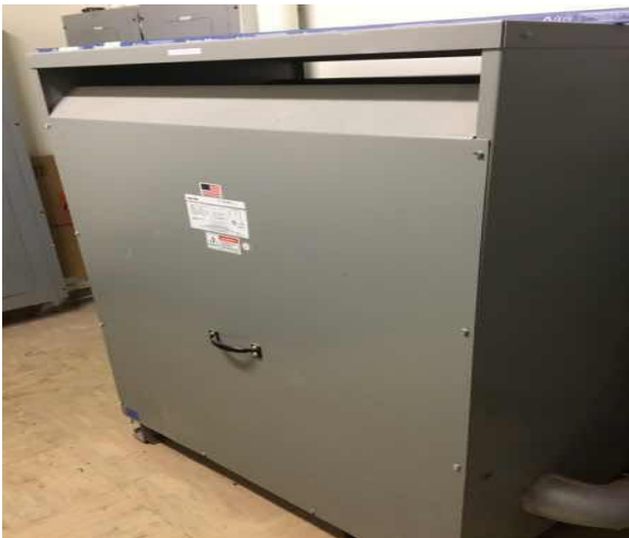
D5012 Low Tension Service & Dist.: - Transformer
