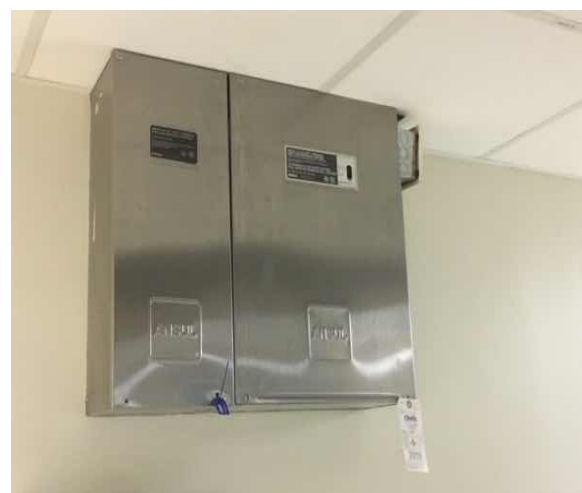
D4095 Hood & Duct Fire Protection:- Ansul System
