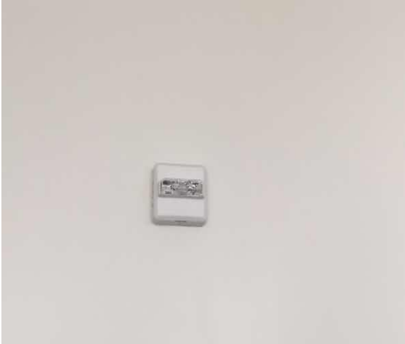
D5037 Fire Alarm Systems:- Strobe
