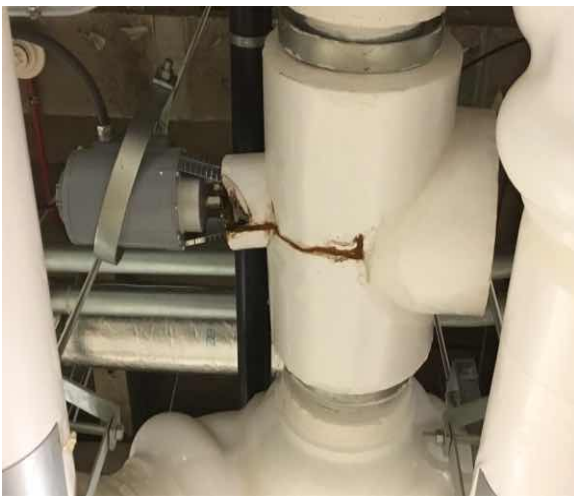
D3045 Chilled Water Distribution:- Cracked Chilled Water Piping at a Valve Controller- Leakng
