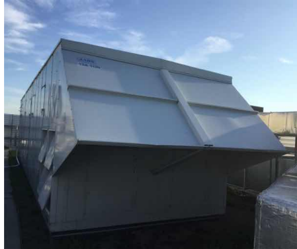
D3052 Package Units:- Rooftop Unit
