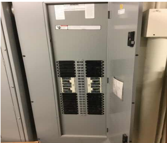
D5012 Low Tension Service & Dist.:- Panel Board
