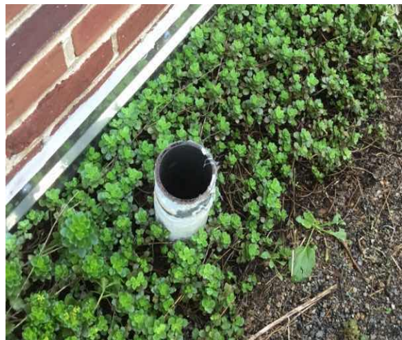
D2031 Waste Piping:- Vent
