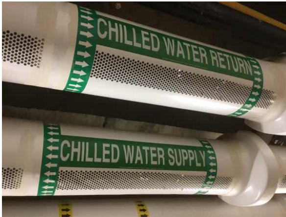
Chilled Water Piping
