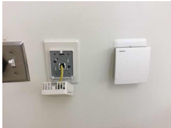
Detached Thermostat in Room 321
