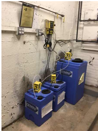
Water Filtration System
