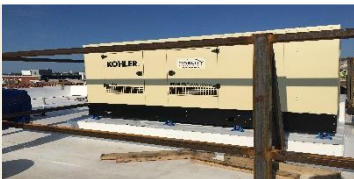
View of mechanical unit for air conditioning in place on roof.
