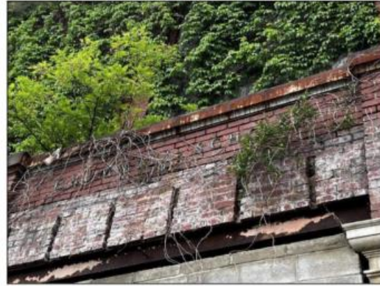
Figure 2: South entrance, missing cornice. Note lettering.
