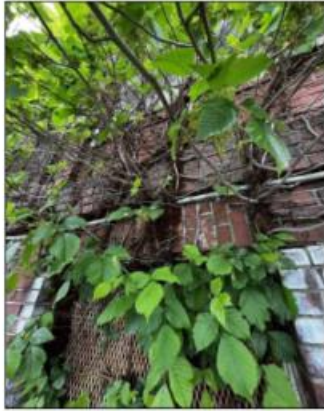
Figure 1: Vegetation growing into the masonry.
