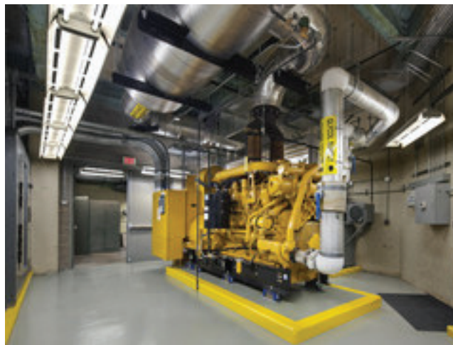
Figure 7.8 Sample Emergency/Standby Generator
