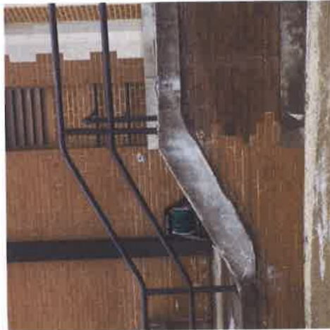
Figure 4 – Concrete distress at existing stairs.
