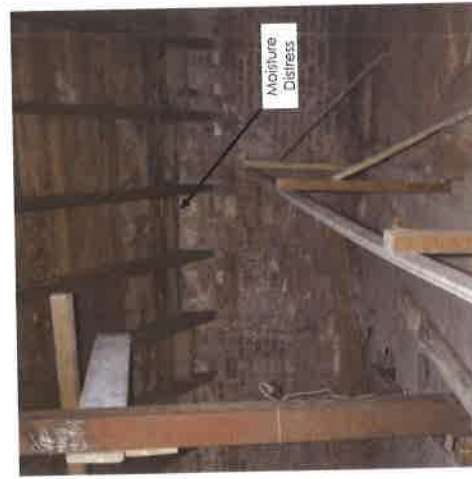
Figure 8 – Moisture distress at rafter bearing pockets slab.
