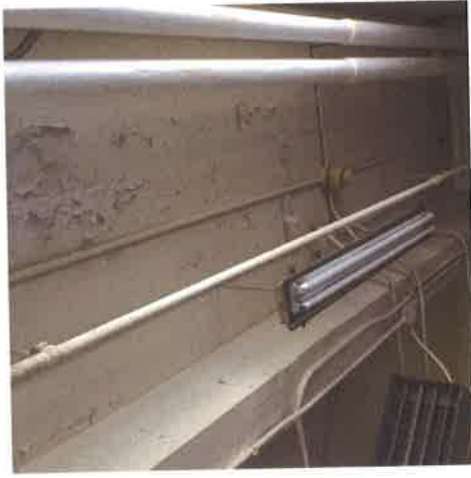
Figure 11 – Peeling paint in basement of 1930's connector.
