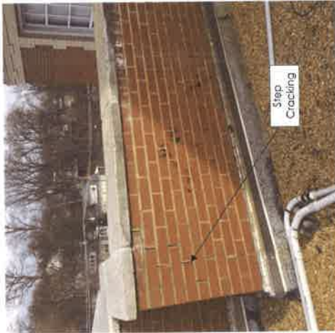
Figure 3 – Parapet distress at northwest corner of 1980's bldg.
