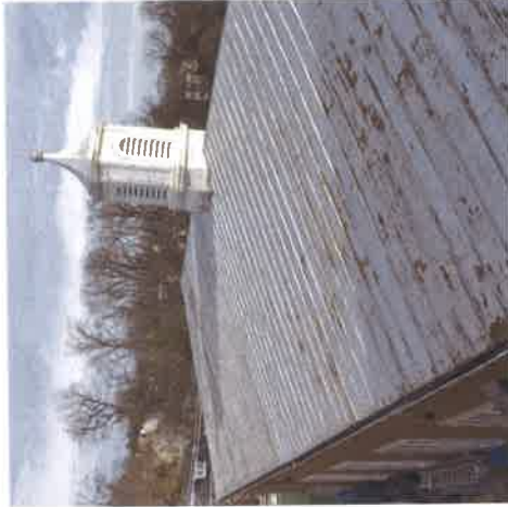
Figure 6 – 1930's building roof distress.
