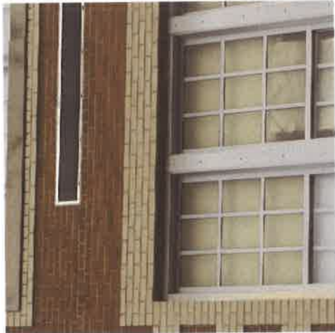
Figure 1 – Step crack at left side of window extending right.
