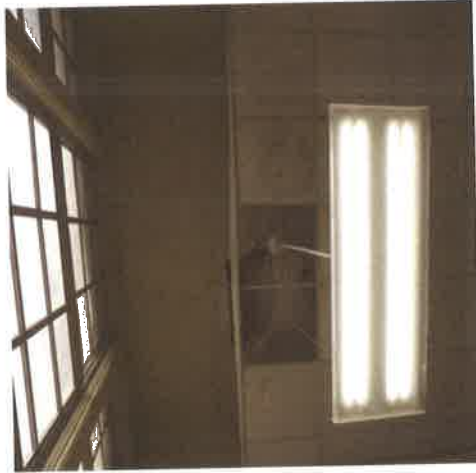
Figure 9 – 1911 Bldg: exposed rebar at underside of stairwell slab.
