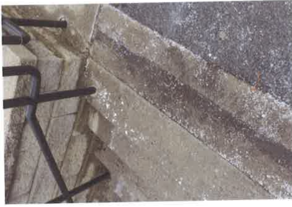
Badly clogged trench drain at top of site stairs
