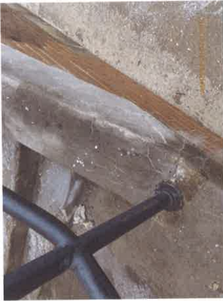
Rear pedestrian stamps and ramp showing cracking and deterioration
