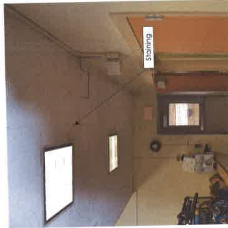
Figure 10 – Moisture distress at underside of second floor.
