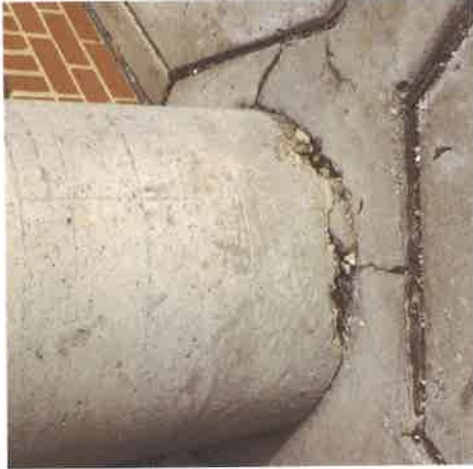
Figure 5 – Concrete distress at base of 1980's building column.
