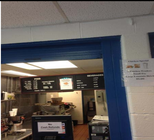
23. Lead-Based Paint on Blue Metal Window Casing Located in Snack Bar – Rollup. Reading No. 45.
