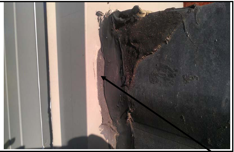
2. Roof by Hatch – View of Dark Gray Perimeter Caulk (ACM), Samples # R05-R06
