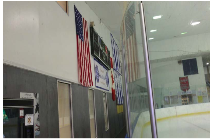
20. Assumed Asbestos-Containing Mastics Behind Scoreboard. Not Sampled.
