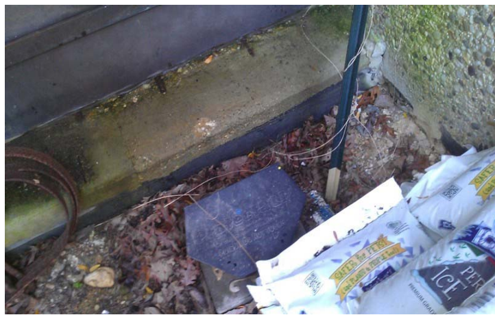
8. East Side of Building – View of Exterior Felt Paper Waterproofing (ACM), Samples #E07-E08
