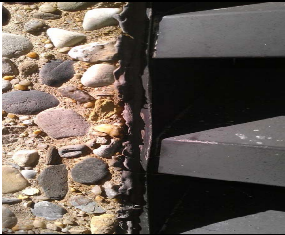
7. East Side of Building – View of Exterior Black Caulk (ACM) along Window & HVAC Vent, Samples #E05-E06
