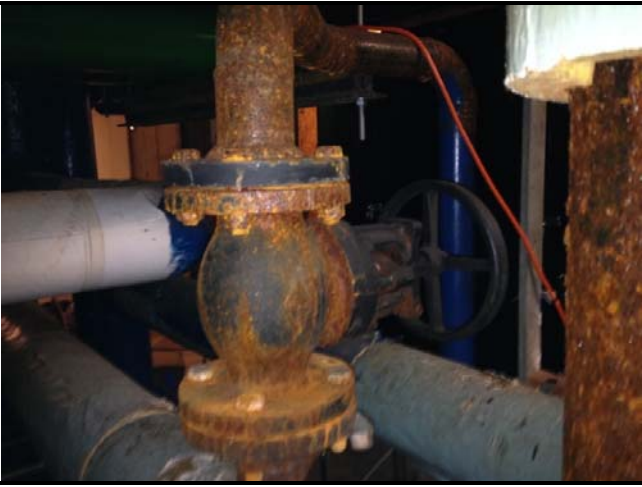
19. Assumed Asbestos-Containing Pipe Flange Gaskets in Heating and Plumbing Systems. Not Sampled.
