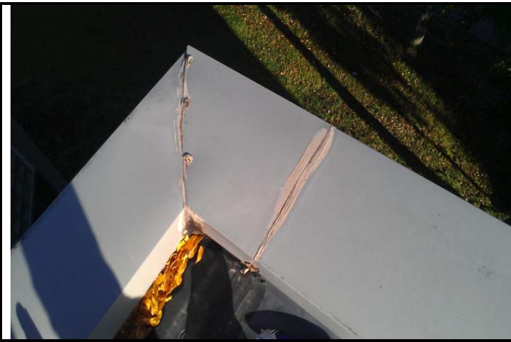
1. Roof by Hatch – View of Tan Caulk along Metal Coping (ACM), Samples # R01-R02
