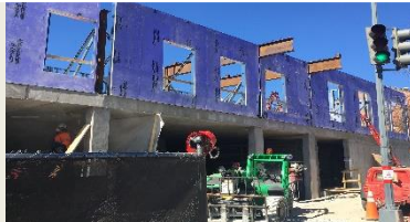
View From 14 th St. Structural Steel Reinforcement to Load Bearing Wall Connection
