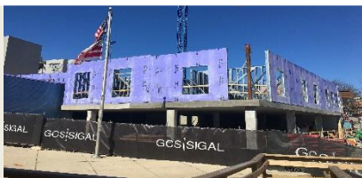
View From from Chapin St Load Bearing Wall Sequence begins from West Elevation
