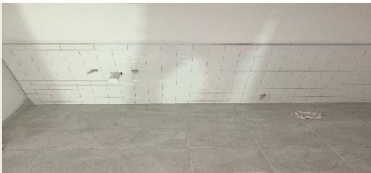
View of Ceramic wall tiles are scheduled to be installed in the 1st and 2nd floor bathrooms.
