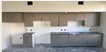
View of Cabinetry is scheduled to be installed on 2nd and 3rd floor levels.
