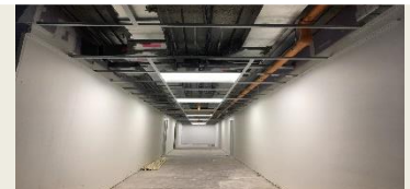
View of Ceiling grid install completed on First and Second Floor Levels.
